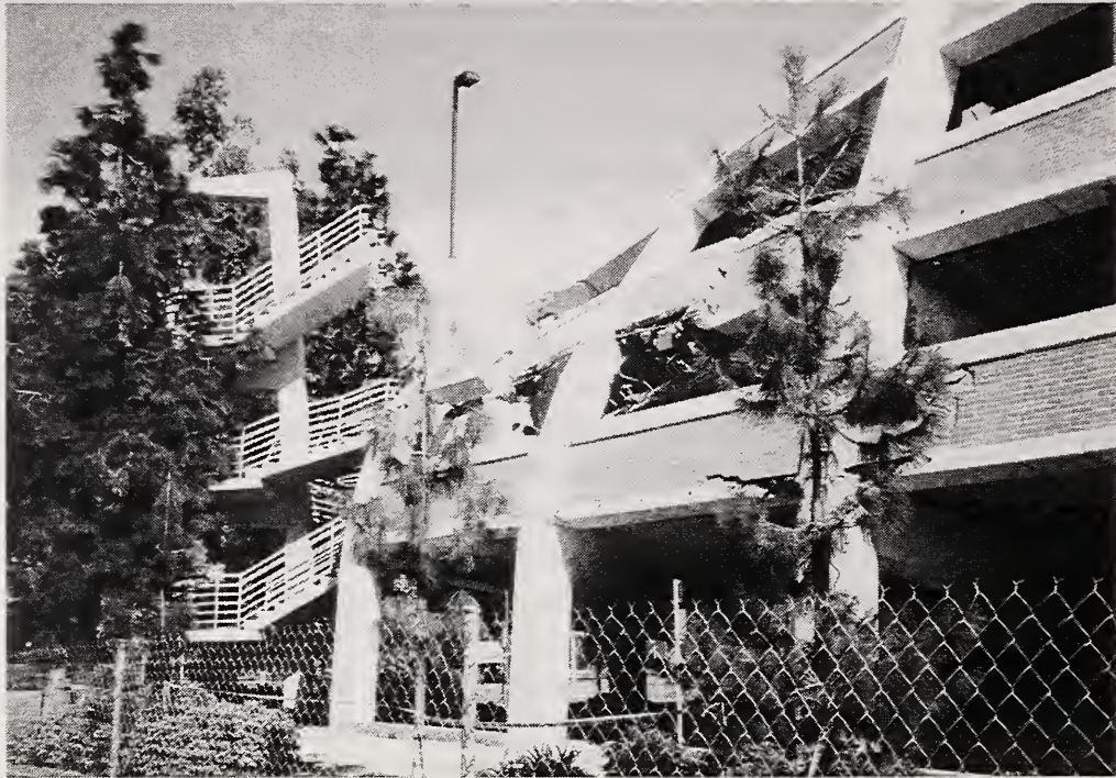
Figure 3.60 The three-year old four-level parking garage at the Northridge campus of California State University partially collapsed in the earthquake. The collapse apparently started at the interior, causing the exterior walls to be pulled in to the middle of the structure. Precast concrete "trees" were connected to form a moment-resisting frame at the exterior of the structure.
