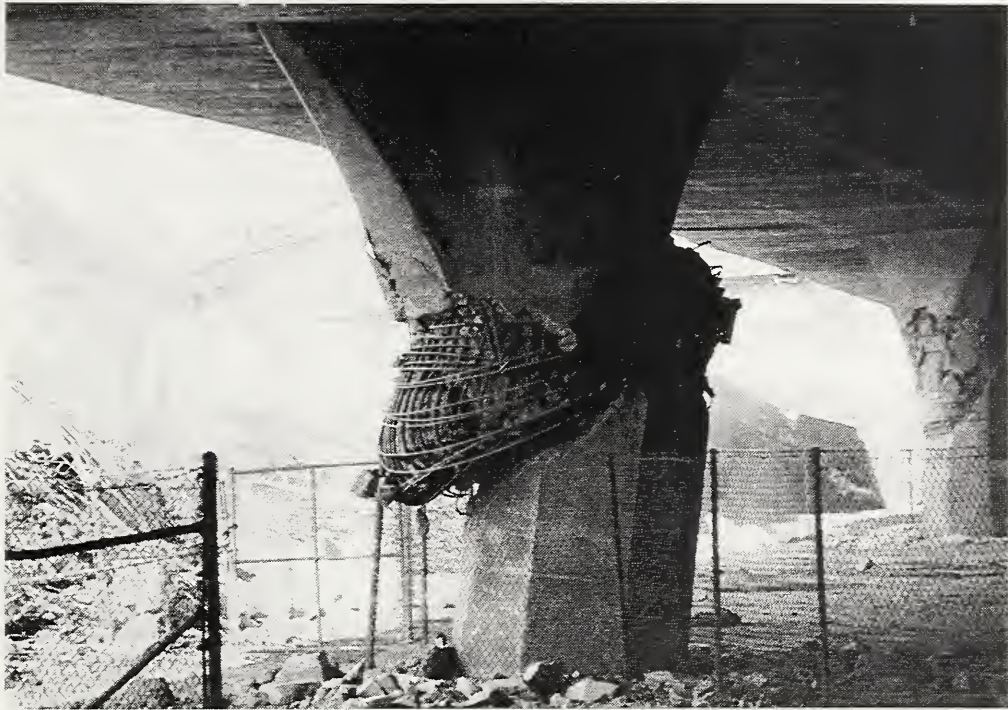
Figure 4.21 Damage to a pier of the SR118 Mission-Gothic Undercrossing, looking to the northwest at the southernmost pier of Bent 3 of the westbound bridge.
