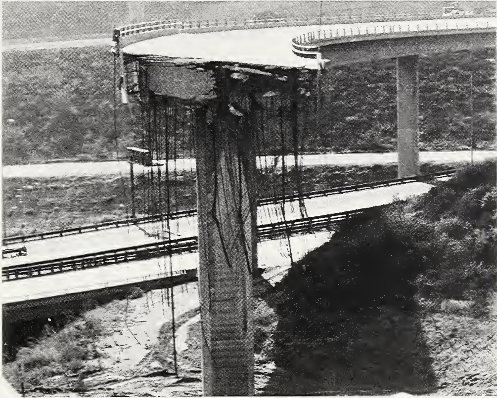
Figure 4.15 View of the flexural failure at Pier 3 of the SR14/I5 North Connector Overcrossing, looking to the south
