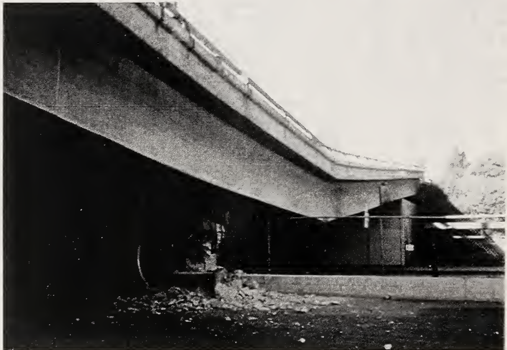
Figure 4.44 View of collapsed span of I10 over Fairfax Ave.; note rotation of girder over Pier 2 (Courtesy of EERC)
