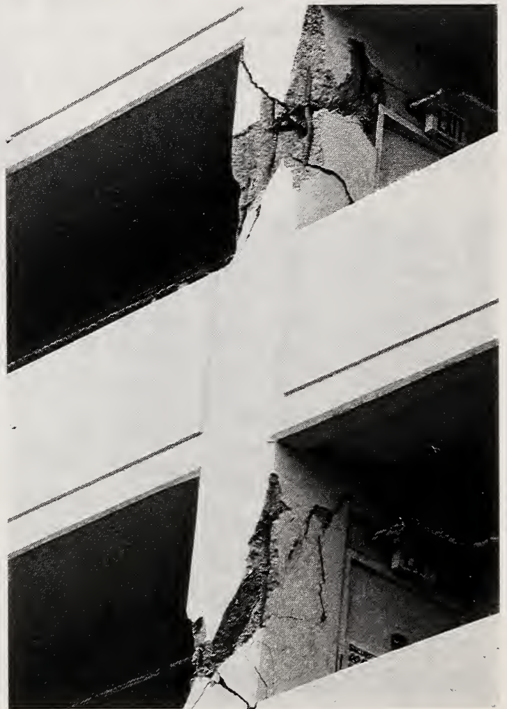
Figure 3.15 A closer view of the failed columns at the back of Champagne Towers shows minimal transverse reinforcement.
