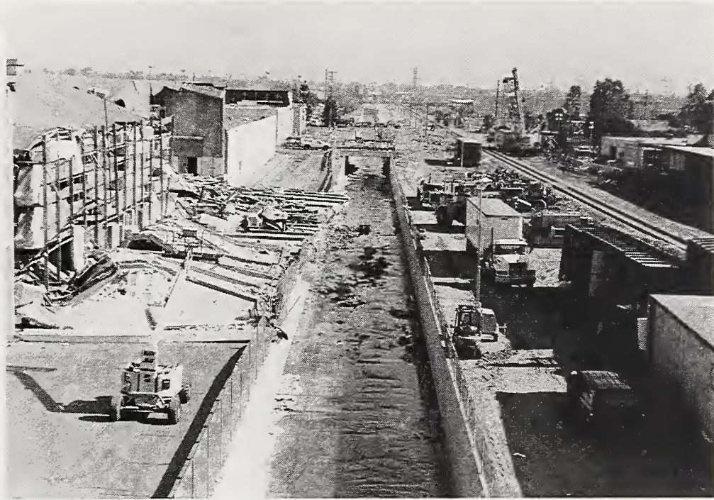
Figure 3.33 The south wall of the concrete tilt-up Levitz furniture store/warehouse south of the Northridge Fashion Center fell away from the building into the alley and stream channel. The damaged roof was being supported by the racks of furniture. On the south side of the stream channel a freight train derailed during the earthquake. That clean-up effort was still underway three days after the quake.
