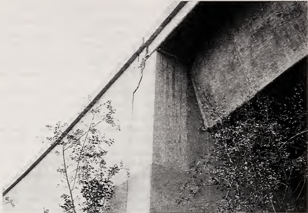
Figure 4.57 Close-up of abutment wall cracking at the east end of the ramp connecting eastbound SR118 with northbound I210
