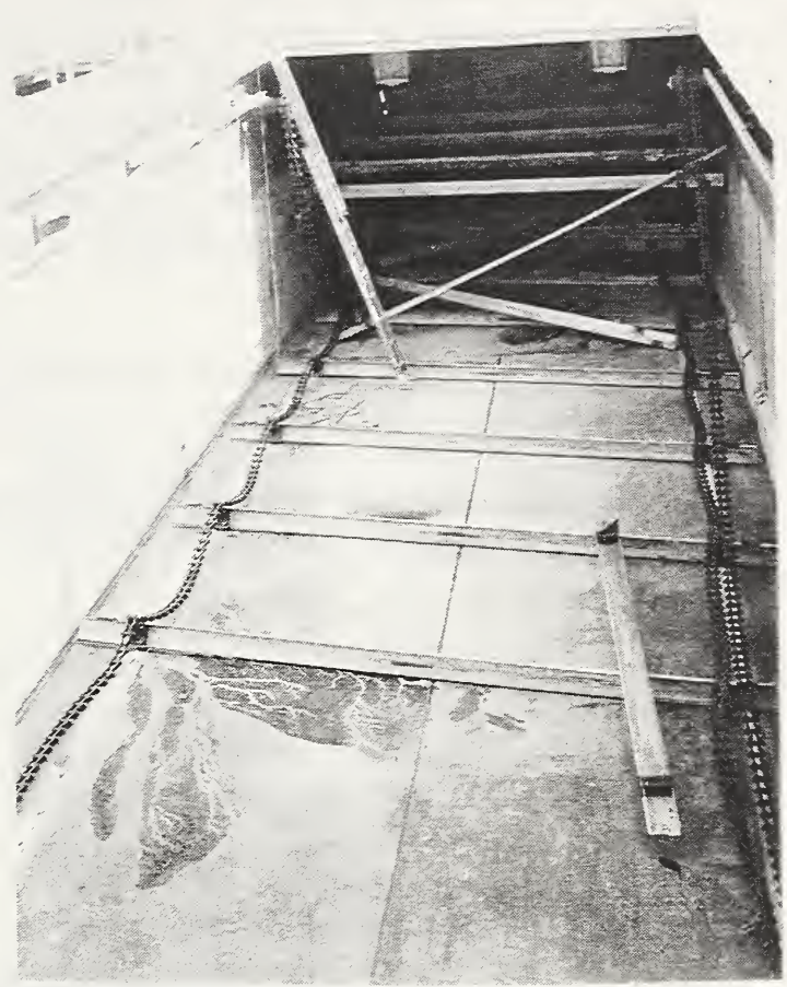
Figure 5.7 A damaged sludge scraper in a clarifier tank at the Tillman Water Reclamation Plant.
