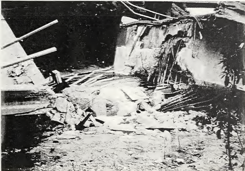
Figure 4.16 View of crushed Pier 2 and the hinge near Pier 2 (Courtesy EERC)
