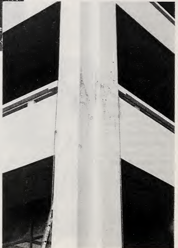
Figure 3.54 The cracked beam-column joints between the first and second stories of the Trans World Bank building were repaired using epoxy injection.
