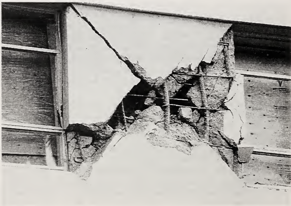
Figure 3.24 The transverse reinforcement in the St. John's hospital window piers was spaced at about 150-200 mm on center with 90° hooks at the ends, typical for construction of its age (about 50 years old).
