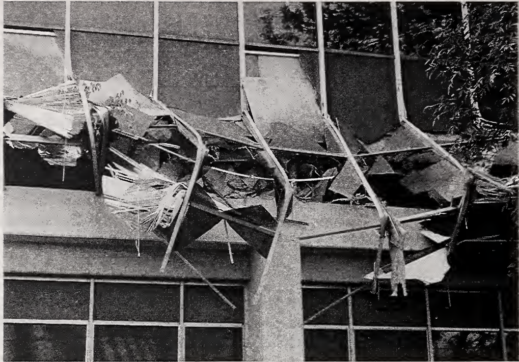
Figure 3.41 The second story of the concrete frame Kaiser Permanente office building on Balboa Avenue in Northridge completely collapsed. The first story was relatively undamaged, suggesting it was far stiffer than the story above.
