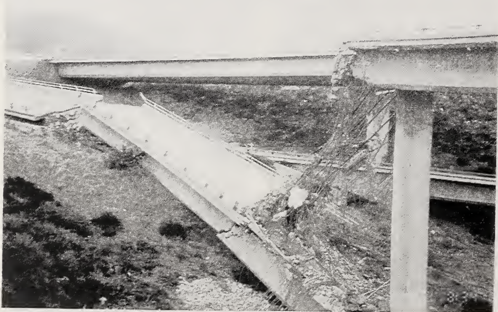
Figure 4.14 Collapsed portion of the SR14/I5 North Connector Overcrossing, looking east.. Pier 2 was at the left, near the broken hinge on the ground (Courtesy of EERC)
