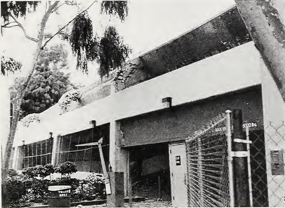
Figure 3.62 The cast-in-place concrete parking garage at the Kaiser Permanente Hospital complex in West Los Angeles collapsed in on itself. The moment frame that provided lateral resistance on the south face of the structure could not resist the out-of-plane forces apparently caused by the collapse of interior elements.
