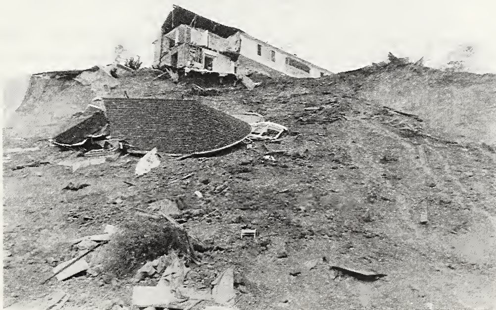
Figure 2.8 A landslide along the Pacific Coast Highway north of Santa Monica undermined the foundation of a house at the crest of the slope, bringing a portion of the house down.
