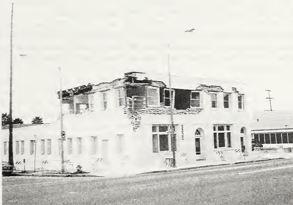
Figure 3.40 In other rehabilitated unreinforced masonry buildings, such as this two story structure in Hollywood, entire wall thicknesses were lost between rows of through-bolts.
