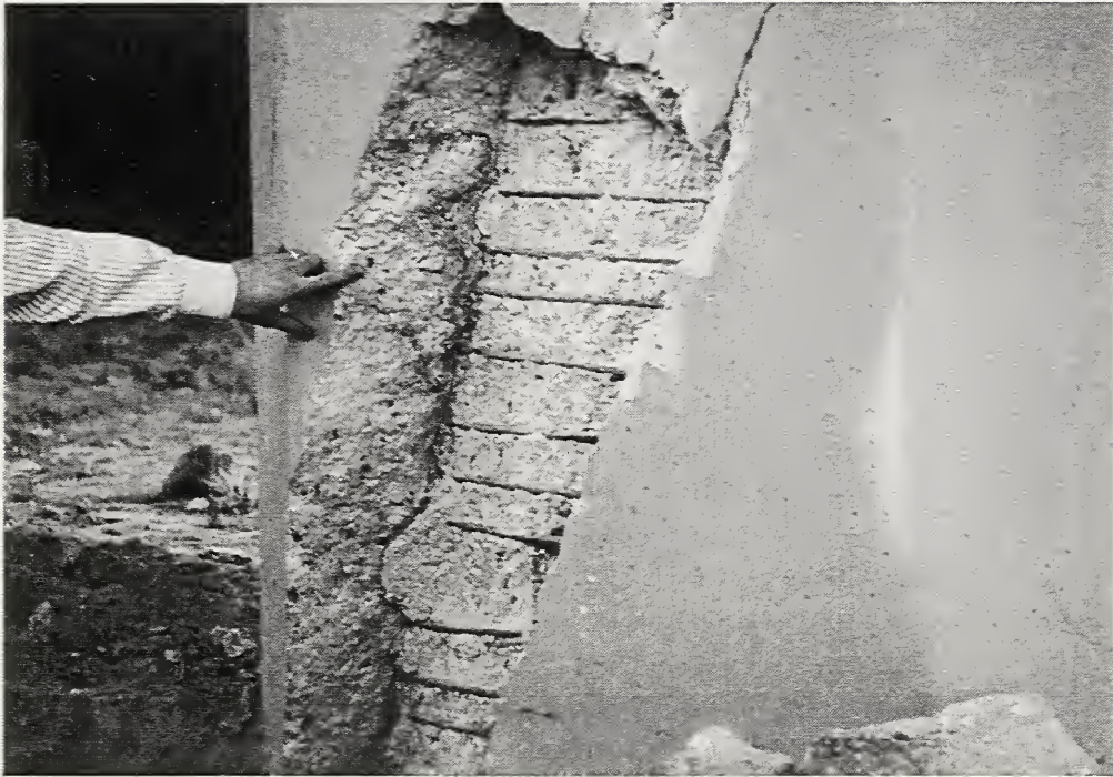
Figure 4.52 Close-up view of the westernmost pier at the Interstate 5, State Route 118, Southwest Connector, looking to the southeast. Loose cover concrete has been removed by Caltrans.
