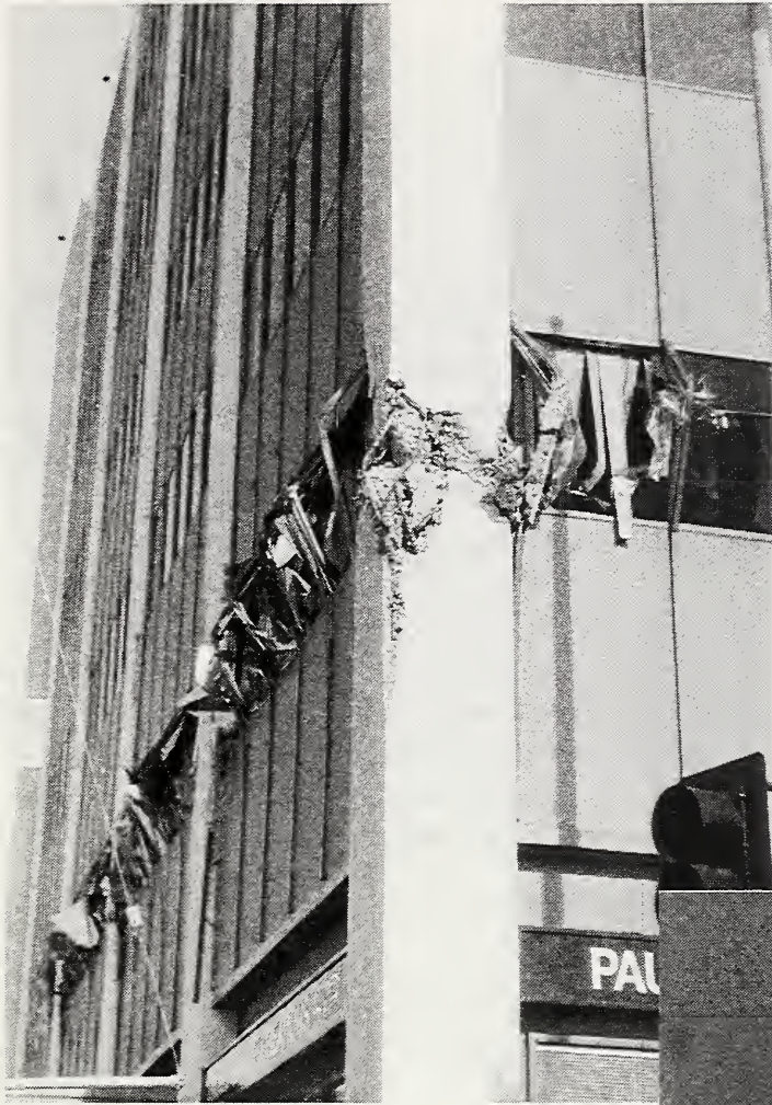
Figure 3.47 The cracking in the concrete columns at the second story was so extensive that the vertical-load carrying capacity of the building was affected. The building settled 50-100 mm at the second story, as these bulging window frames attest. The worst damage was at the southeast corner, the outside corner of the L-shape, pictured here. The building, which developed a slight list, was demolished within days of the quake.
