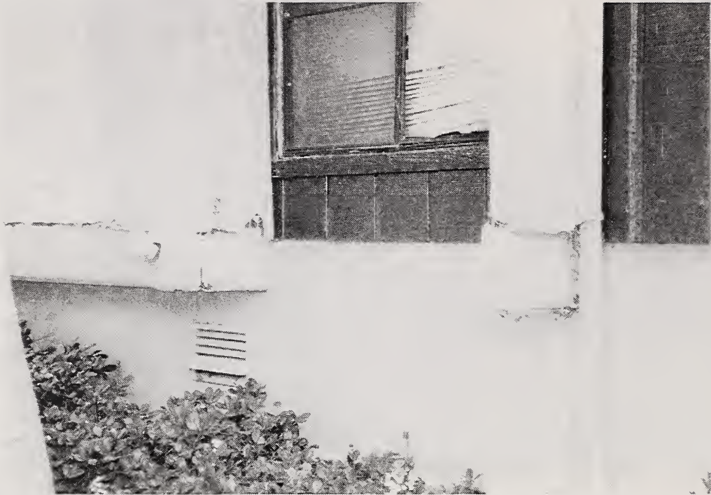
Figure 3.8 Horizontal cracks at the interface of the foundation wall (usually concrete) and the first story (typically wood-framed with stucco facade) were often seen in damaged low-rise apartment buildings.
