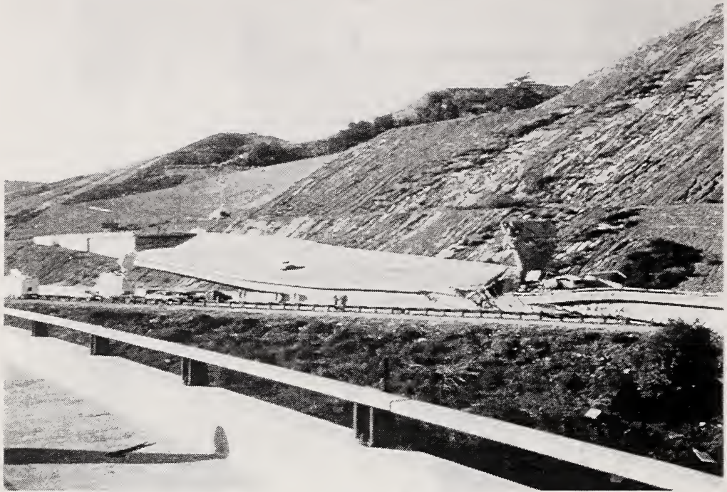
Figure 4.11 Overview of the collapse of the SR14/I5 Separation and Overhead, Ramp C, looking to the south at Abutment 1. Pier 3 can be seen at the right of the photograph (Courtesy of EERC)
