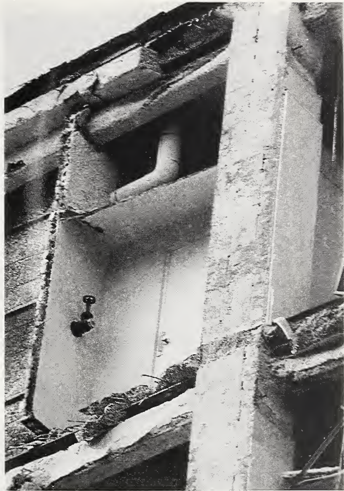
Figure 3.51 The exposed structure of the Sherman Way office building shows remains (at the floor level and the column) of the minimal ties that anchored the masonry facade.
