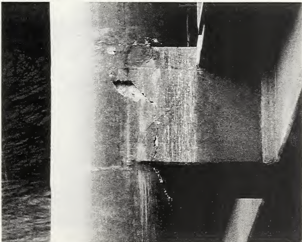
Figure 4.54 Close-up of the outrigger joint at the SR90/I405 interchange, Jefferson Boulevard Undercrossing, center bent, east side, looking to the south
