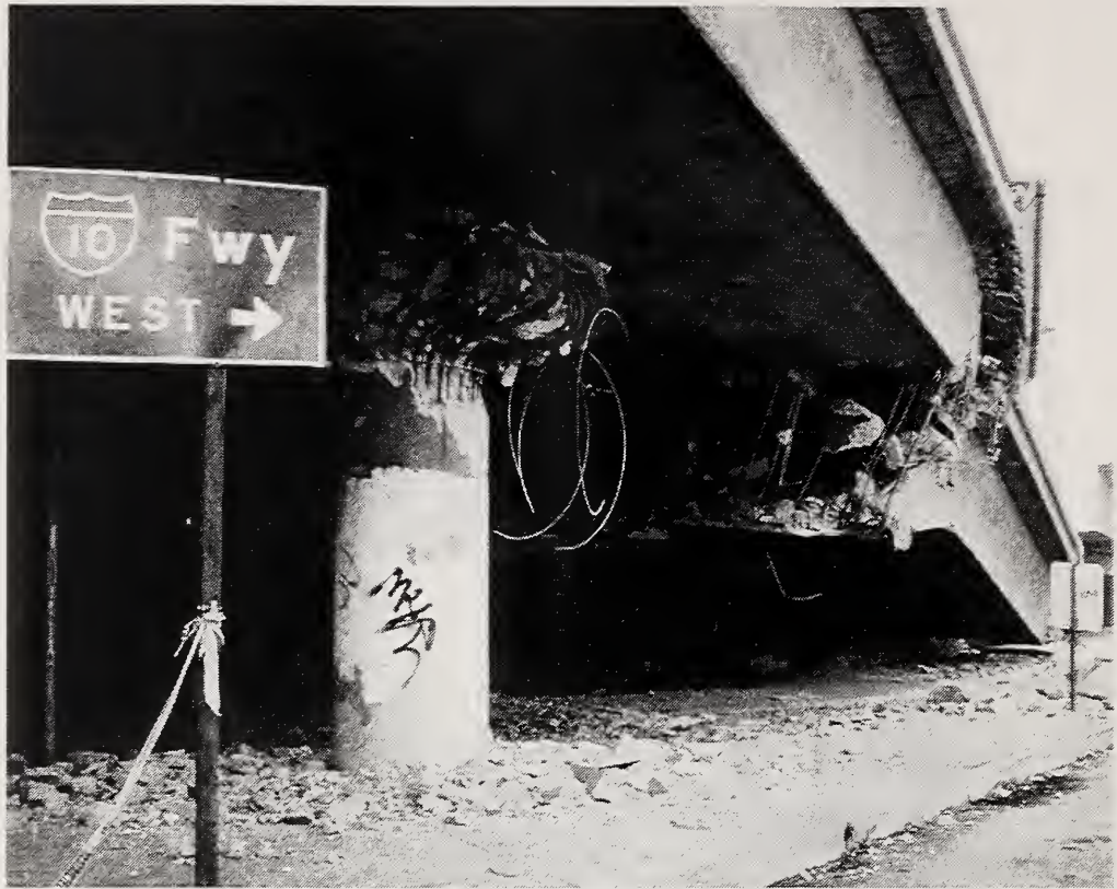
Figure 4.38 Collapsed westbound lane of I10 at Venice Blvd.; pier of Bent 7 in foreground
