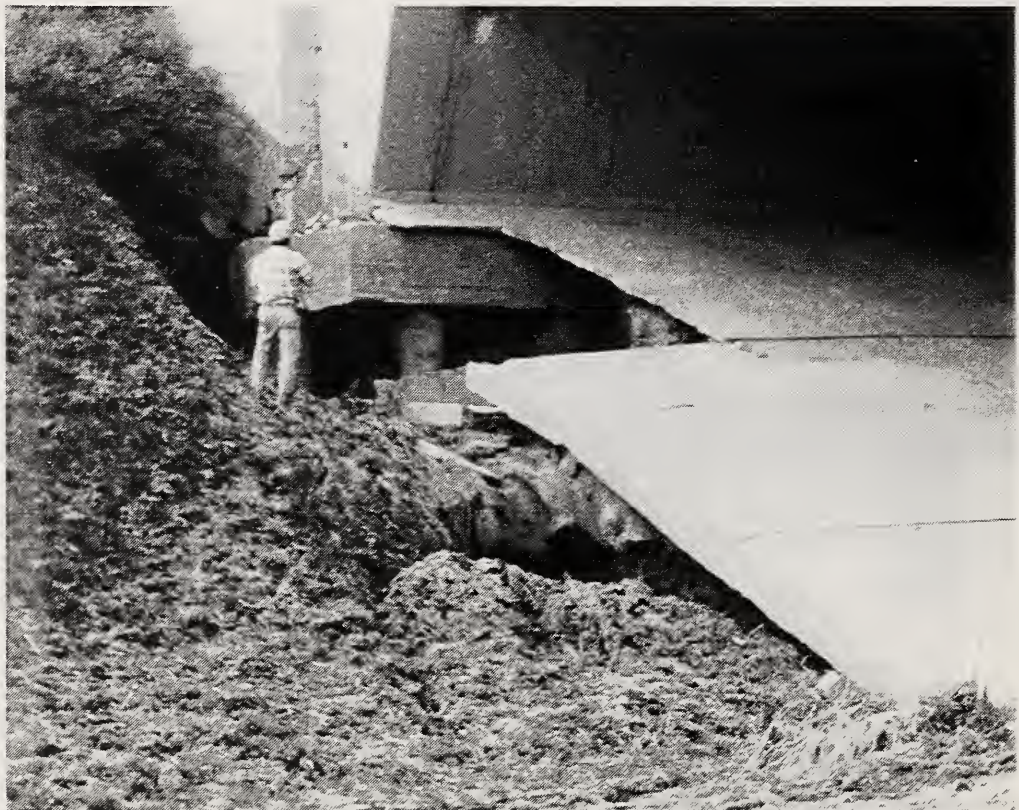
Figure 4.32 SR118 Balboa Avenue Overcrossing, view of the washout on the east side of the south abutment, caused by a ruptured water main
