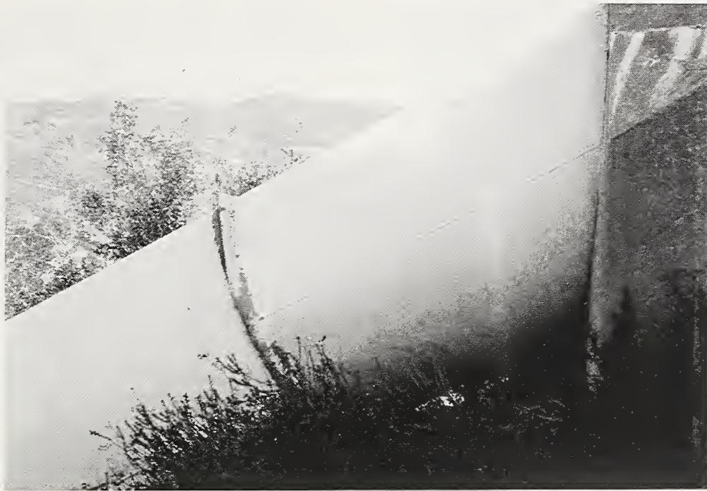
Figure 5.3 The steel pipeline at Terminal Hill separated from its supporting saddle at several places and pipe sections bulged at other locations along the alignment.
