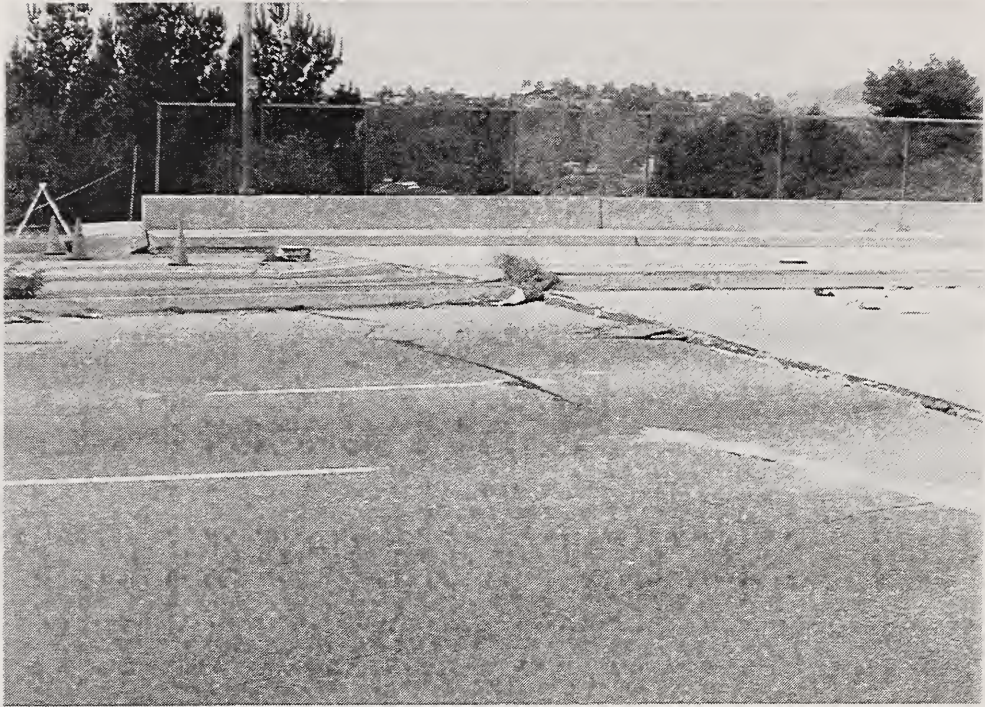
Figure 5.20 Transverse cracks in pavement near the intersection of Balboa Boulevard and SR118.
