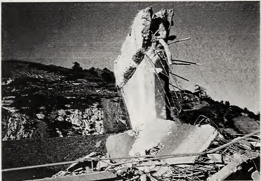
Figure 4.12 Damage at Pier 3 of the SR14/I5 Separation and Overhead, Ramp C, looking to the west (Courtesy of EERC)
