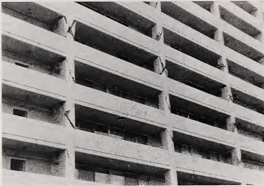
Figure 3.14 The back of the Champagne Towers building was badly damaged. The railings here are solid infill, which effectively stiffen the lower half of the columns. The shortened upper half of the columns were forced to accommodate all the displacement, and they failed in shear.
