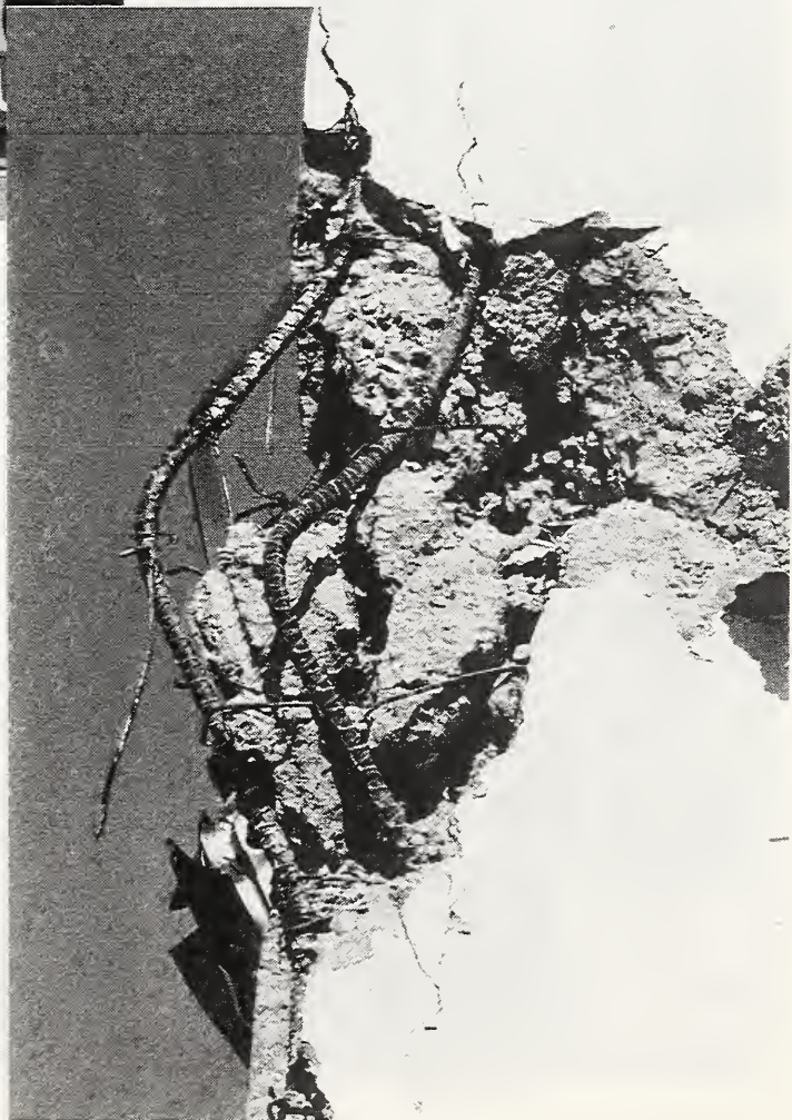
Figure 3.48 A close up of the damaged southeast corner of the Barrington Building shows the widely spaced, undeformed bars used for transverse reinforcement.
