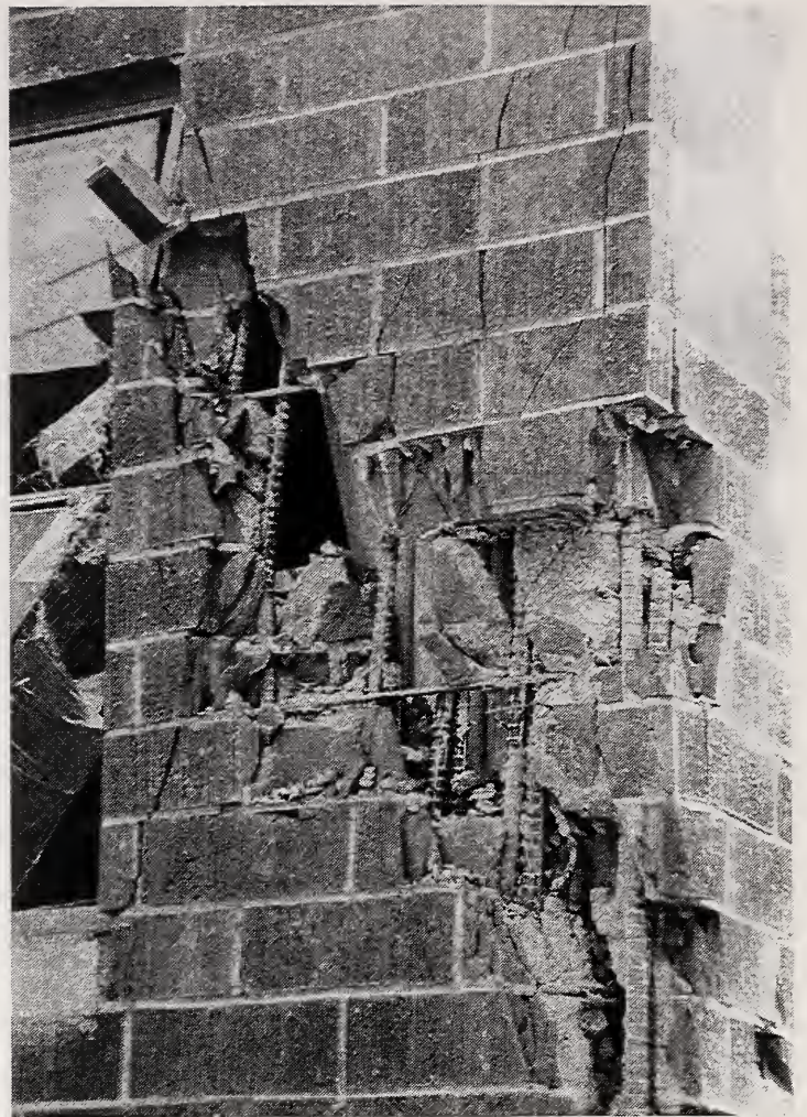
Figure 3.27 The facade of the five-story Berkley Convalescent Hospital directly adjacent to the St. John's Hospital complex consisted of two wythes of brick masonry with a reinforced and grouted space between. In some places, all three layers of this facade were destroyed along lines of diagonal cracking. The facility was evacuated.
