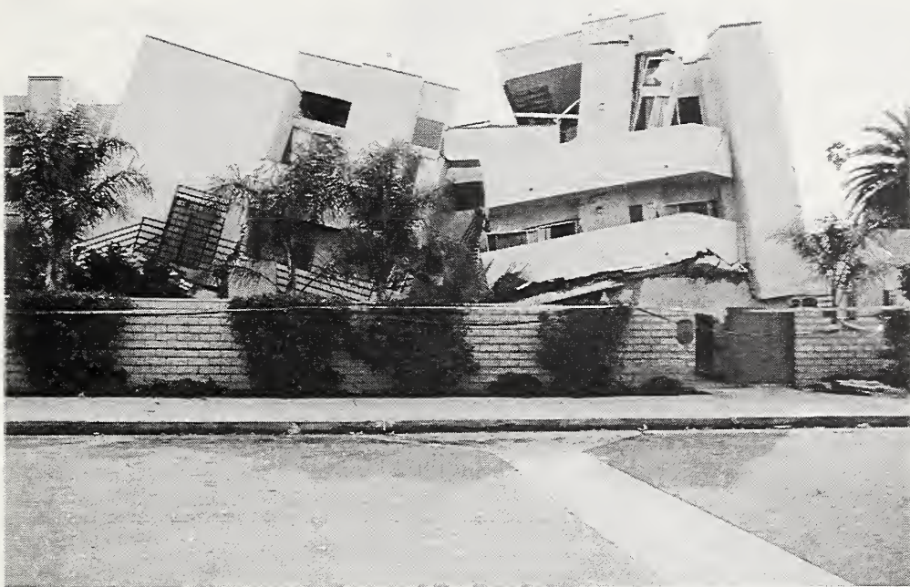
Figure 3.10 The central row of concrete first-story columns in a three story apartment building on Sherman Way in Sepulveda collapsed, causing the wood-framed upper stories to settle inward.
