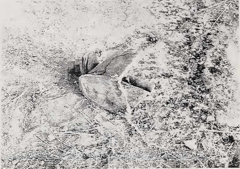
Figure 5.5 Welds of the restrainers broke as the result of strong shaking.
