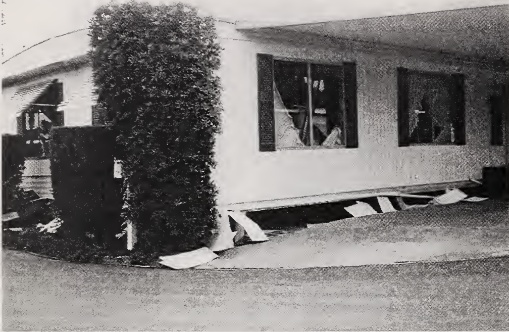
Figure 3.19 Damage to manufactured homes caused by collapsed supports was common.
