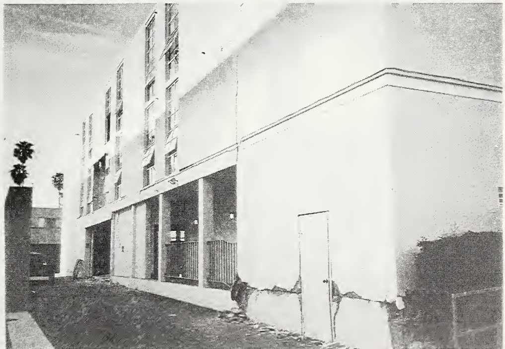
Figure 3.26 The Bay Vista Health Care Center was closed due to damage. Differential movement between the building and its base was indicated by the crack at the foundation line. The corner of the concrete foundation wall spalled, apparently due to crushing. A facade panel over the garage opening was dislodged.
