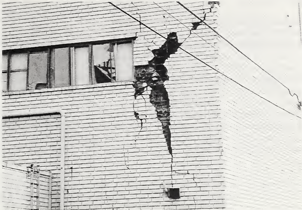
Figure 3.59 A close-up view of the damage shows the pattern of reinforcing used in the masonry facade.
