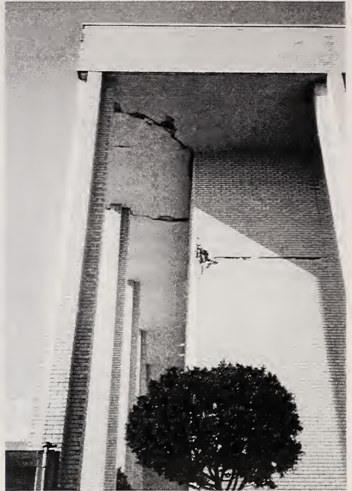
Figure 3.31 The Broadway department store at the Northridge Fashion Center had horizontal cracks in the facade and spalled corners at each floor level, and cracks in the soffit.
