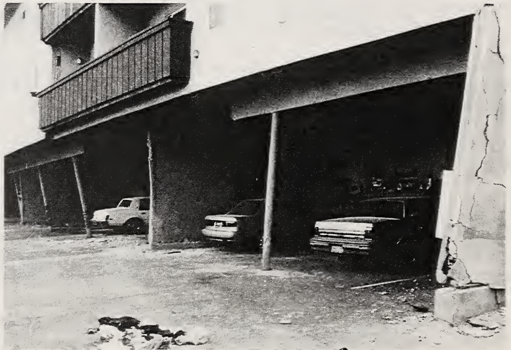
Figure 3.5 Steel pipe columns between parking bays supported the upper stories of the Northridge Meadows apartment buildings. Few of the buildings in the north half of the complex collapsed, but all were damaged.
