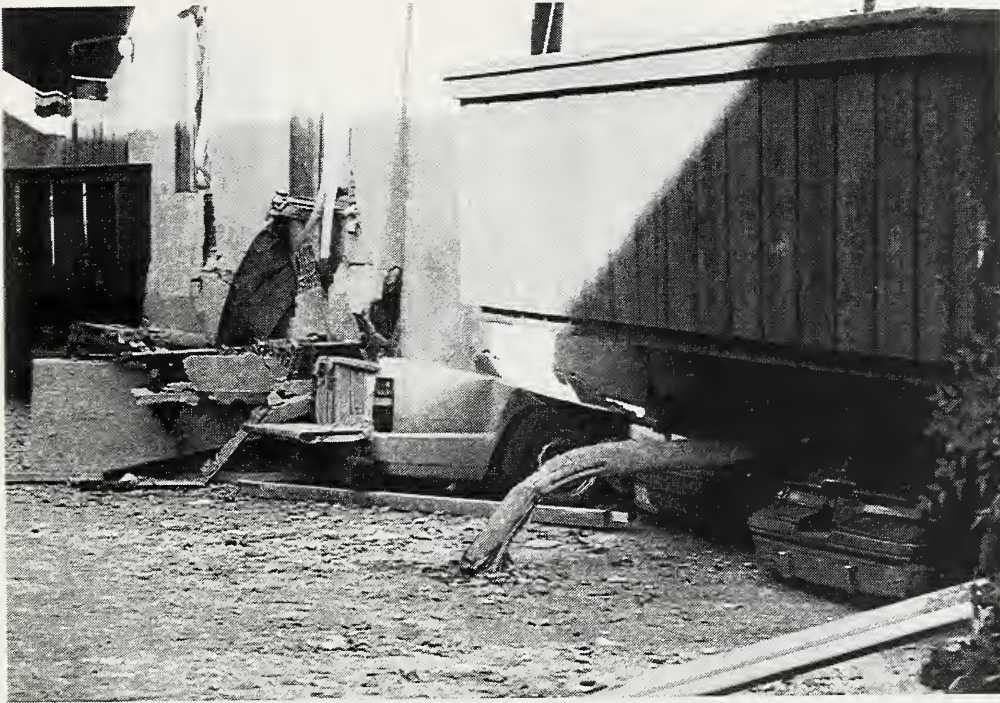
Figure 3.6 At Northridge Meadows, the first story steel pipe columns generally hinged near their bases but retained their length, controlling the displacement of the upper stories.
