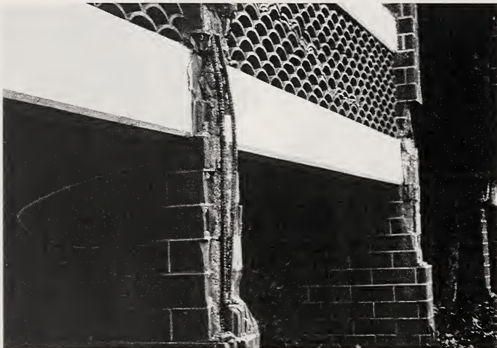
Figure 3.28 Two faces of the Berkley Convalescent Hospital had wing walls separating balconies. The ends of these wing walls spalled at the lower stories.
