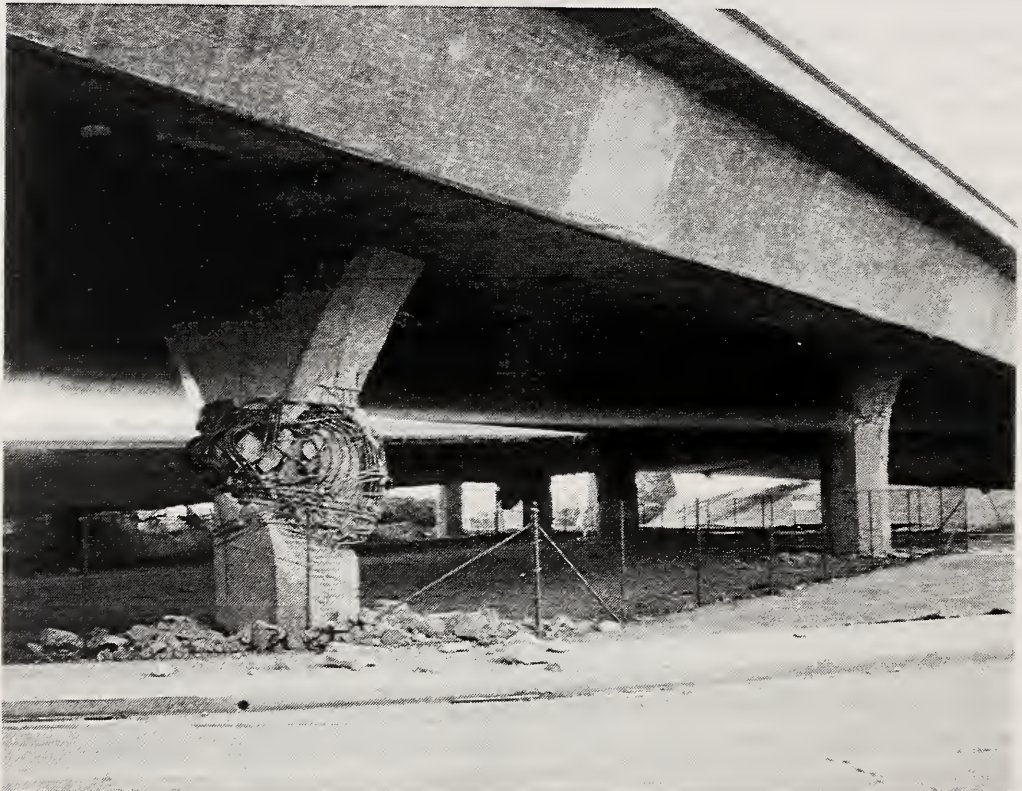
Figure 4.20 Damage to piers of the SR118 Mission-Gothic Undercrossing, looking to the northwest at the north face of the westbound bridge, Bents 3 (foreground) and 2.
