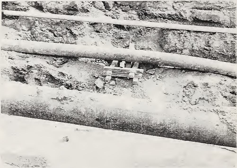
Figure 5.14 Some of the buried pipelines located near the intersection of Balboa Boulevard and Bircher Street--the potential hazard of co-location of lifeline systems. At this site are three water lines (two of them main lines); three gas lines; two sewers; one crude oil line; overhead power, telephone, and cable TV lines; the street lighting system; and the street itself.
