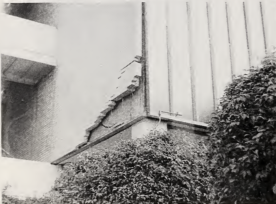
Figure 3.50 The similar west wall of was damaged, but did not peel away from the structure. This close up of the interface between the first and second stories shows that the masonry facade is supported on a steel angle. At the west end of the building, the facade was crushed at the toe where it is supported by the angle.
