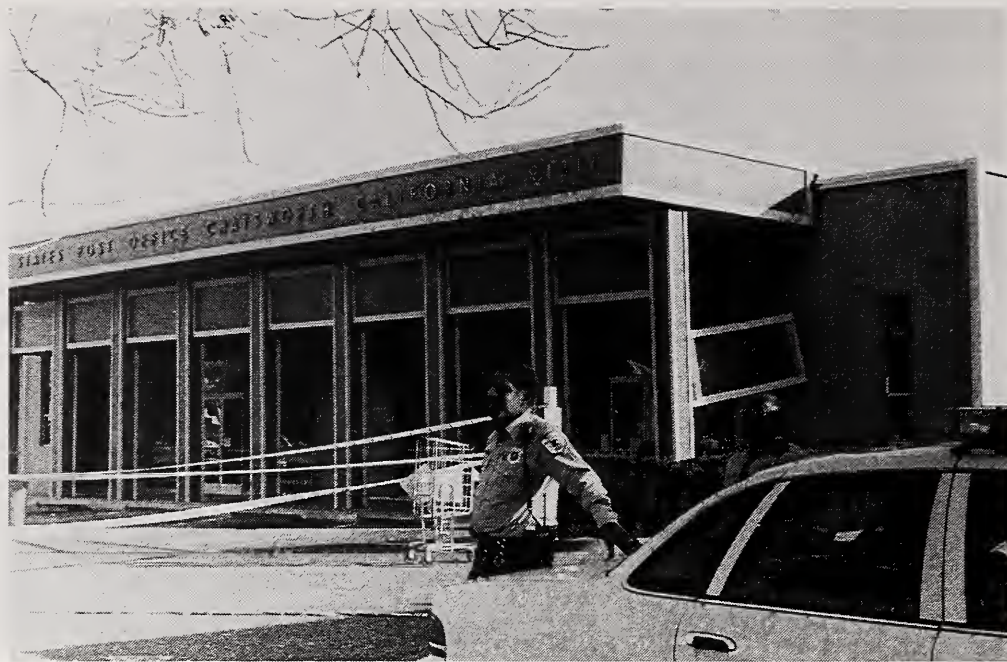
Figure 3.35 The Chatsworth Post Office was closed due to damage. Mail was being collected in the parking lot.
