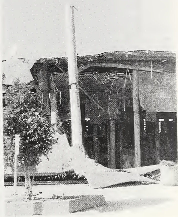
Figure 3.29 A portion of the concrete waffle slab roof and the interior floor slabs at the Bullock's department store at the Northridge Fashion Center mall fell to the basement, leaving many of the columns standing. No reinforcing steel can be seen in the remaining columns that would have connected the columns to the floor slabs.
