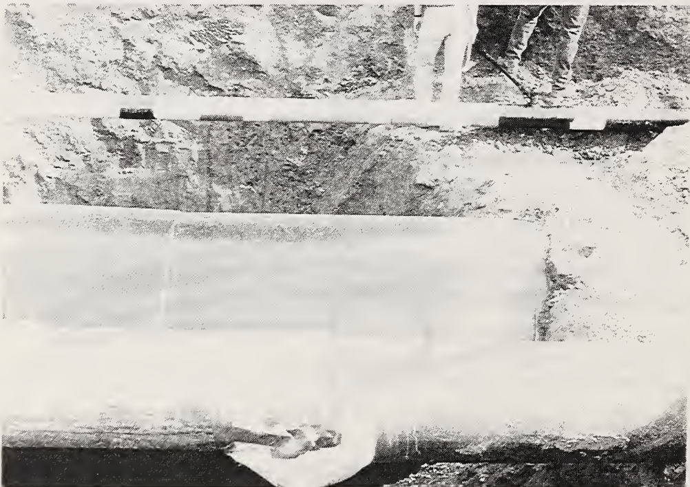
Figure 5.10 Ground contraction along Balboa Boulevard caused the rupture of a gas distribution line, the Rinaldi trunk water main, and a gas main.
