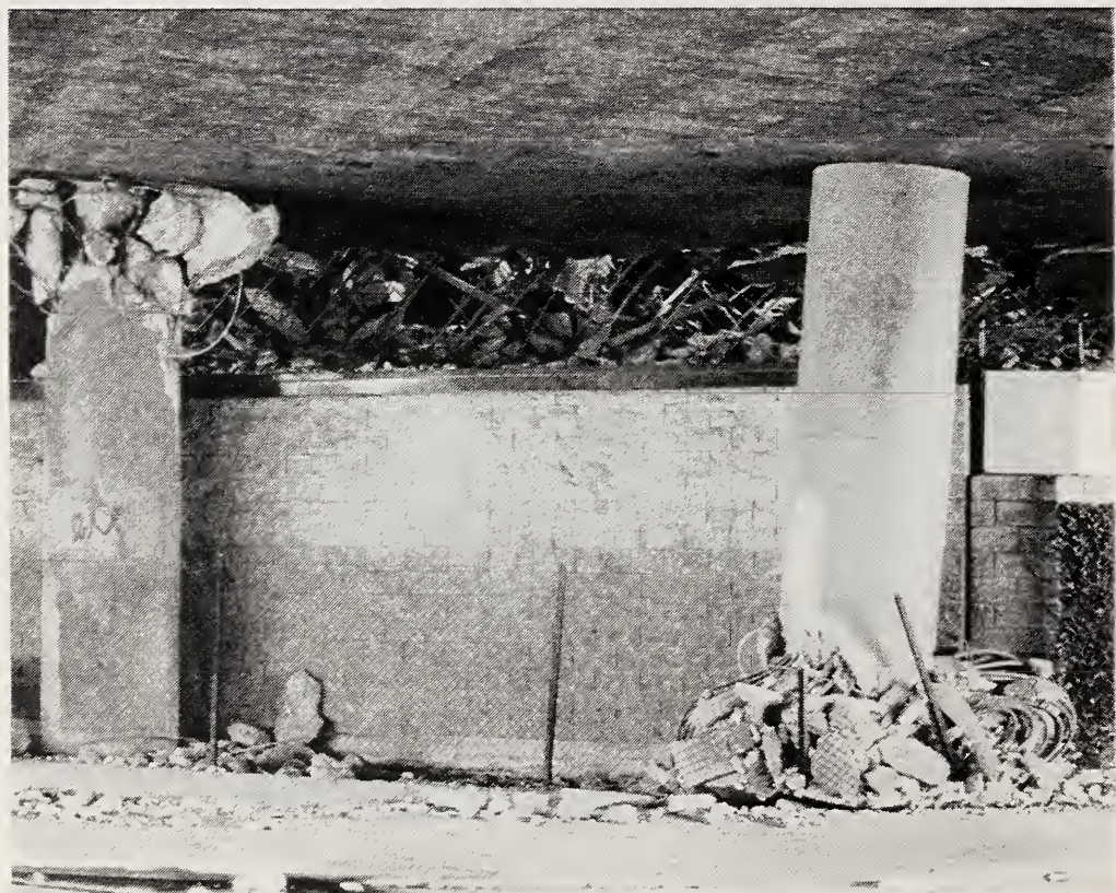
Figure 4.39 Failed piers in Bent 7 supporting westbound lane of I10 at Venice Blvd.
