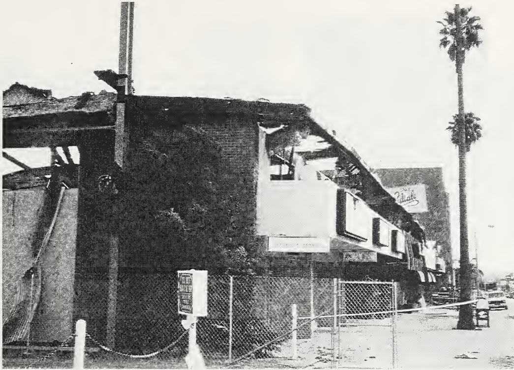
Figure 6.2 Fire damage in a two story commercial building.
