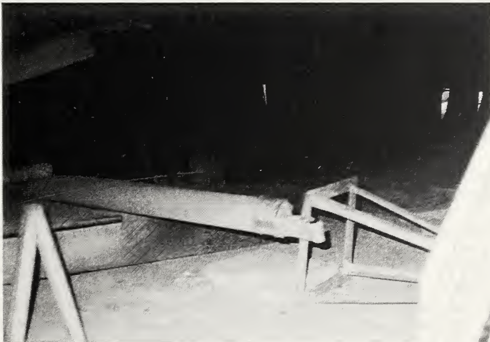
Figure 3.22 The metal supports under many homes tipped over, bringing down the houses above.
