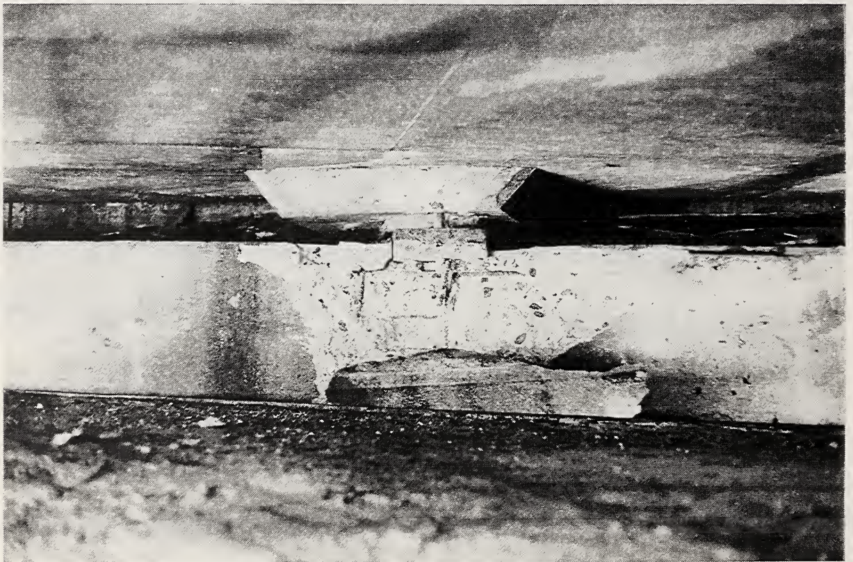
Figure 4.48 Abutment damage at sliding-type bearing
