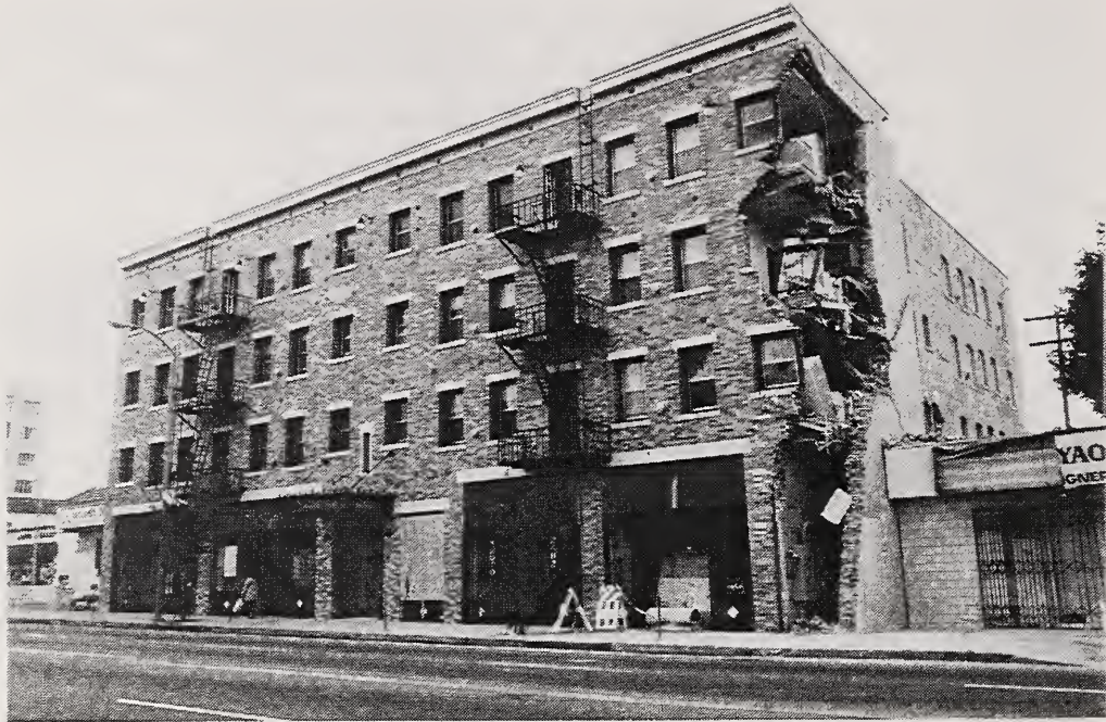
Figure 3.37 The corner of this rehabilitated unreinforced masonry apartment building in East Hollywood crumbled on all four stories.
