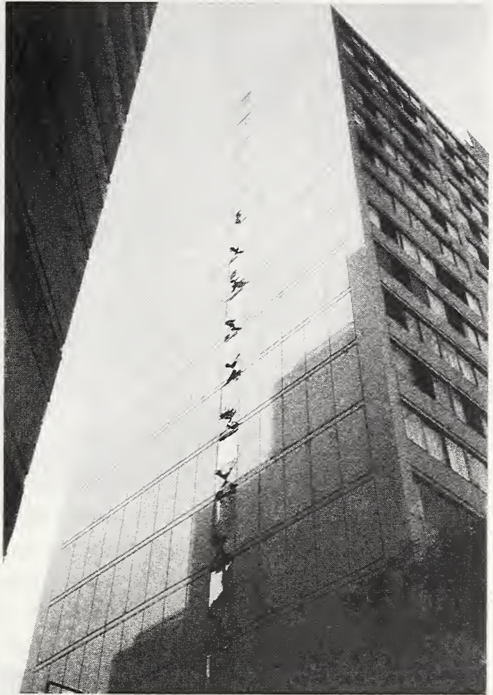
Figure 3.12 Champagne Towers apartment building in Santa Monica suffered a classic form of earthquake damage: shear failure of the coupling beams between linked shear walls at the transverse end of the building.
