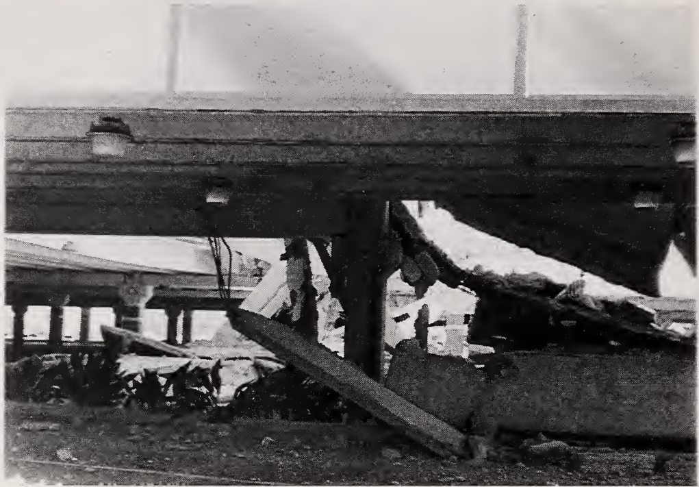
Figure 3.68 In precast parking garages, the support of the double-tees that comprise the floors is a vulnerable link in the system. This garage, at the north end of the Northridge Fashion Center, illustrates a common failure: the double-tees pulled off their supports, leaving the column-beam frame essentially intact.
