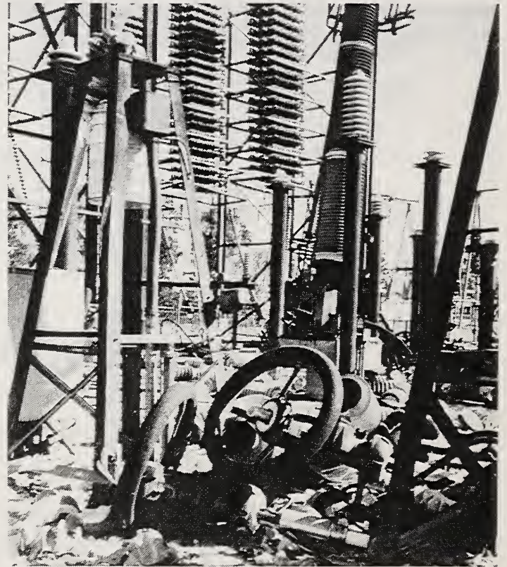
Figure 5.16 Porcelain is an integral part of high voltage electrical equipment due to insulation requirements and is also the most vulnerable to damage during strong earthquake shaking. (Photo courtesy of Edward Matsuda, Pacific Gas and Electric Company.)
