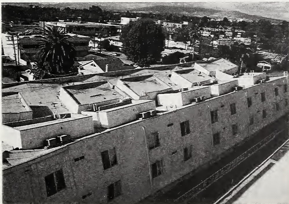
Figure 3.11 This overhead view of the partially-collapsed apartment building on Sherman Way shows the solid concrete masonry block perimeter walls along the longitudinal axis of the building. Access to the first story parking was limited to the transverse ends of the building. When the row of interior columns failed, both sides of the building settled in towards the middle.
