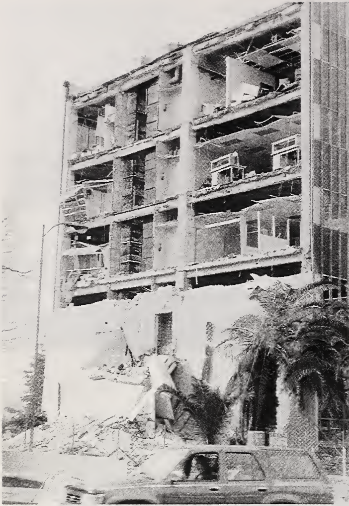
Figure 3.49 The east end wall and stair tower of a five-story apparently steel-framed office building on Sherman Way in Reseda collapsed. The enclosing masonry wall became detached from the structure and slid to the ground, with the upper stories remaining intact. The doorway opening in the wall, shown here resting at about the second story level, originally provided access from the top story to the stair tower.
