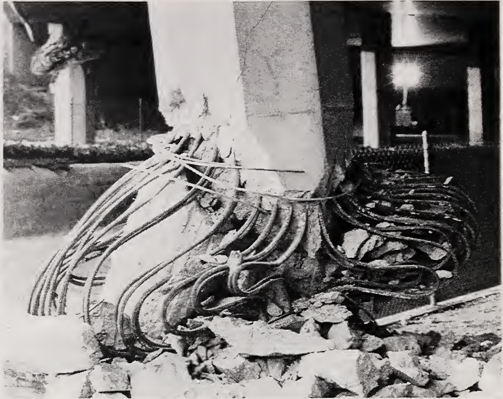
Figure 4.27 Damage to pier 3S-1 of State Route 118 at Bull Creek Canyon Channel, looking to the northwest
