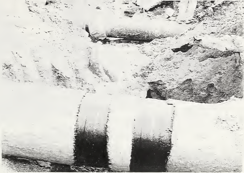
Figure 5.11 Ground extension along Balboa Boulevard resulted in the rupture of the same gas main and water main shown in Figure 5.10. The rupture of the gas main here caused a major fire that engulfed five houses.
