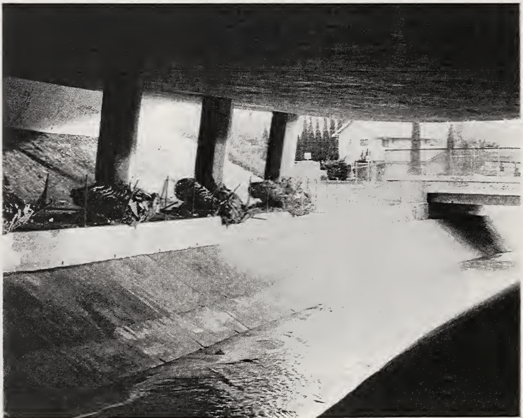
Figure 4.28 Damage to piers of Bent 3S of State Route 118 at Bull Creek Canyon Channel, looking to the southeast.
