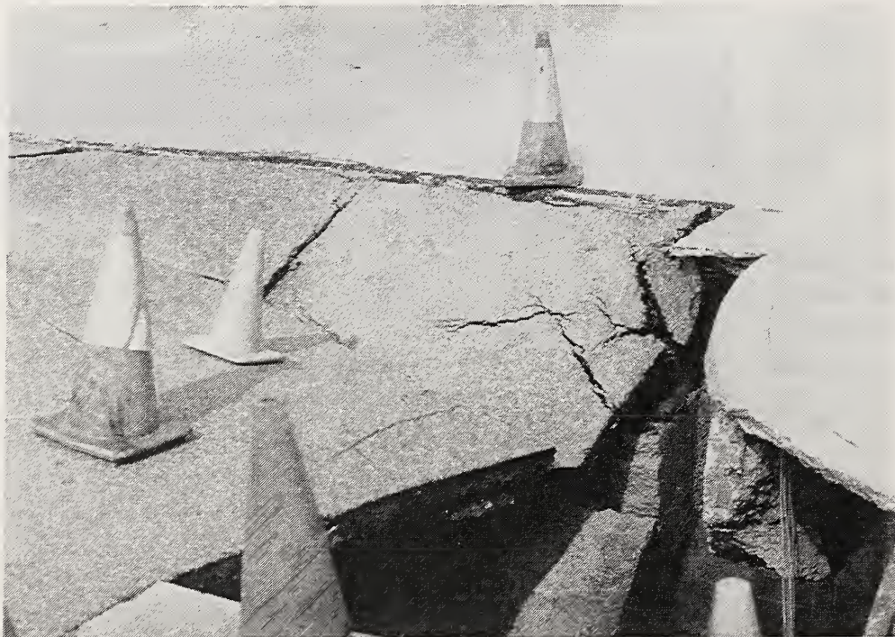
Figure 5.21 The approach of Balboa Boulevard at SR118 caved in due to the loss of the abutment fill because of a water main break.
