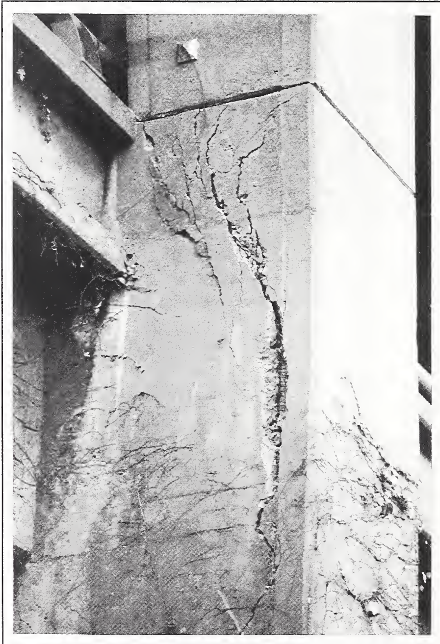
Figure 3-23 Cypress Viaduct Pedestal Failure
