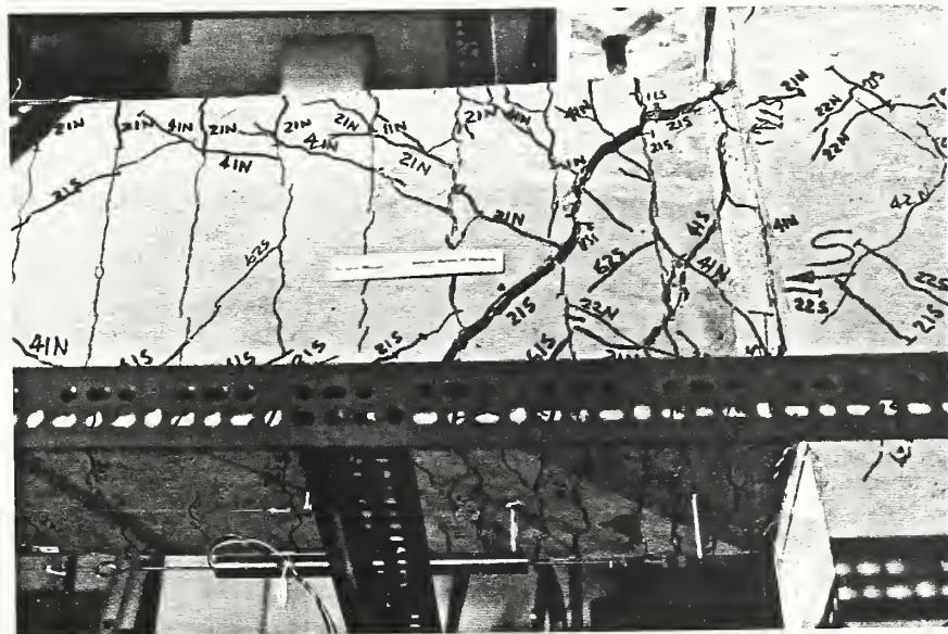
Fig. 4.24 Shear crack opening of A-M-Z4 at 6 \Delta_y , cycle 2.
