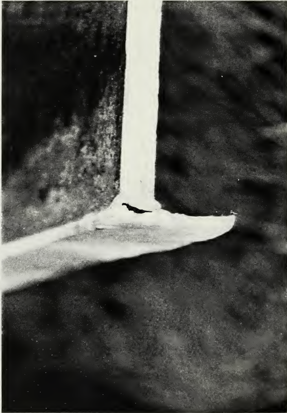
Figure 3.6 - Tear in Tank Bottom at Inside Fillet Attaching First Shell Course and Bottom Plate
