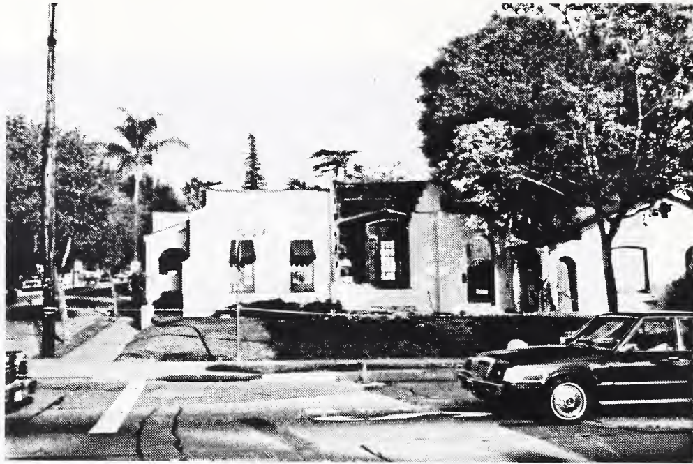
Photo 7 Many houses with unreinforced hollow clay tile walls sustained severe damage. This house at the corner of Greenleaf Avenue and Beverly Blvd. in Whittier lost the front wall.
