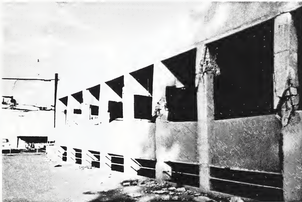
Photo 26 Extensive damage to relatively short columns and the ends of deep beams.
