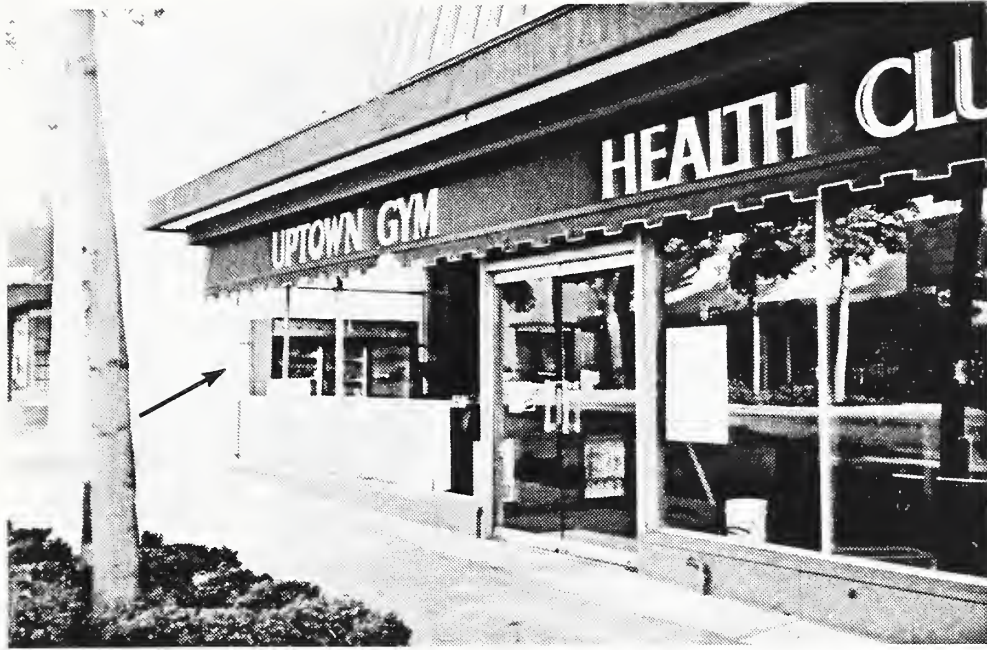
Photo 33 Distortion of the building caused damage to windows at the corner of the building in the Uptown Whittier shopping section.
