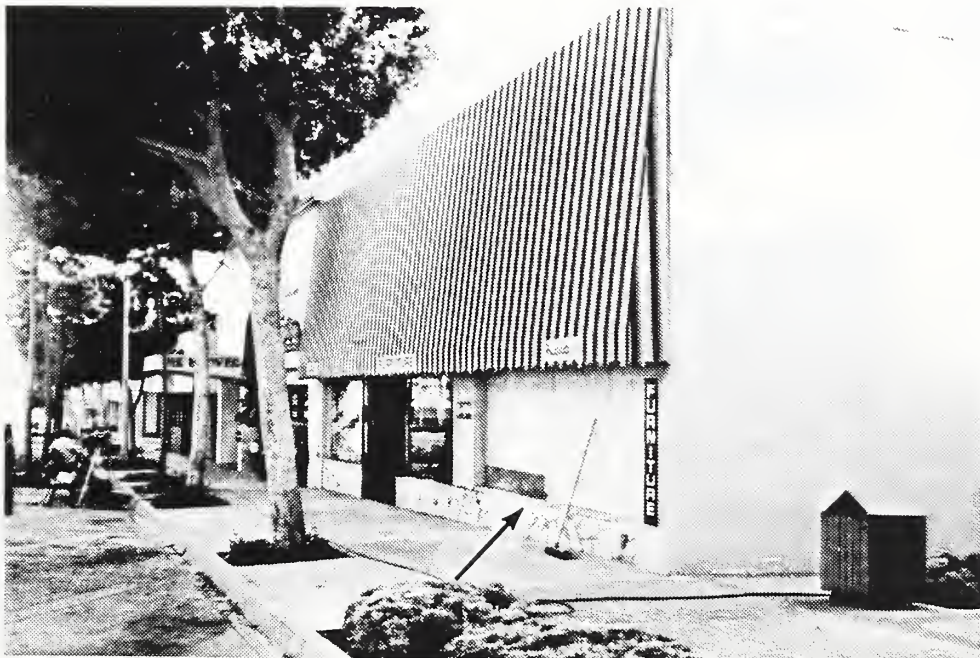
Photo 34 Damage glass in a store in the Uptown Whittier shopping section.
