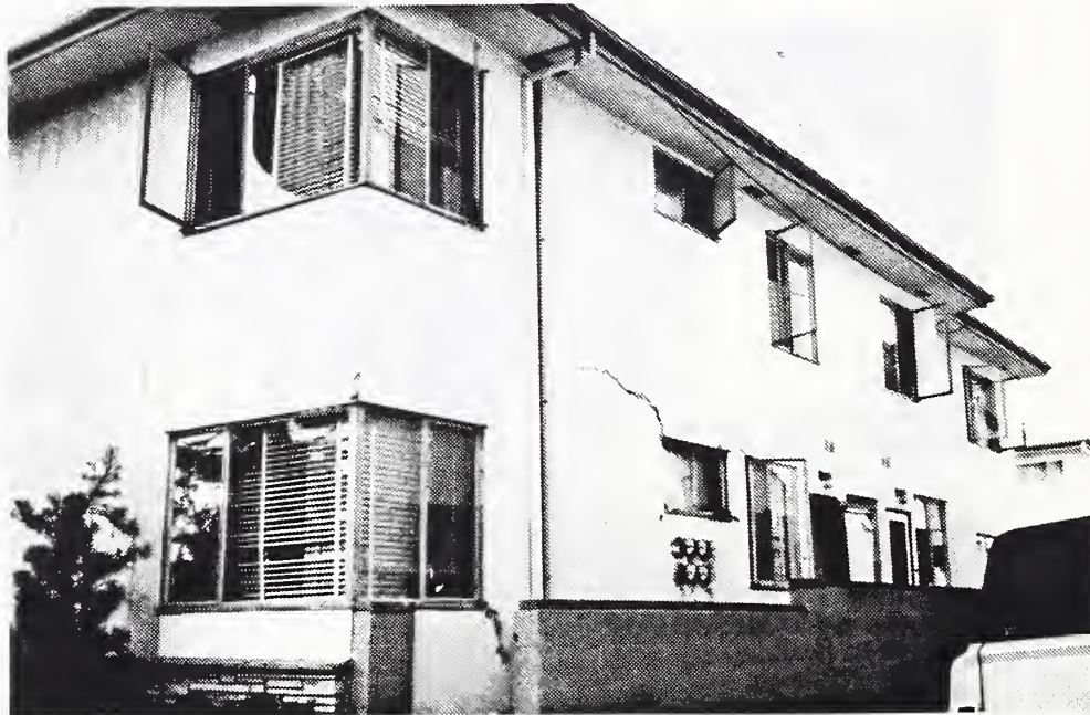
Photo 16 Large cracks developed at the corners of window openings. Note broken window panes at the corner of the building, Whittier.
