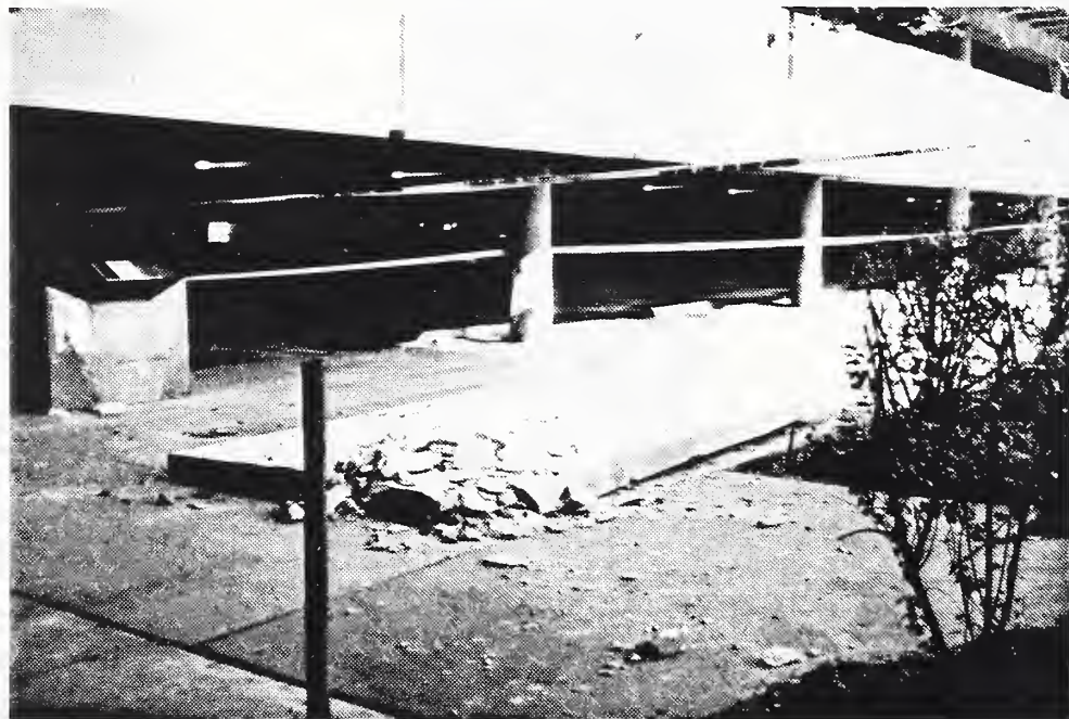
Photo 24 A precast concrete fascia unit fell two stories and fatally injured a passer by. This was the only fatality of the earthquake due to a structural failure.
