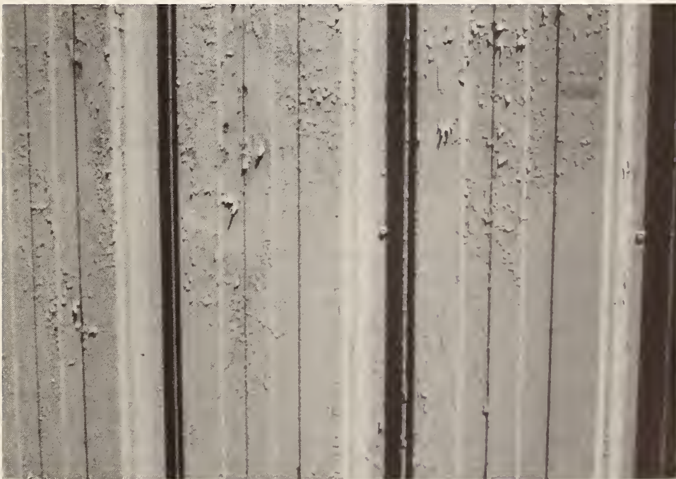
Figure 23. Adhesion failure of maintenance coating to a thin organic factory coating
