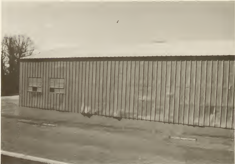
Figure 7. Impact damage of metal panels
