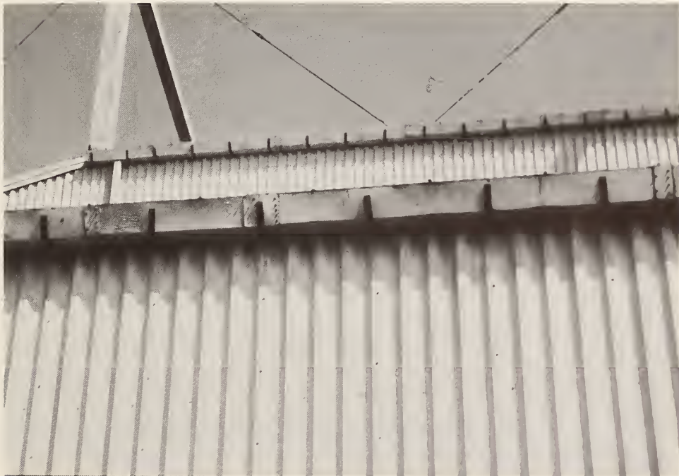
Figure 9. Corroded gutter hangers
