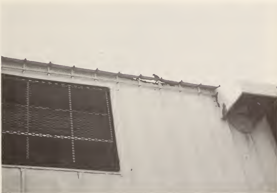
Figure 3. Illustration of loss of metal at top edges of panels under the eave
