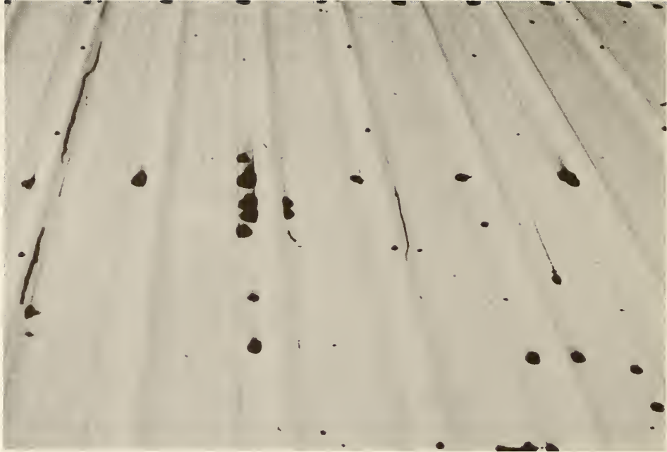
Figure 10. Corroded fasteners with associated corrosion of the metal panels
