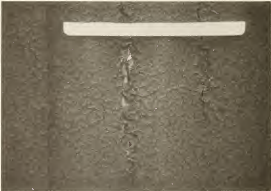
Figure 13. Cracking of bituminous coating
