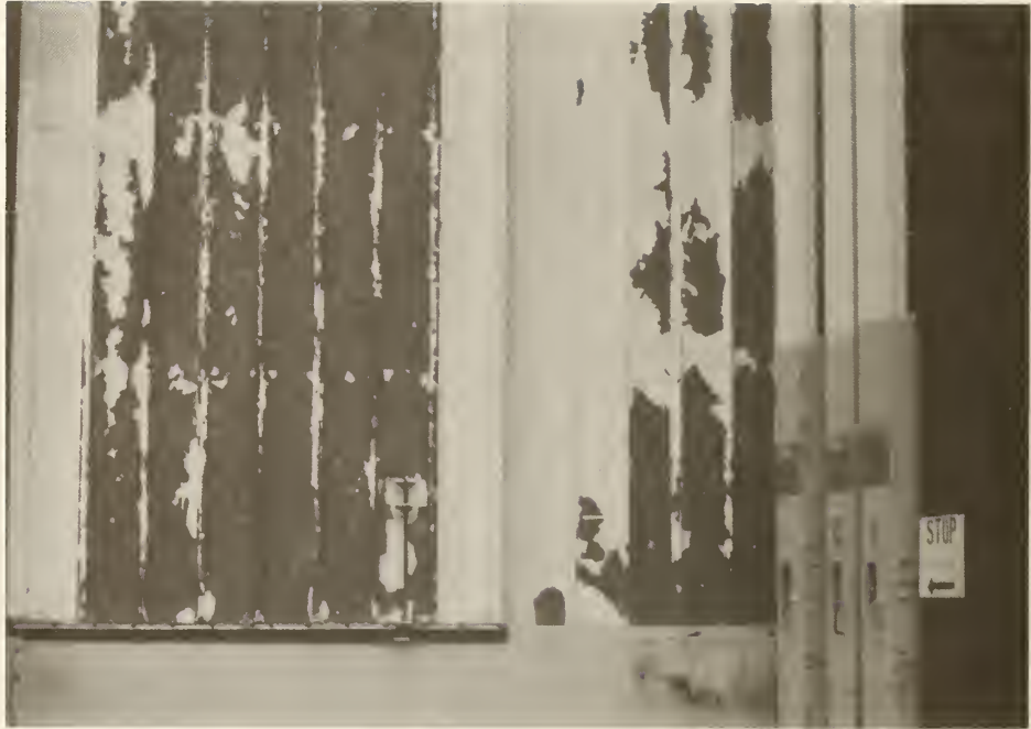
Figure 18. Peeling of alkyd coating from galvanized steel panels
