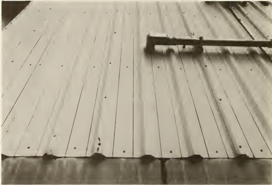
Figure 16. Corrosion along factory formed bends of steel panels protected by a thin organic coating
