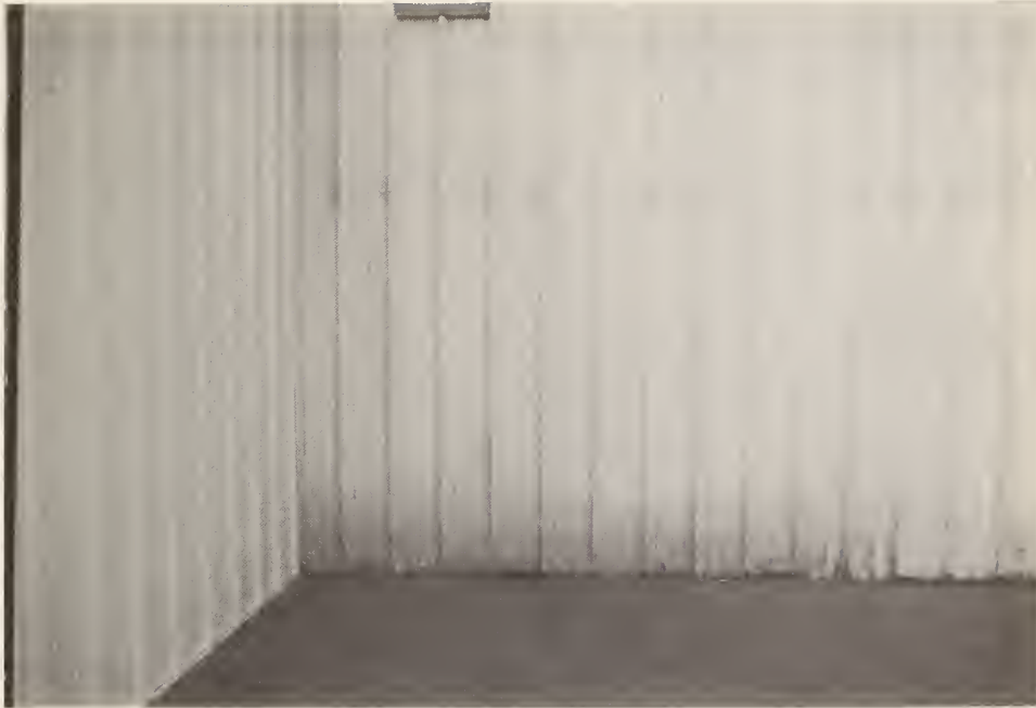
Figure 2. Illustration of loss of metal at bottom edges of panels
