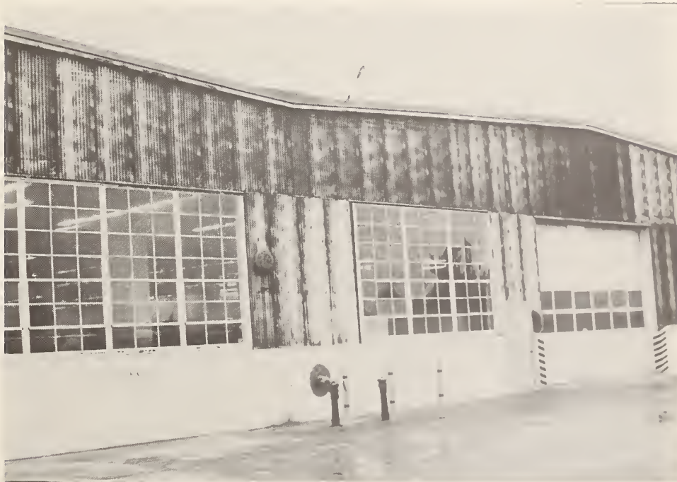
Figure 15. Fibers of reinforcing fabric showing on surface of deteriorated bituminous coating
