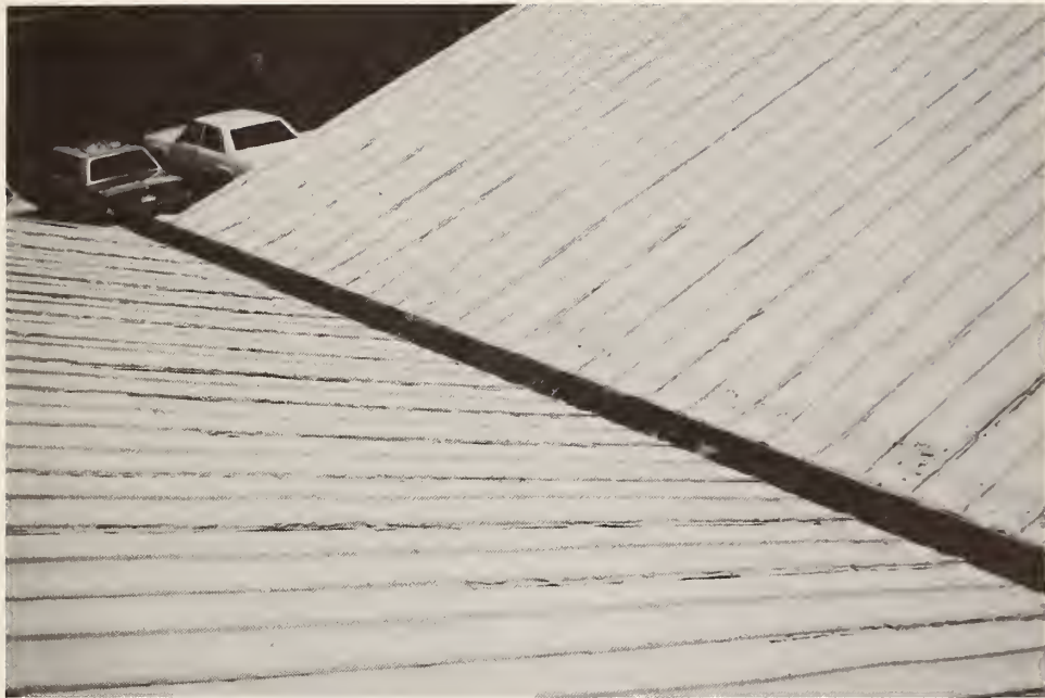
Figure 8. Deterioration of drainage system
