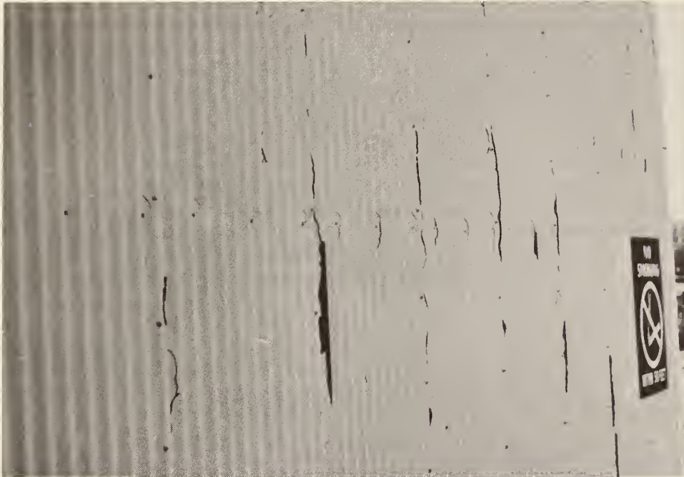
Figure 22. Peeling of bituminous factory coating system recoated with a mineral spirit solvent paint
