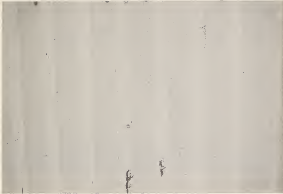
Figure 14. Cracking of topcoated bituminous coating systems
