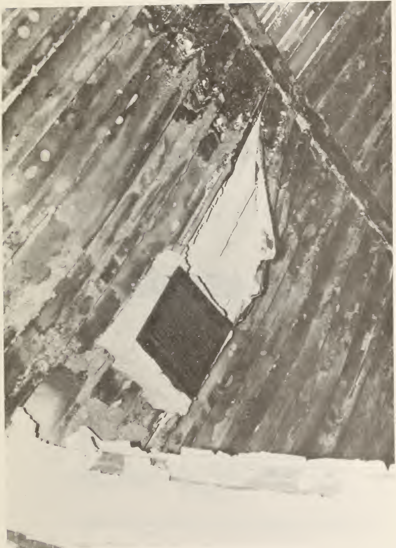
Figure 24. Photograph showing bottom of walk-on deck after test 1
