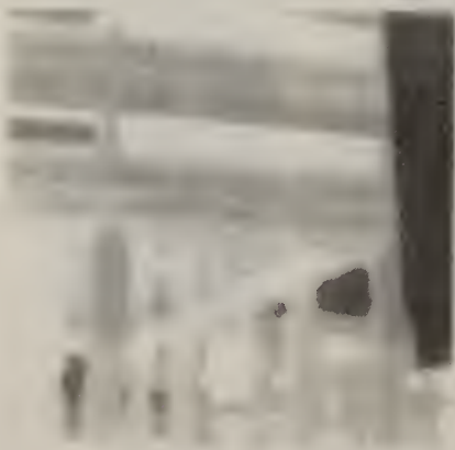
18-5 Third floor overhang of the N wall at the W end
