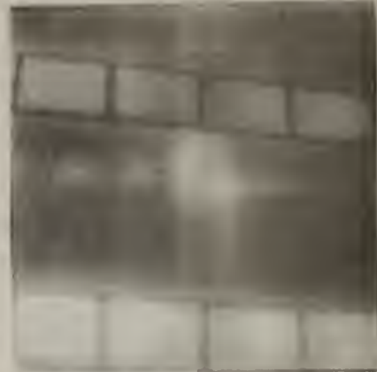
20-2 Close-up of the floor-wall- post seam on the E face of the N wing
