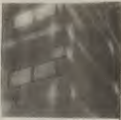
20-3 SW corner showing seams at the second and third floors
