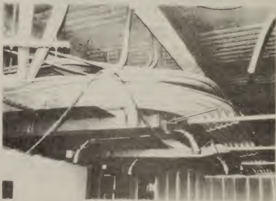
Figure 2.15 Typical air supply and return duct system in ceiling of occupied space (with drop ceiling removed)
