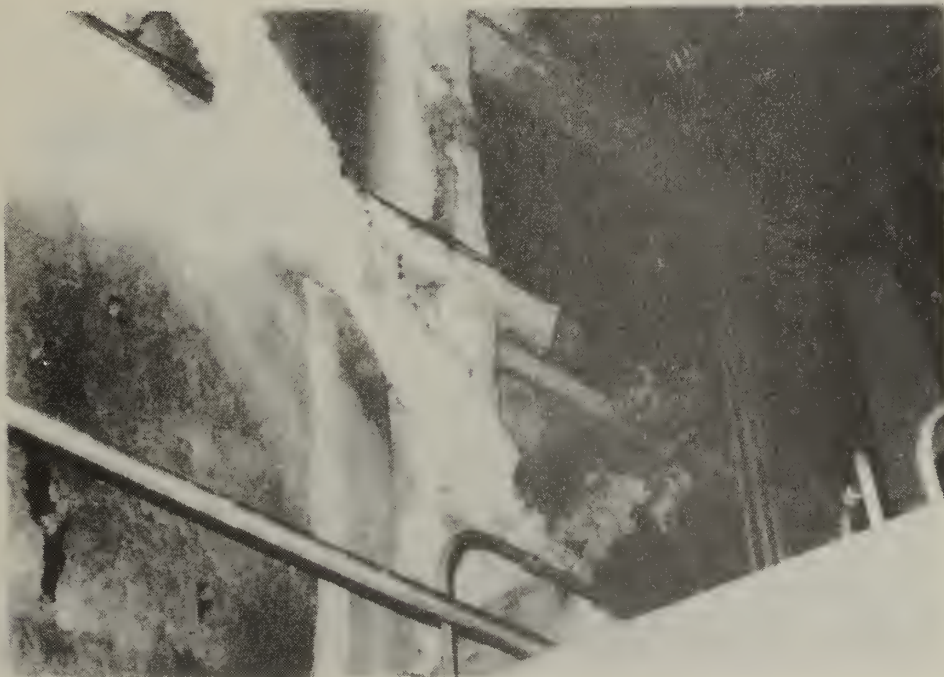
Figure 2.4 Damaged sprayed-on fireproofing on vertical steel bracing members
