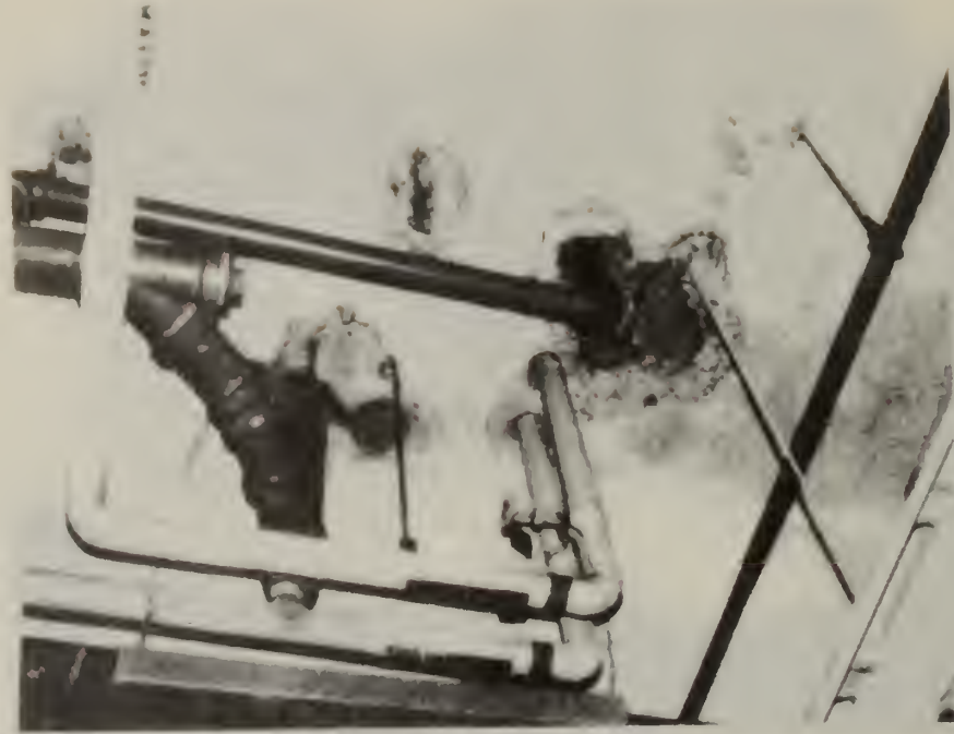
Figure 2.9 Damage to fireproofing caused by floor penetrations for plumbing system modifications
