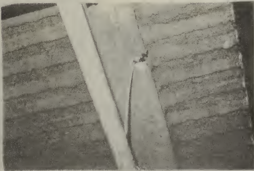
Figure 2.8 Fireproofing damaged by addition of hangers during modifications to plumbing and HVAC systems
