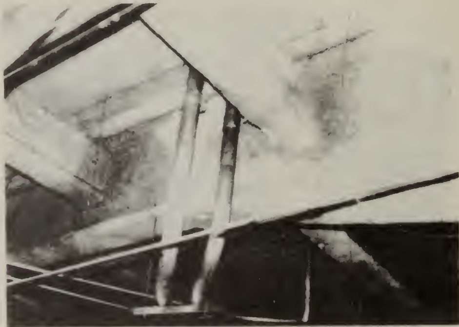
Figure 2.10 Damage to fireproofing on structural steel due to HVAC system modifications
