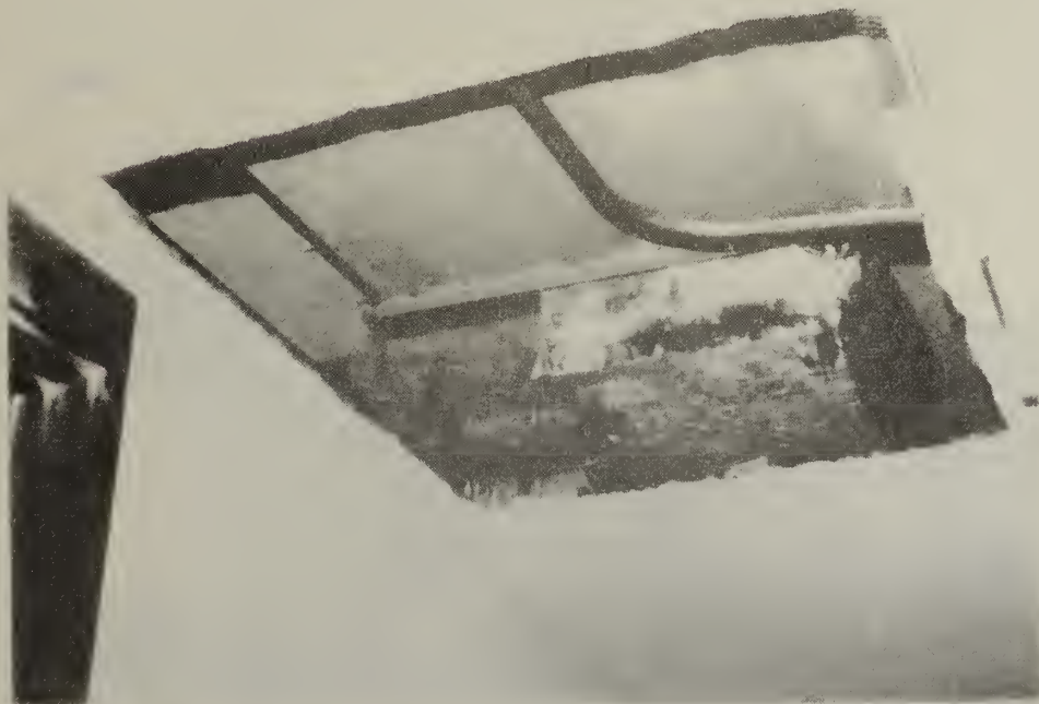
Figure 2.17 Drywall ceiling construction with hole cut for maintenance work in the plenum
