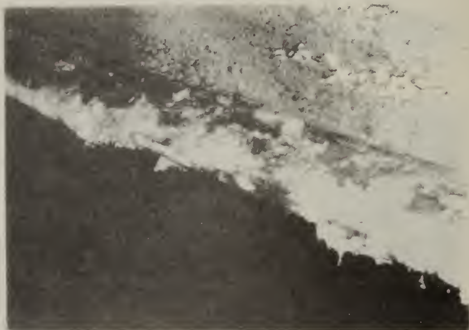
Figure 2.6 Horizontal structural member easily accessible to building occupants with damaged fireproofing
