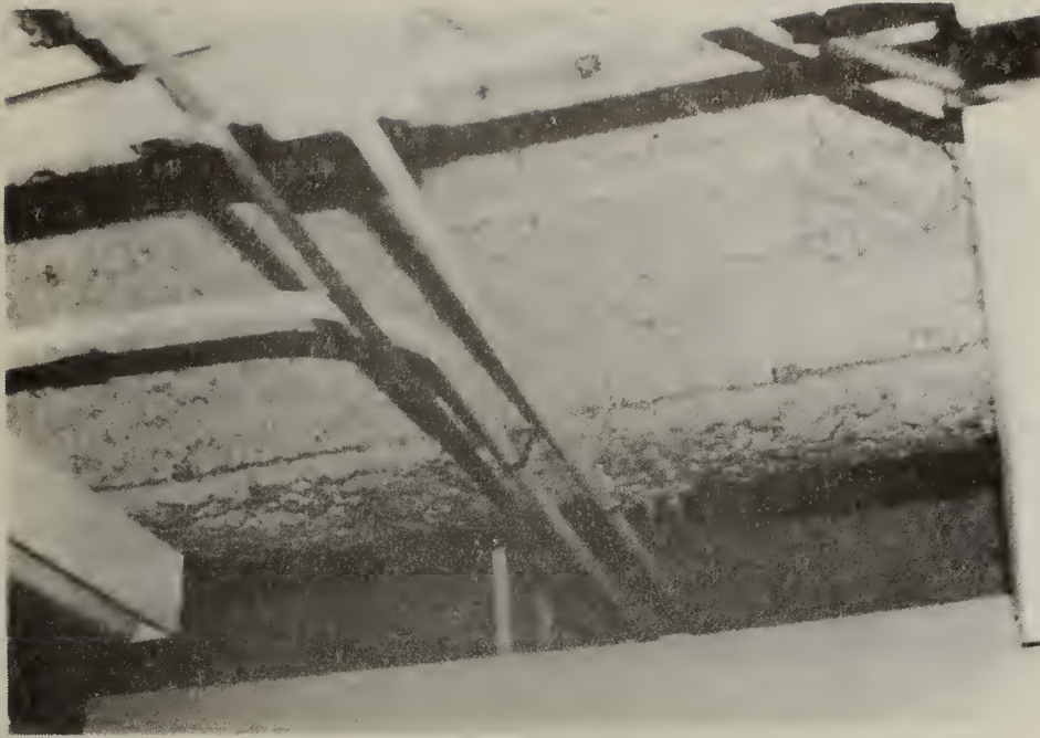
Figure 2.11 Damage to fireproofing on structural steel due to electrical system modifications
