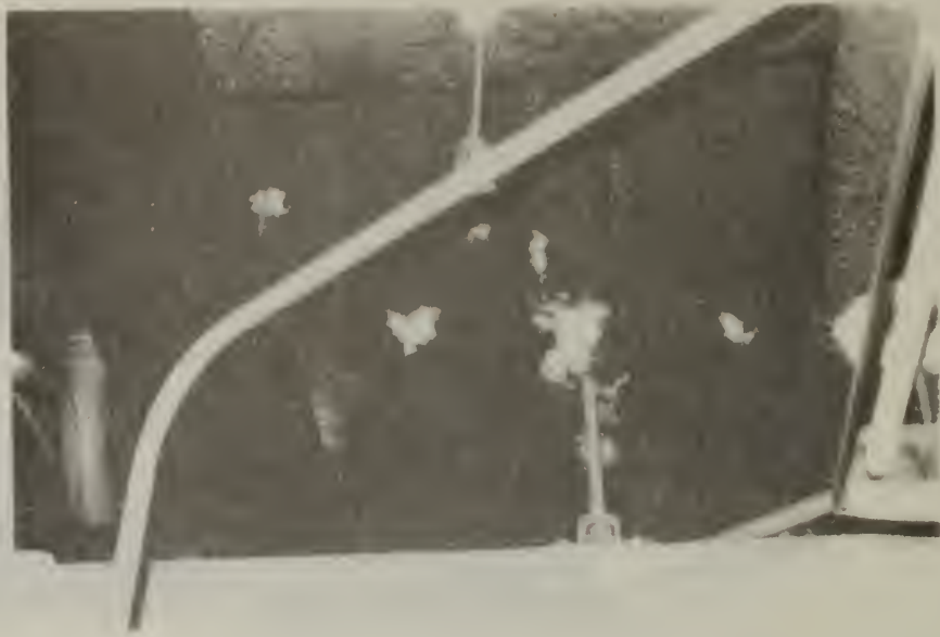
Figure A.15. Room 18204 - ceiling of zone 2 elevator control room showing patching of fireproofing during electrical and plumbing modifications
