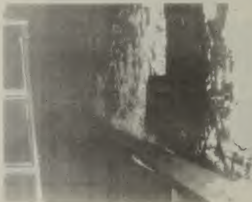
Figure A.8. Zone 3 elevator hoist room adjacent to roof - fireproofing removed from beam
