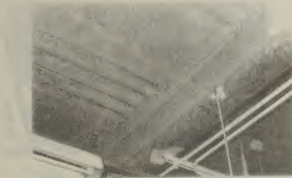
Figure A.13. Room 12207 - ceiling of zone 1 elevator machine room showing patching of fireproofing damaged during installation of hangers for ductwork
