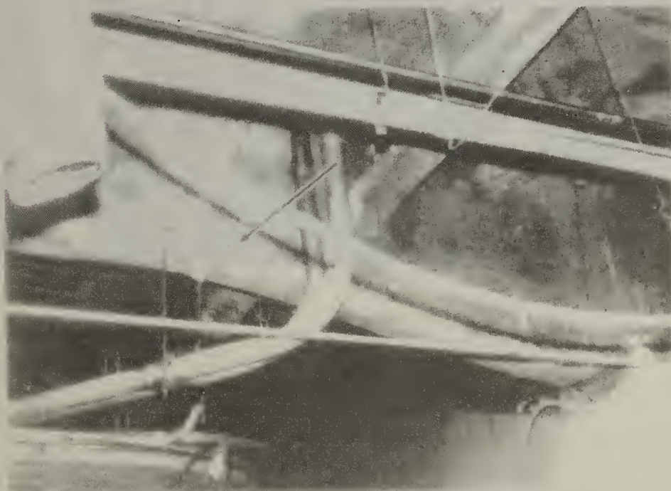
Figure 6. Damage to fireproofing due to renovation of plumbing system in Room 15219
