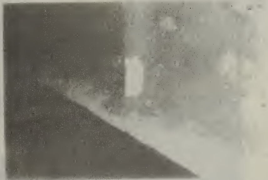
Figure A.14. Crawl space for courthouse ventilation off plenum stairwell #1 - patching of fireproofing following physical damage
