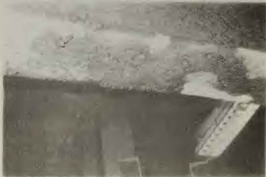
Figure A.16. Room 18204 - beam in zone 2 elevator control room showing patching of fireproofing
