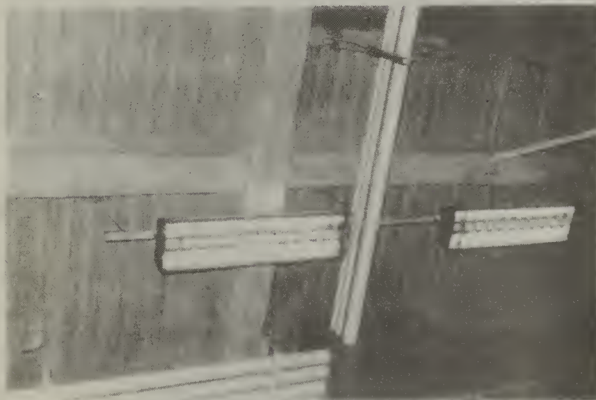
Figure A.6. Room 20408 - ceiling of electrical substation with no apparent damage to fireproofing
