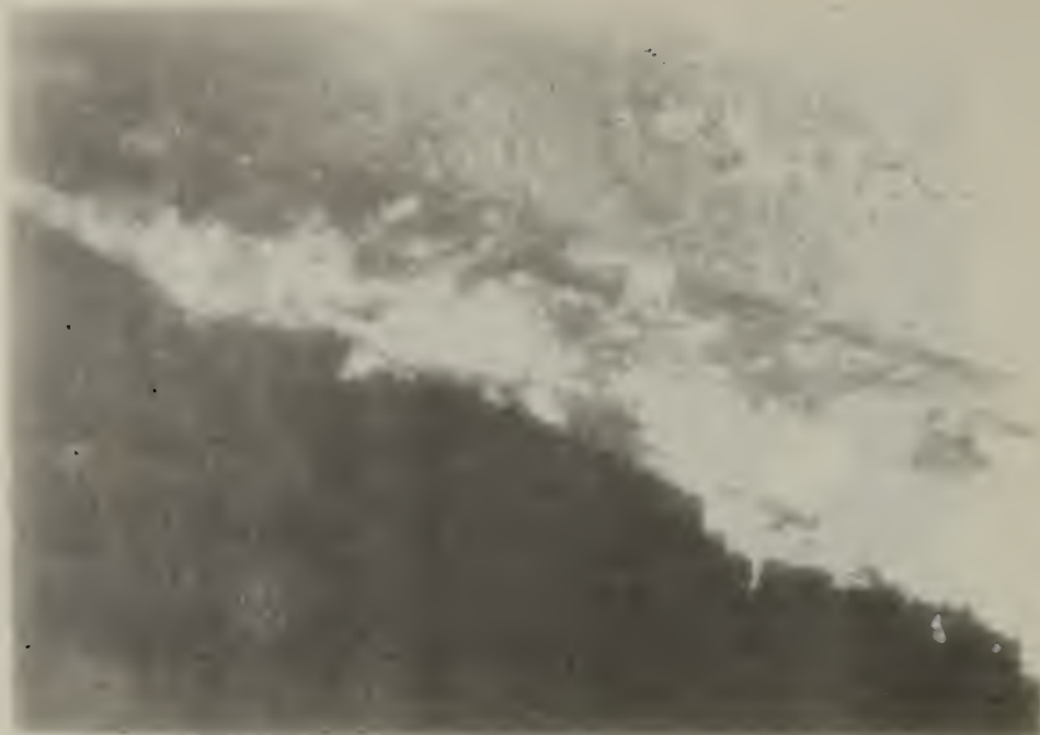
Figure A.7. Zone 3 elevator hoist room adjacent to roof - physical damage to fireproofing on beam caused by roofing contractor.
