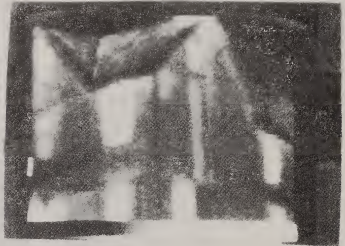
Figure 2.19 Example of an exterior thermogram of a retrofitted dwelling. Notice the missing insulation in a bay cavity and the abnormally warm roof.
