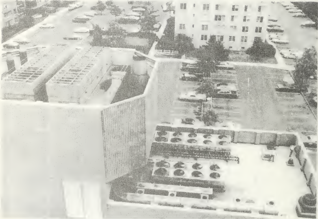
Figure 2.17 The central equipment building roof showing the cooling towers and the dry coolers for control of PHW and engine lubricating oil temperatures
