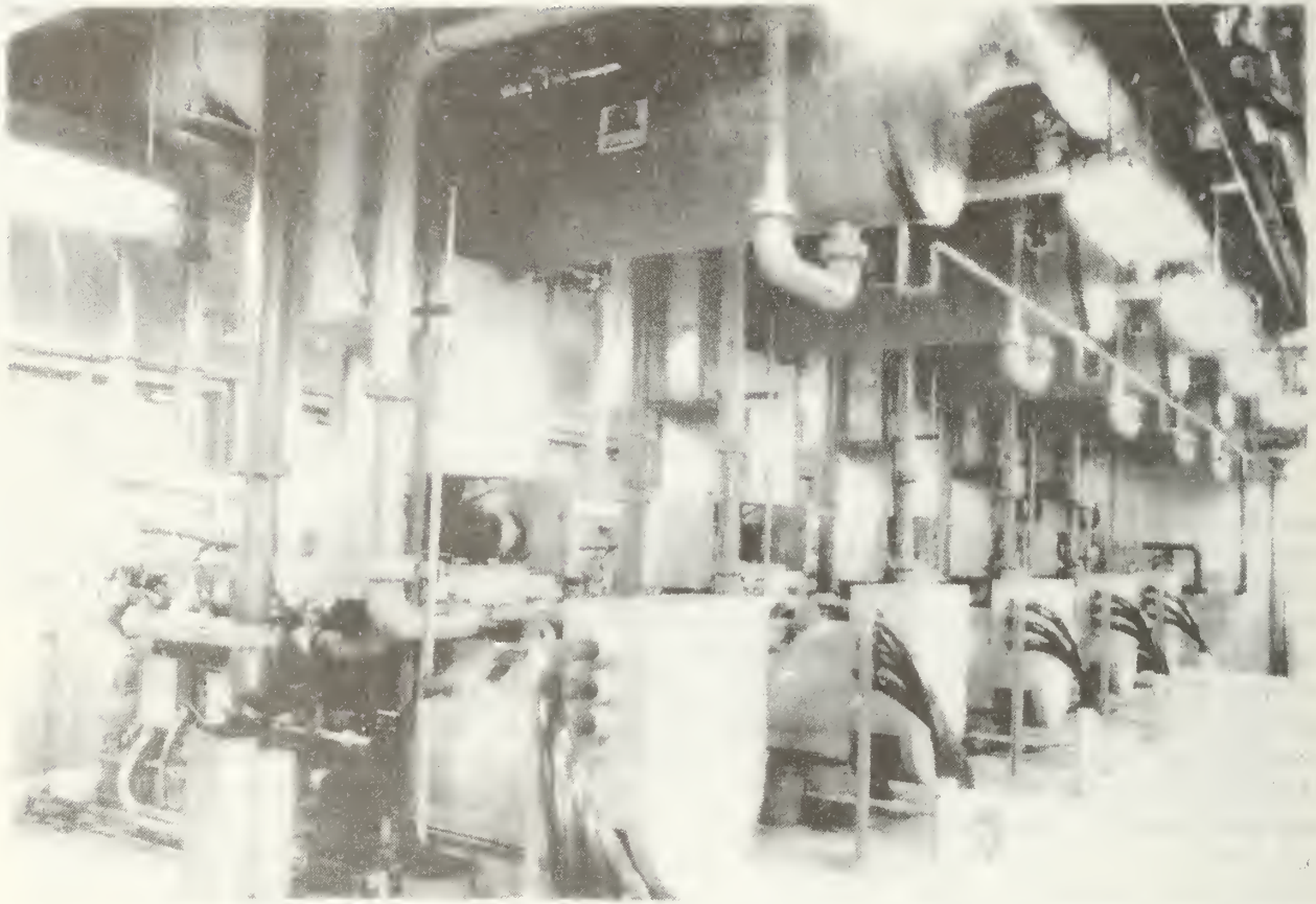
Figure 2.9 All five of the 600 kW engine-generators
