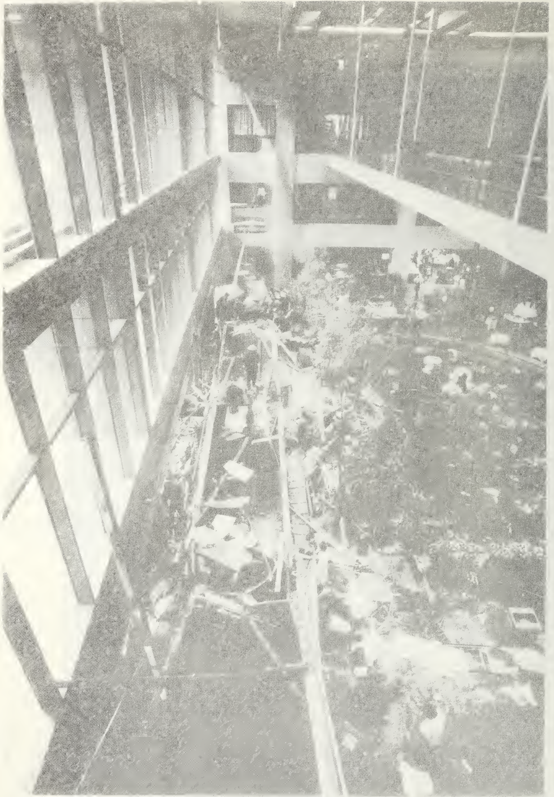
Figure 4.2 Walkways shortly after the collapse. View is directly to the north along the axis of the walkways. Span U7-8 is in foreground and third floor walkway is at upper right. Water is coming from broken sprinkler pipes. Photo by Greg Smith, reprinted by permission of The Kansas City Times , © 1981, The Kansas City Star Company.
