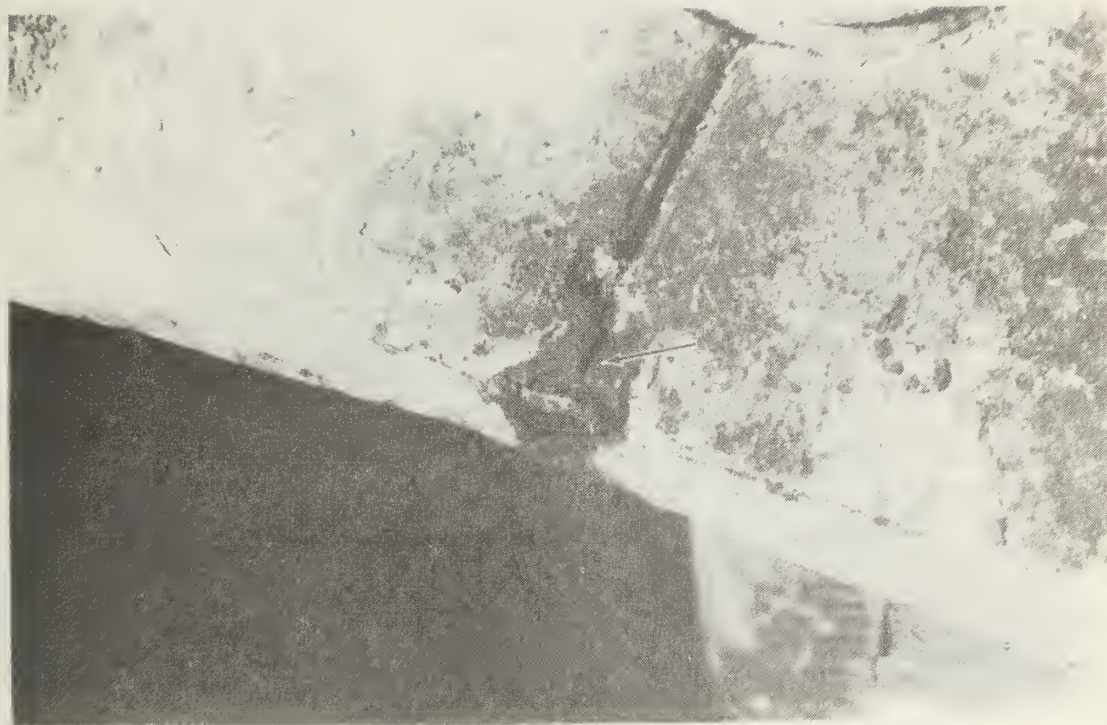
a) Location 8MW. Tack weld crack.
