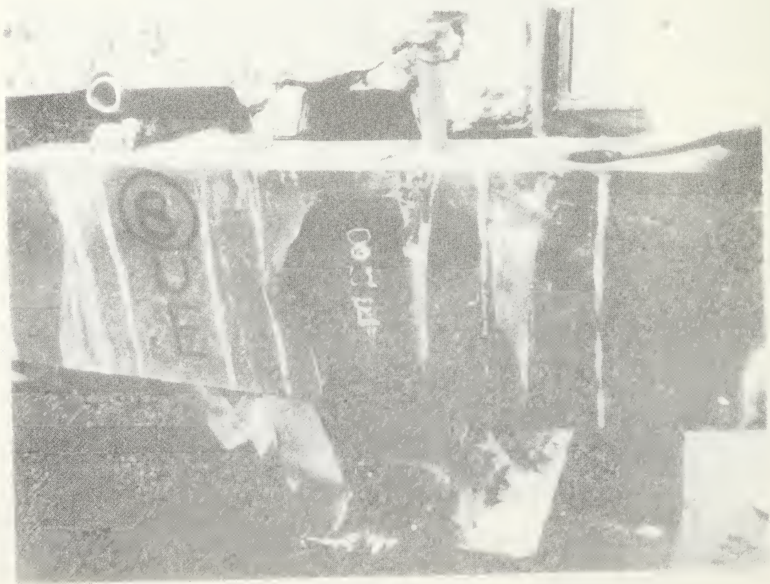
Figure 5.24 Tear in box beam web at location 8UE.
