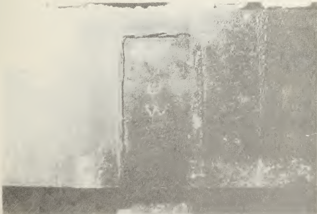
Figure 5.22 Shear failure in clip angle fillet weld at location 9UW, north side. This weld and the corresponding weld at location 9LW did not show evidence of a pull-out (tensile) failure at the top fillet weld.
