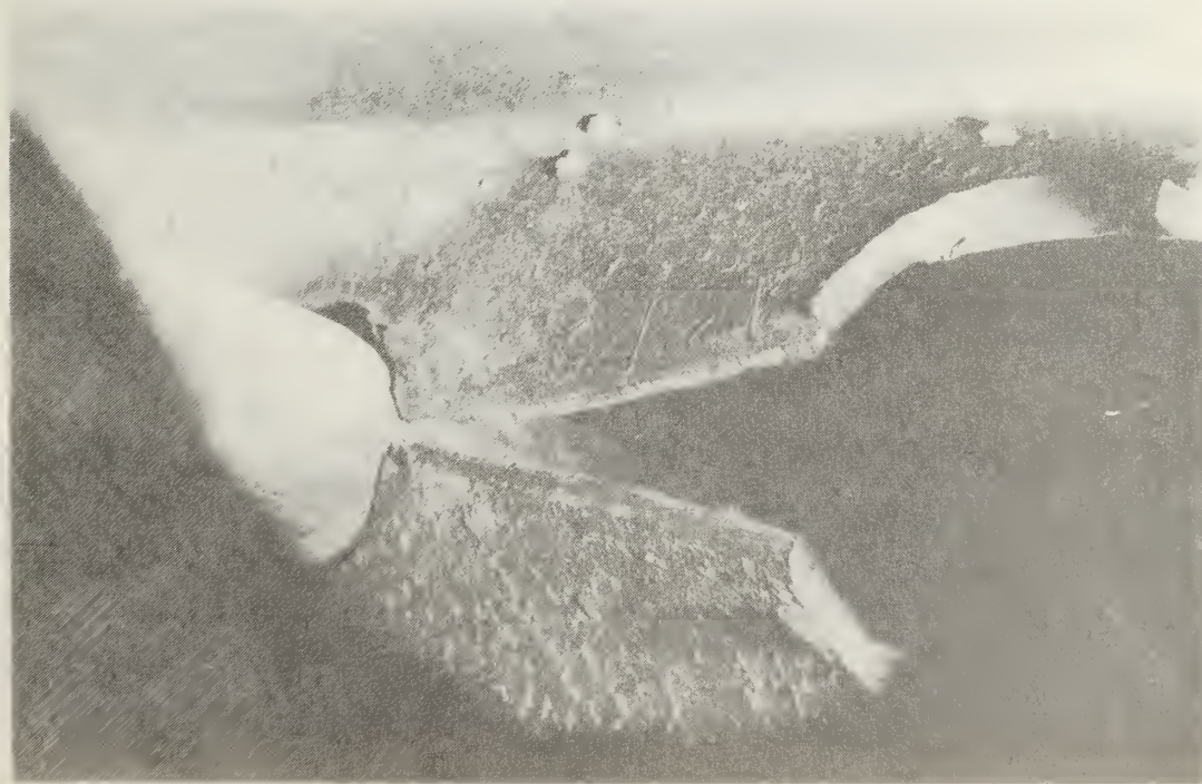
Figure 5.16 Fracture through the weld at location 9UE, lower flange. Weld porosity denoted by arrows.
