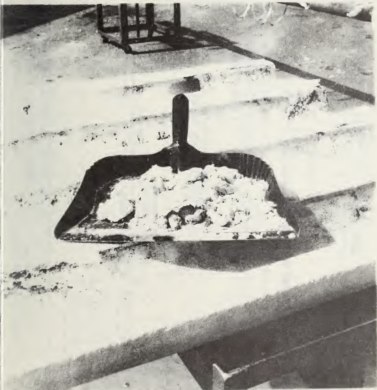
Figure 36. Crumbs of KAYLO-10 insulation found in the conduit space after the carrier pipe and insulation jacket were removed.
