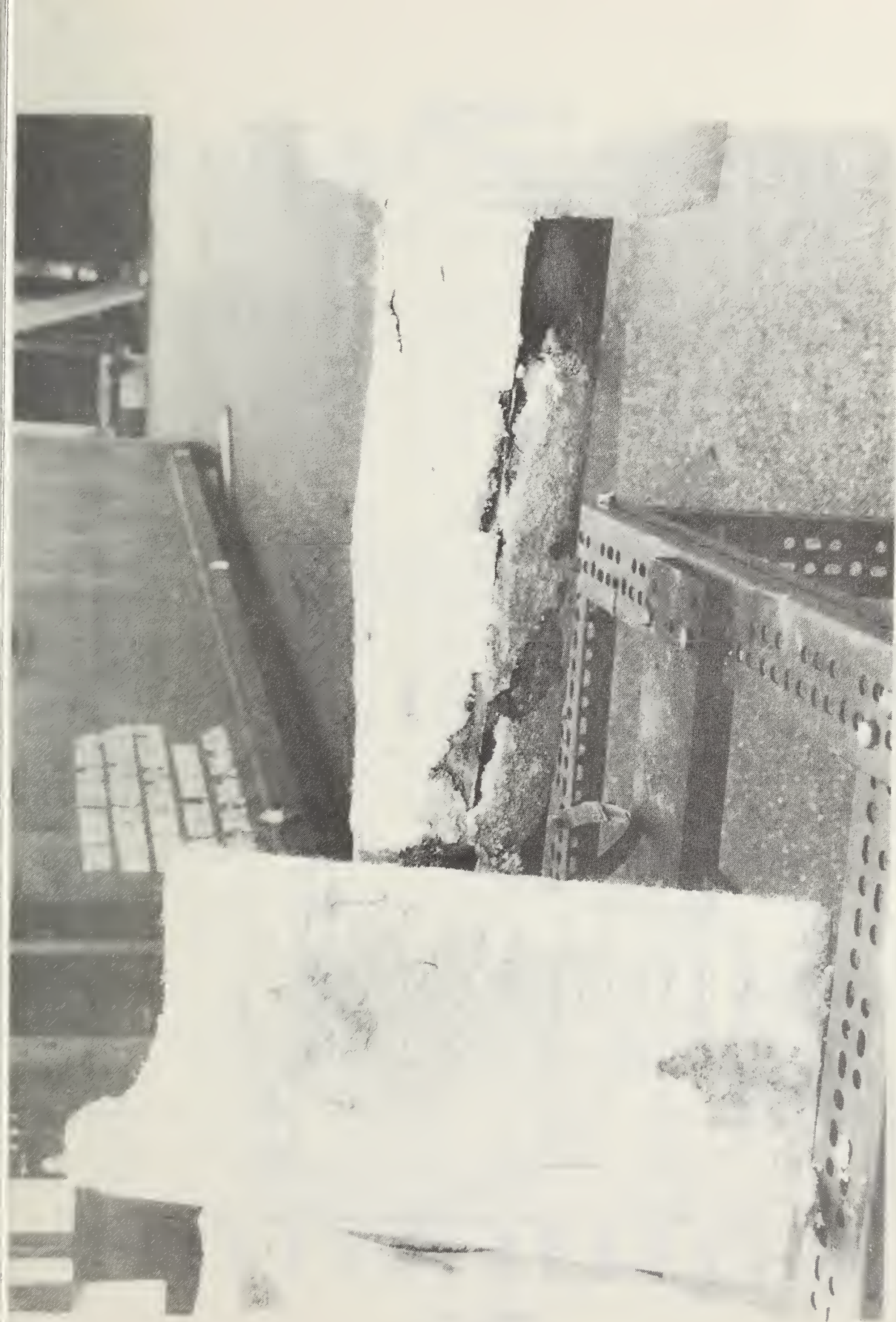
Figure 50. Condition of Wesolite after removal from pipe after boiling.
