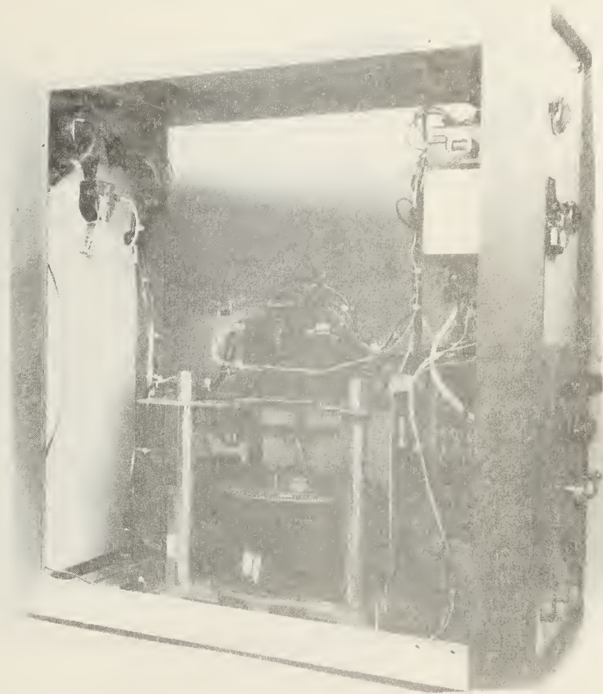
FIGURE 17. Interior View of the Generator Input Unit (left side looking toward rear)
