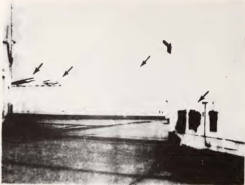
Figure 20 -- Nose Dock, MacDill AFB, Delamination of Elastomeric Coating (indicated by arrows).
