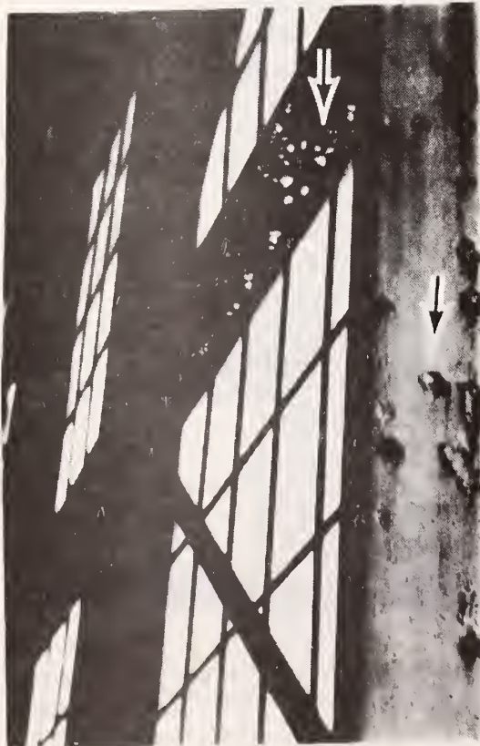
Figure 25 -- Steel Support Beams, Patrick AFB (arrows indicate areas of steel corrosion).
