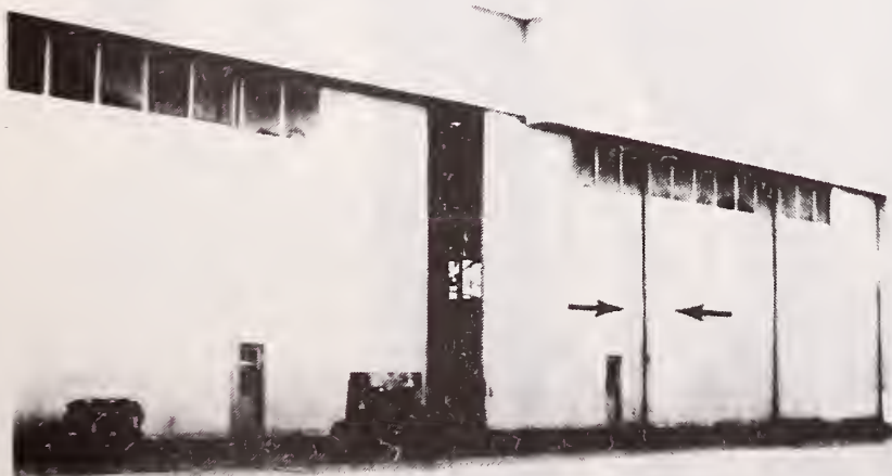
Figure 23 -- Hanger Doors, Tyndall AFB (arrows indicate area shown as close-up in Figure 24).
