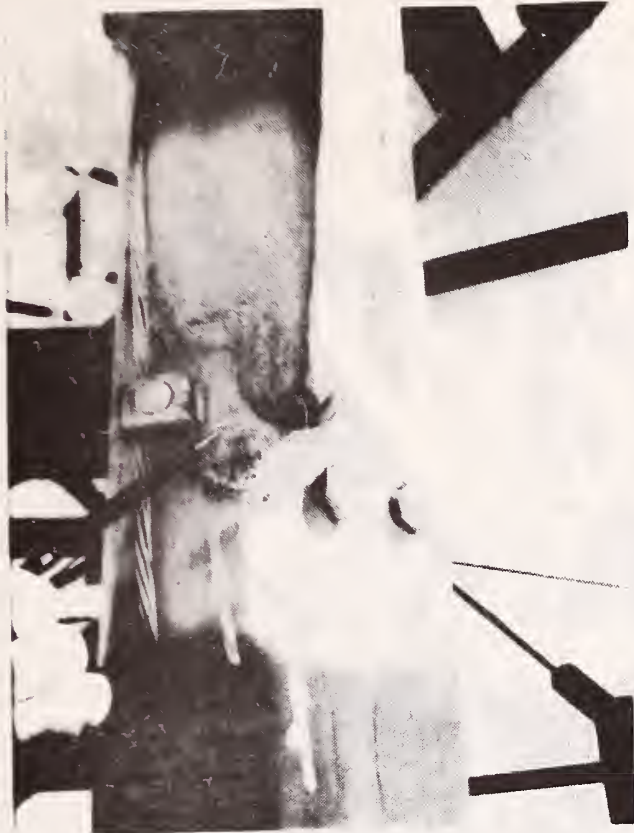
Figure 34 -- Communication Tower, Tyndall AFB.
