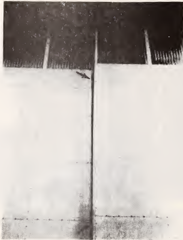
Figure 24 -- Hanger Doors, Tyndall AFB, Detail of Unpainted Area of Door Overlap (indicated by Arrows)
