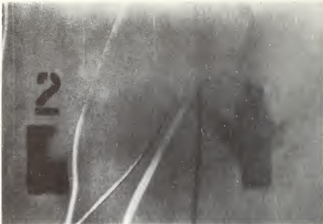
Figure 42. Test FE 1 - Smoke coming out of AC (2) insulated and NM uninsulated (3) switches
