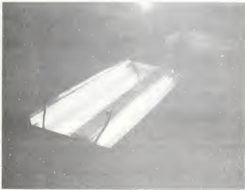
Because of biohazards, light fixtures in the laboratories must be serviced from the mechanical space above.
