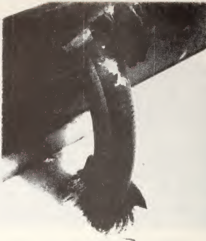
Figure 2-35. Uninsulated Flexible Coupling
