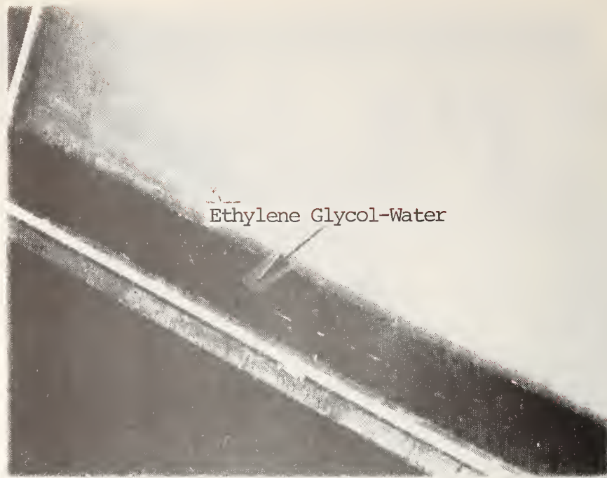
Figure 2-19. Leaking Aluminum Absorber Plate
