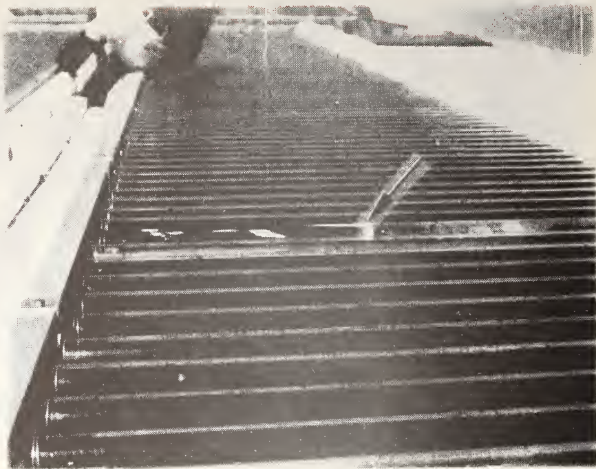
Figure 2-31. Evacuated Tube Breakage
