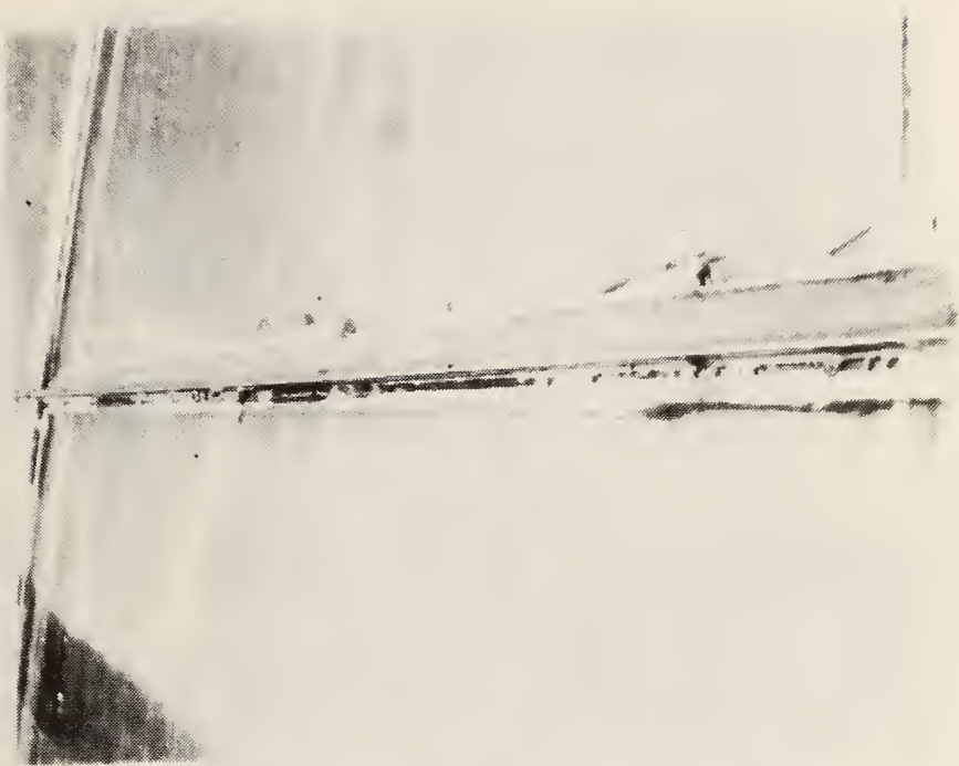
Figure 2-9. Undersized and Improperly Bedded Tempered Glass Cover Plates
