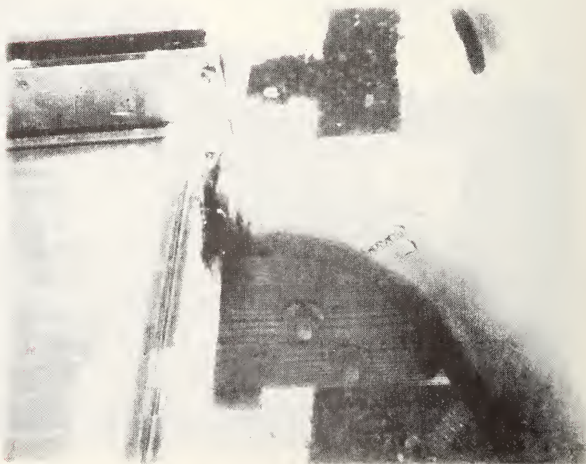
Figure 2-36. Surface Cracking on Cellular Insulation
