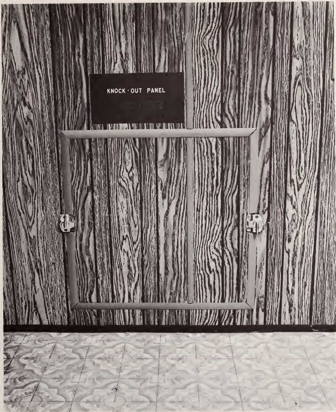
Figure 8. Demonstration Unit. Knock-out panel
