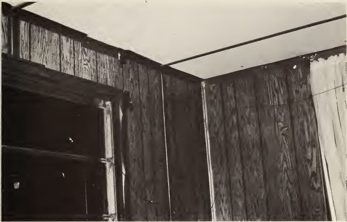
Figure 45. Panel side joints, wall corner joint, ceiling wall joints and window sealed with duct tape.
