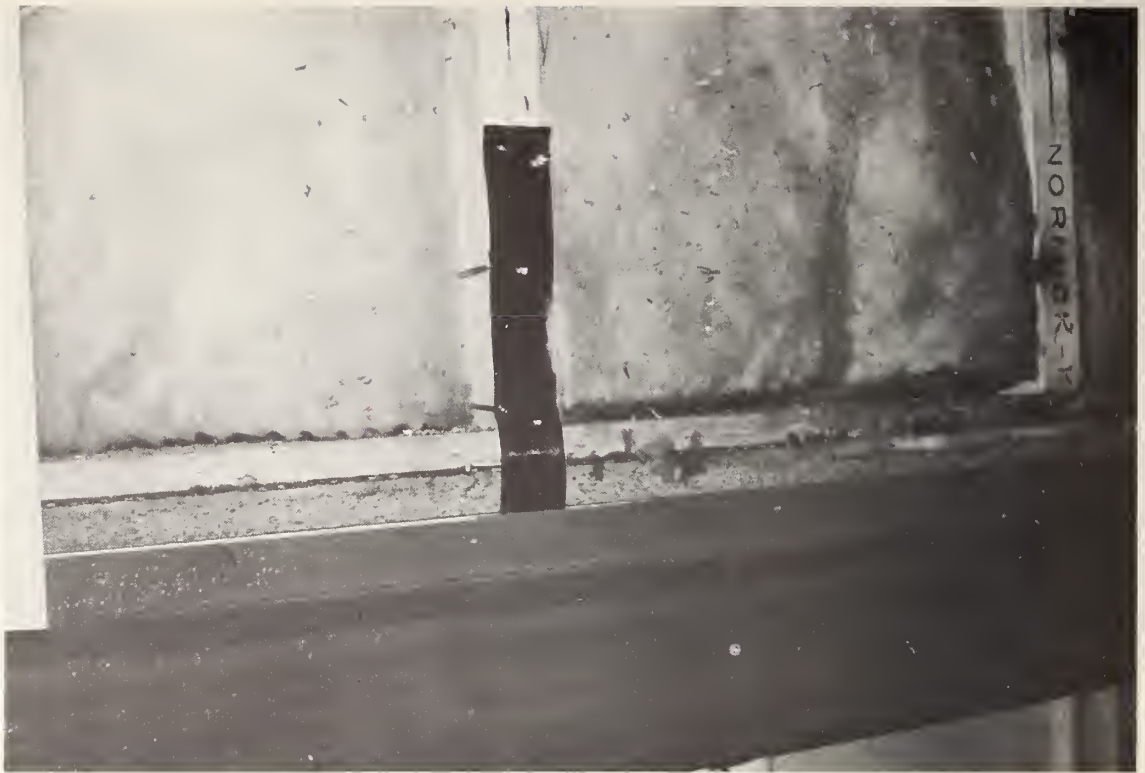
Figure 31. Gap between sill plate and bottom of insulation which could allow outside air in contact with back of inside paneling.
