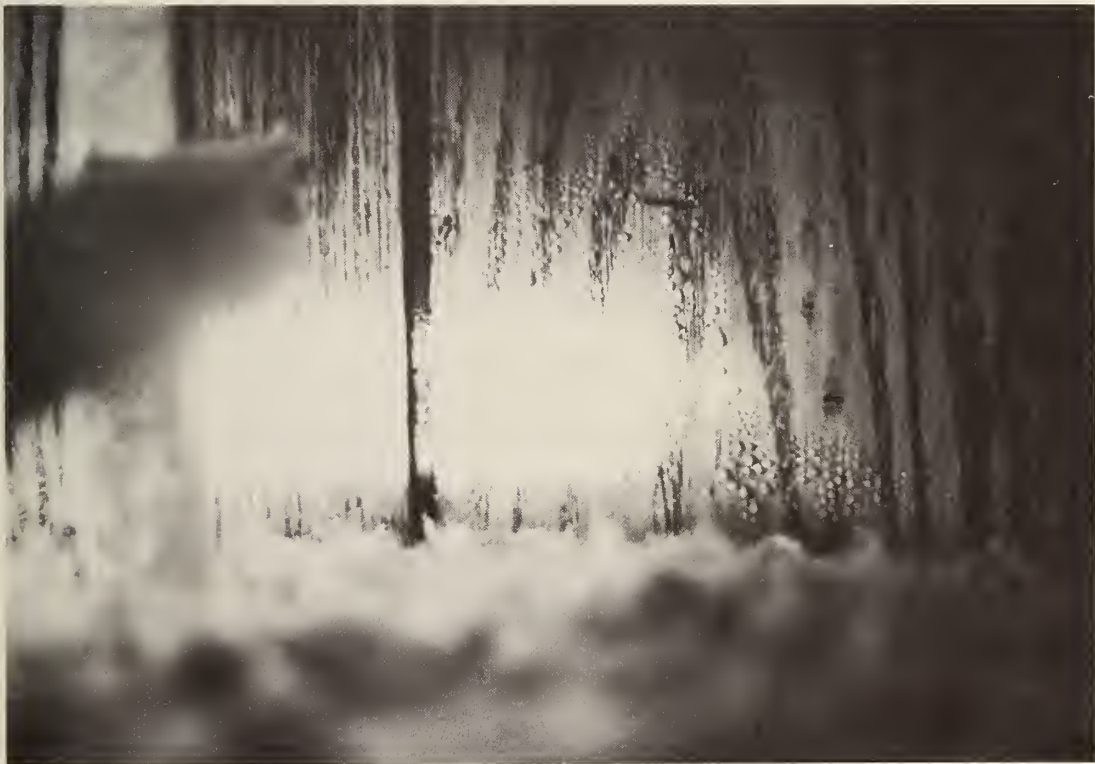
Figure 53 . Surface moisture condensation at base of wall.
