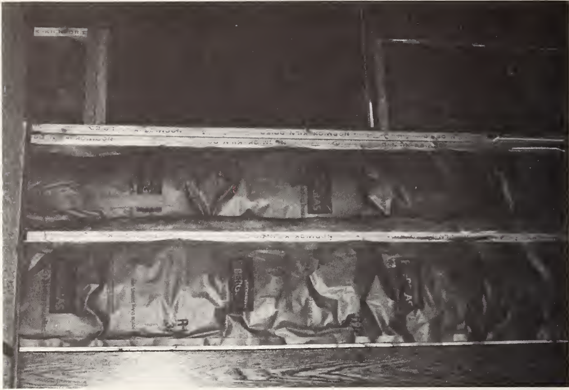
Figure 35. Inside of mobile home wall with paneling removed. Original R-7 batt insulation has been replaced with R-11 batt. Insulation friction fit.
