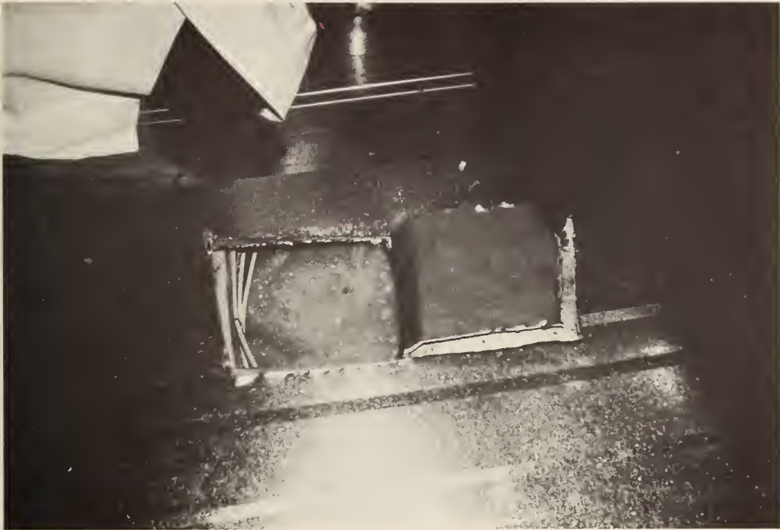
Figure 50 Roof test cut number 3 showing water and ice on bottom surface of sheathing and water droplets on top surface of roof insulation.
