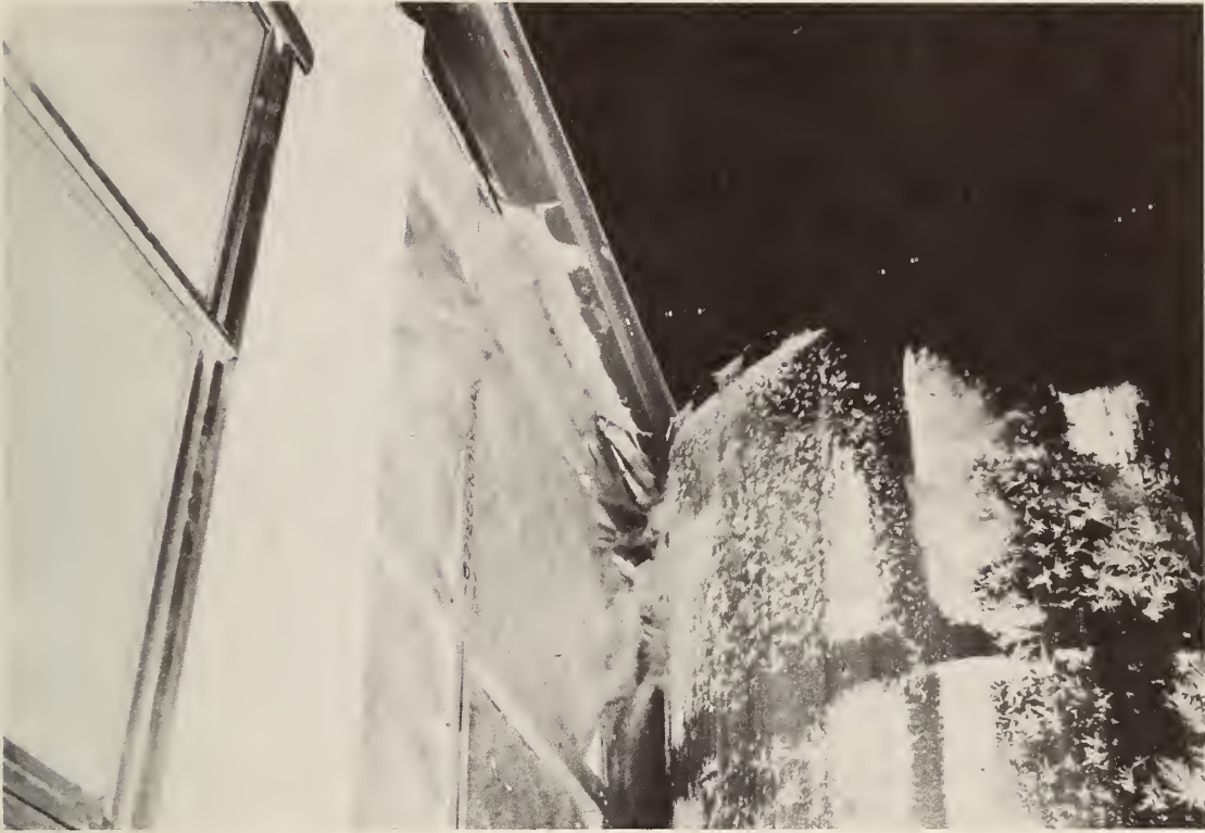
Figure 52 . Frost accumulation at top of wall and under fascia.
