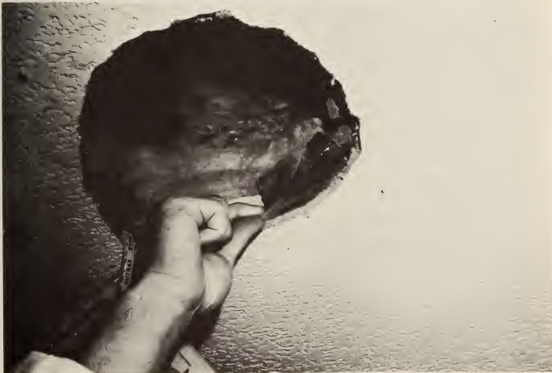
Figure 51 Location of water found on top of plastic film vapor barrier of bathroom exhaust.
