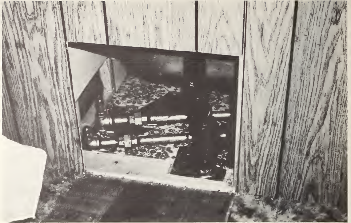
Figure 47. Plumbing hole through floor under bathtub sealed with duct tape. Access gained through hole cut in end bedroom wall.
