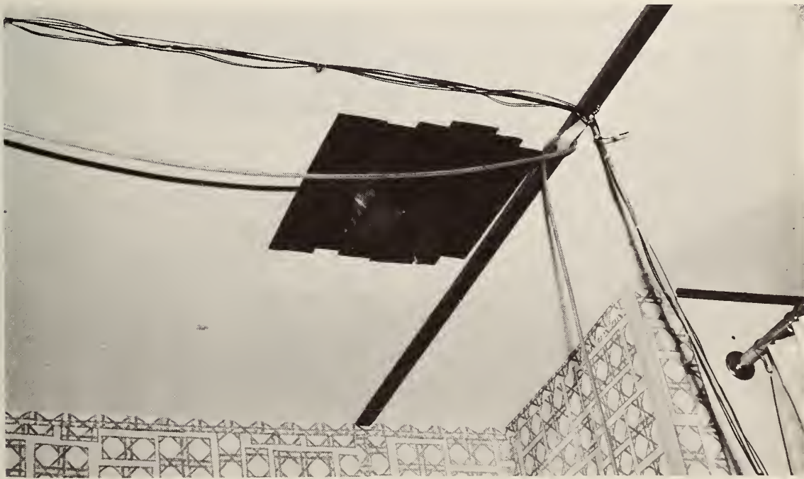
Figure 46. Bathroom exhaust fan sealed shut with duct tape.
