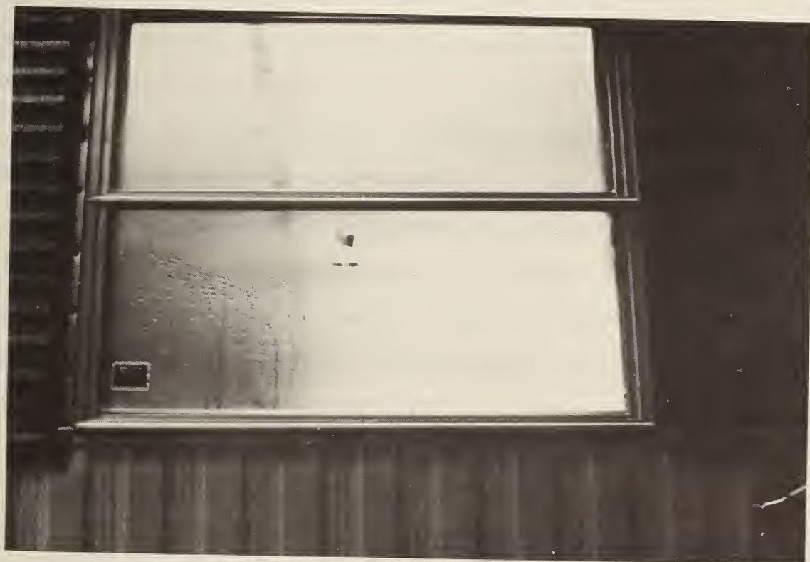
Figure 55. Typical window condensation.
