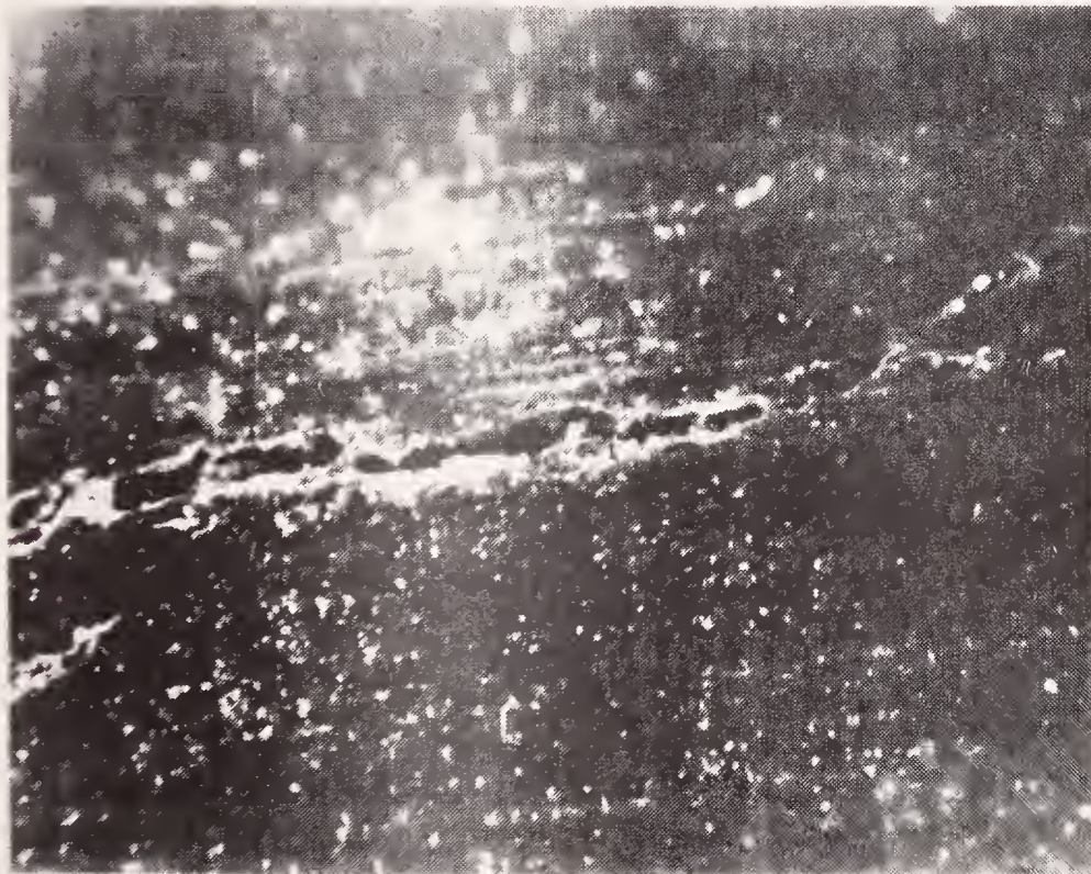
Figure 20. Large crack in the polyurethane jacket of transducer MILES 96R-1 located at Griffis Air Force Base.
