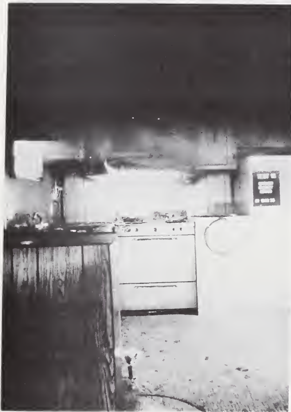
Figure 9. Illustrates the Extent of Involvement of a Cabinet With a Metal Range Hood (Time: 2 min-20 s)
