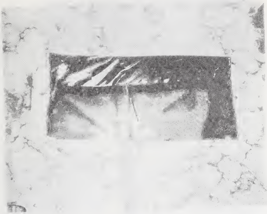
Figure C-86 Riser From Heat Duct in Floor to Register Constructed of Fabric Material.
