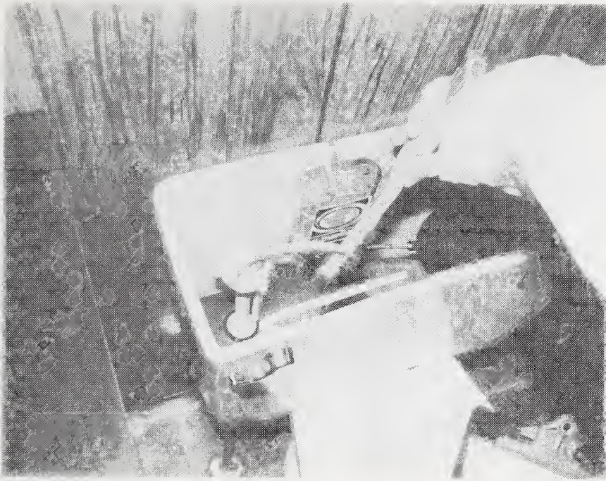
Figure C-78 Submerged Valve Flushing Device Which Could Allow Flush Tank Water to Back Flow Into The Potable Water Supply
