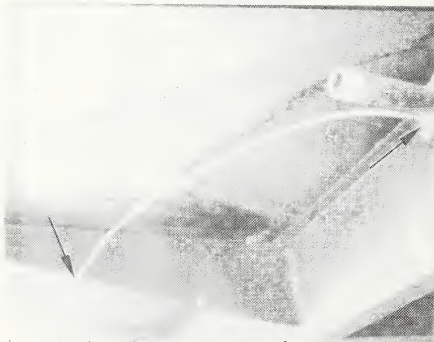
Figure C-85 Improper Grounding of Gas Supply Pipe to Mobile Home Frame
