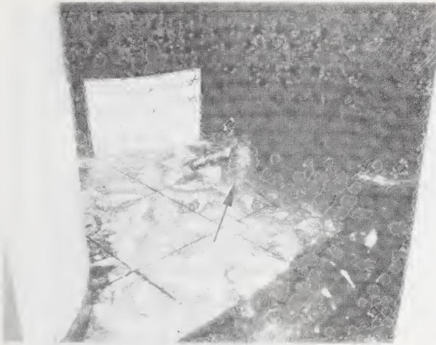
Figure C-52 Notching of Floor Joists for Passage of Plumbing Piping
