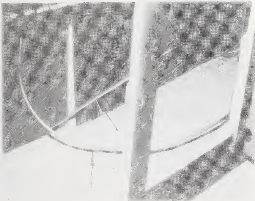
Figure C-68 Example of Poor Workmanship - Excessive Amount of Water Supply Piping Used Under Kitchen Sink
