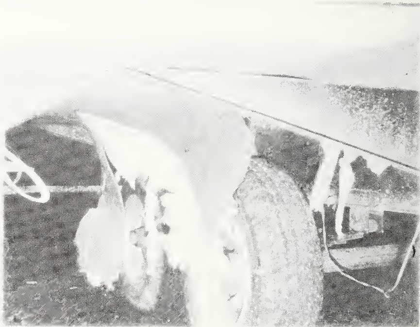
Figure C-44 Damage to Bottomboard on Underside of Mobile Home Exposing Floor Insulation Resulting in Diminished Rodent Resistance and Excessive Air Infiltration.
