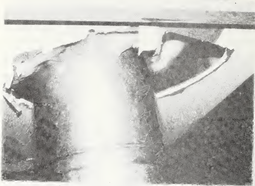
Figure C-91 Example of Poor Workmanship - Hole Cut Through Ceiling for Passage of Furnace Vent
