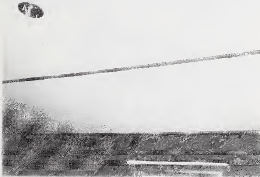
Figure C-11 Water Damage to Ceiling Due to Rain Leak at Roof Membrane Joint
