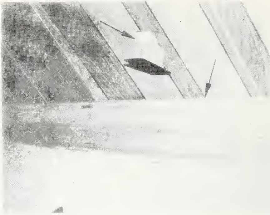
Figure C-69 Plumbing Pipe Running Along Inside Wall in Sleeping Quarters Covered With Lightweight Plastic Cover. Also, Electrical Box Inadequately Attached to Wall
