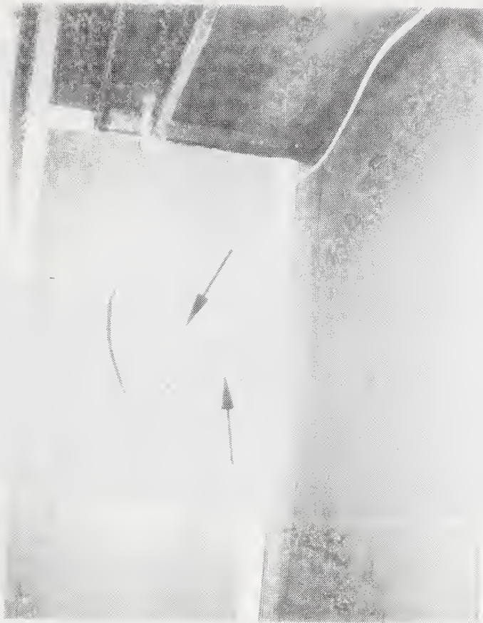
Figure C-101 Cable Inadequately Supported and Exposed in Bedroom Closet.
