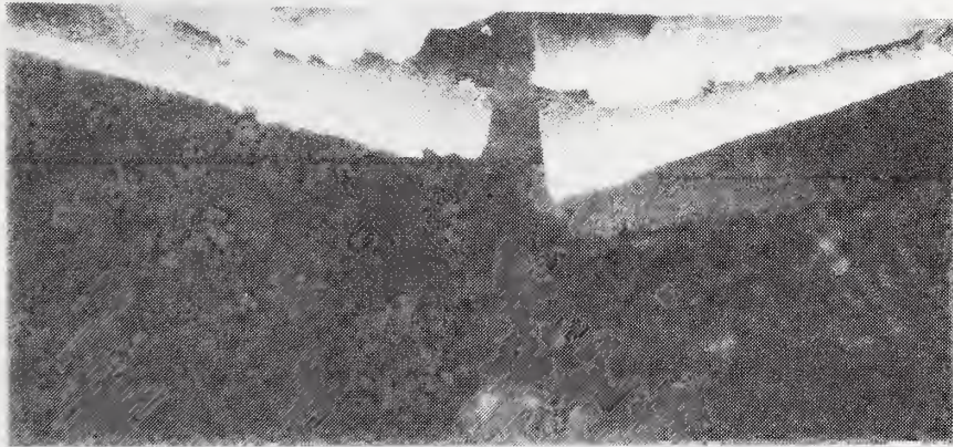
Figure C-49 Failure of Fastening of Bottomboard to Underside of Mobile Home
