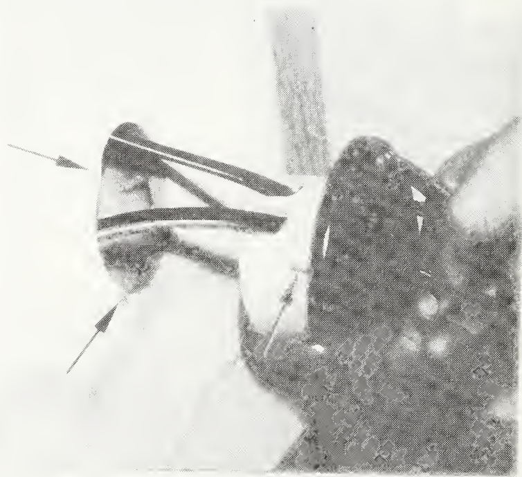
Figure C-96 Ceiling Fixture Inadequately Attached to Vegetable Fiberboard Ceiling Material.
