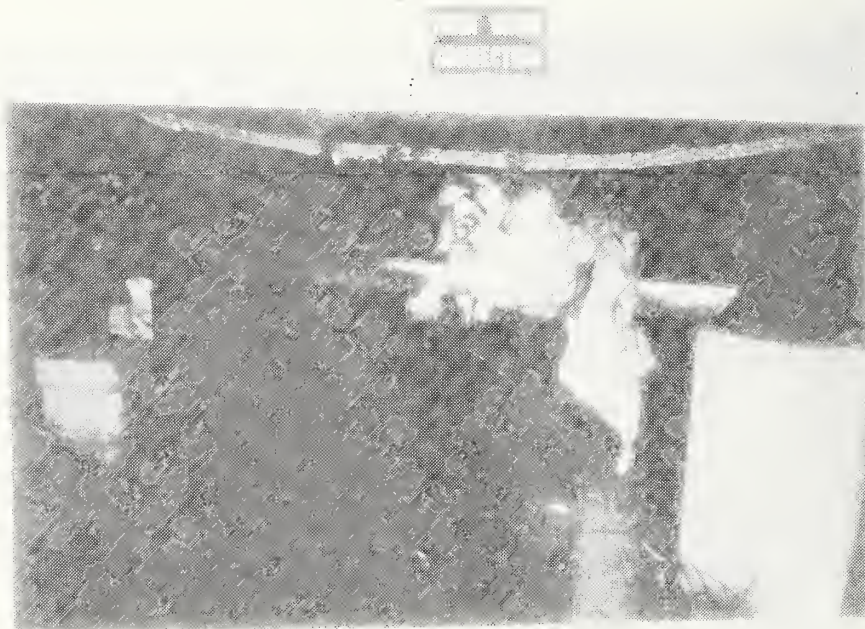
Figure C-48 Failure of Fastening of Bottomboard to Underside of Floor.
