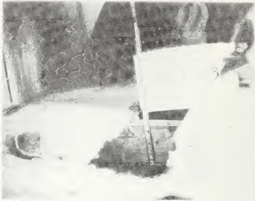
Figure C-43 Buckling of Particle Board Floor Decking Due to Water Damage Caused by Plumbing Malfunction
