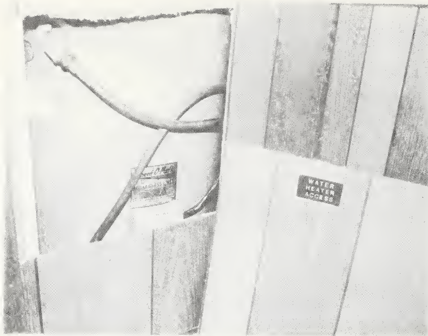
Figure C-80 Inadequate Hot Water Heater Access From Within Closet. Wall Paneling Would Have to be Removed to Replace Hot Water Heater
