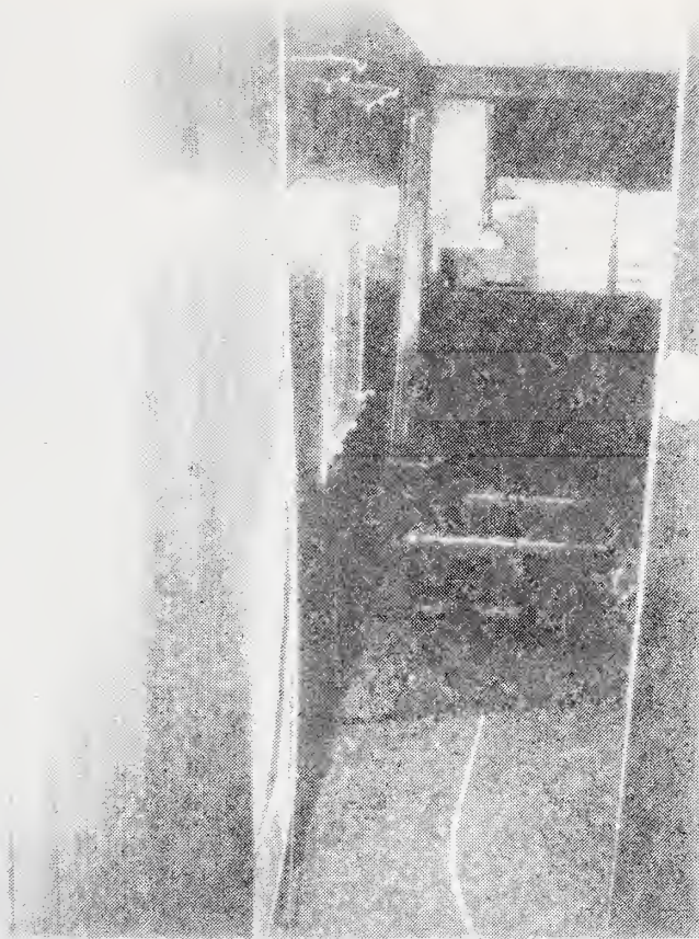
Figure C-7 Buckled Interior Wall Paneling on Exterior Wall Due to Water Penetration of Exterior Skin.
