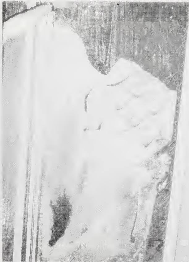
Figure C-53 Exterior Door Construction of Paper Honeycomb Core and Vegetable Fiber Board Skins. (This Mobile Home Had Been Abused and Experienced Exterior Water Damage)
