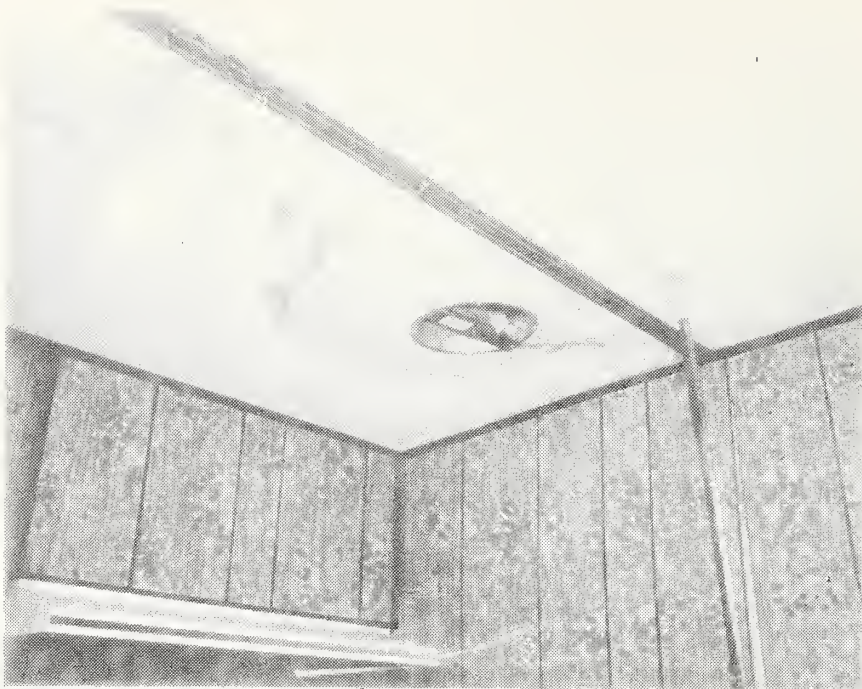
Figure C-12 Water Damage to Ceiling Due to Rain Leak at Vent Stack Penetration Through Roof
