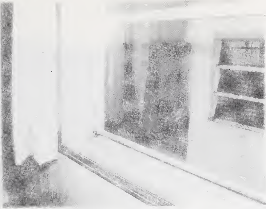
Figure C-56 Water Leak Through Closed Awning Type Windows (Interior Storm Windows)
