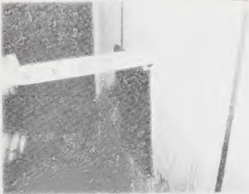
Figure C-97 Loose Receptacle Box Attached Only to Wood Paneling
