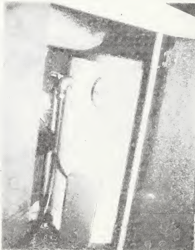
Figure C-81 Hot Water Heater Access Under Kitchen Cabinet. Kitchen Cabinetry would Have to be Removed to Replace Hot Water Heater
