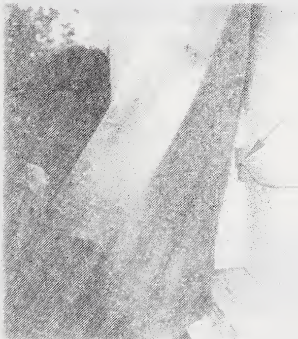
Figure C-8 No Insulation in Exterior Wall Stud Space and Unprotected Electrical Wire Running Through Notched Stud
