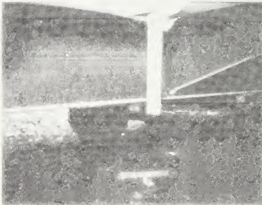
Figure C-62 Hot Water Heater Pressure Relief Overflow Pipe With Threaded End.
