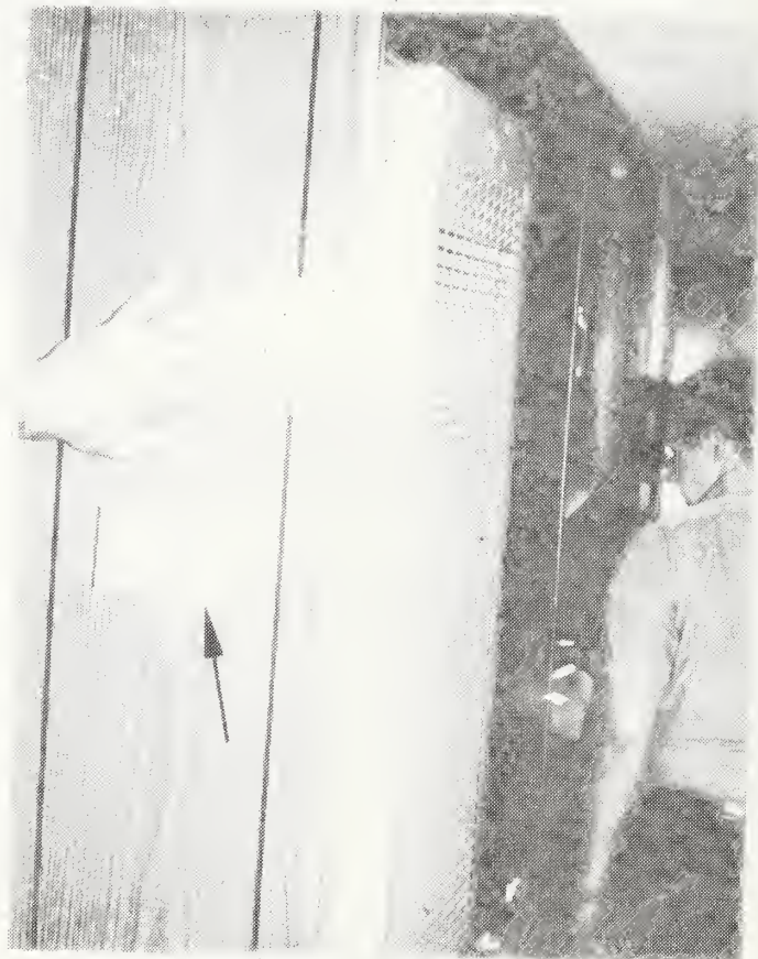
Figure C-92 Furnace Thermostat Located Adjacent to Furnace on Wall Common to Furnace Compartment Causes Problems of Temperature Control.
