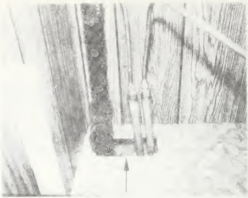
Figure C-50 Inadequate Rodent Resistance Due to Oversize Hole Cut for Passage of Plumbing Piping. No Attempt Was Made to Seal Holes.
