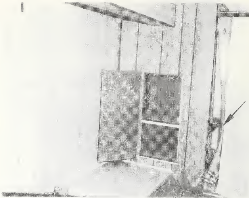
Figure C-32 Distortion of Shower Enclosure Wall Due to Effects of Moisture
