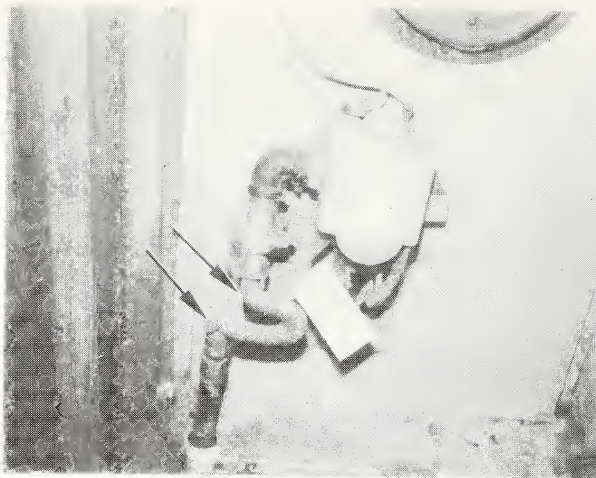
Figure C-84 Flexible Gas Connector on Furnace with Sharp Radius Bend
