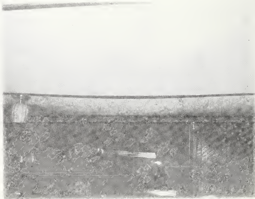
Figure C-21 Deflection of Ceiling Indicating Failure of Attachment to the Roof Truss
