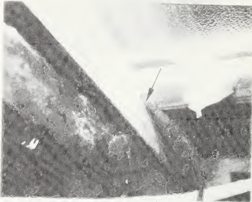
Figure C-103 Inadequate Electrical Cable Protection - Cable Wedged Between Wall Stud and Belt Rail
