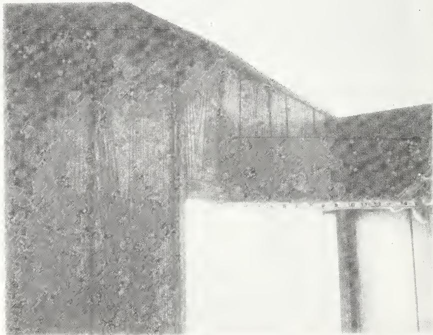
Figure C-55 Racked and Damaged Exterior Door Frame
