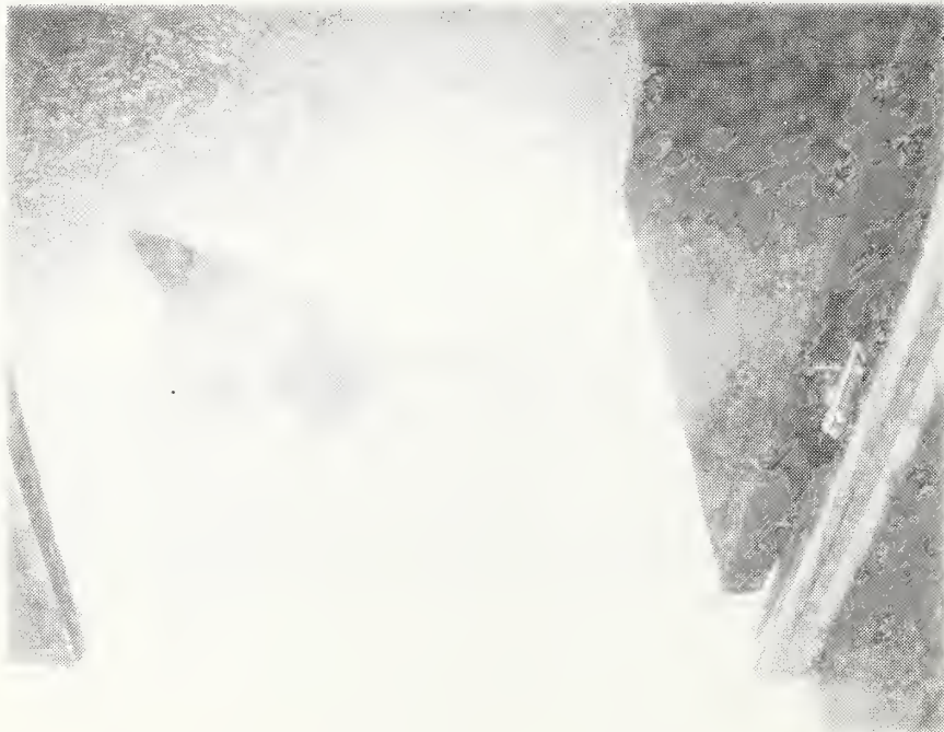
Figure C-40 Damaged Floor Covering at Entrance to Bedroom
