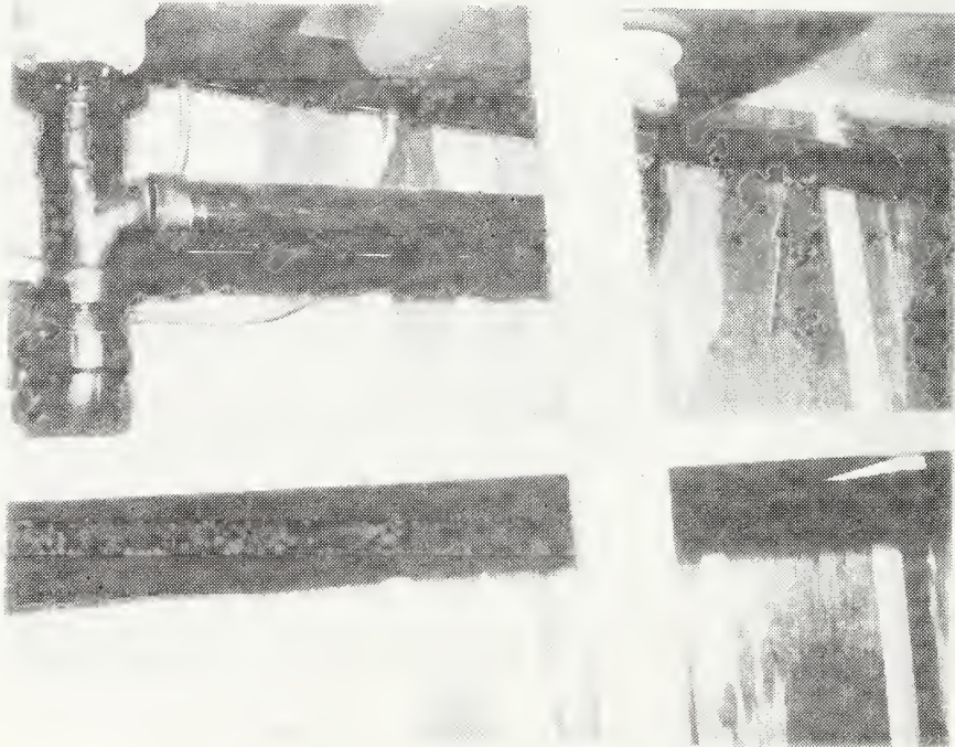
Figure C-74 Negative Slope of Vent Pipe Under Kitchen Sink
