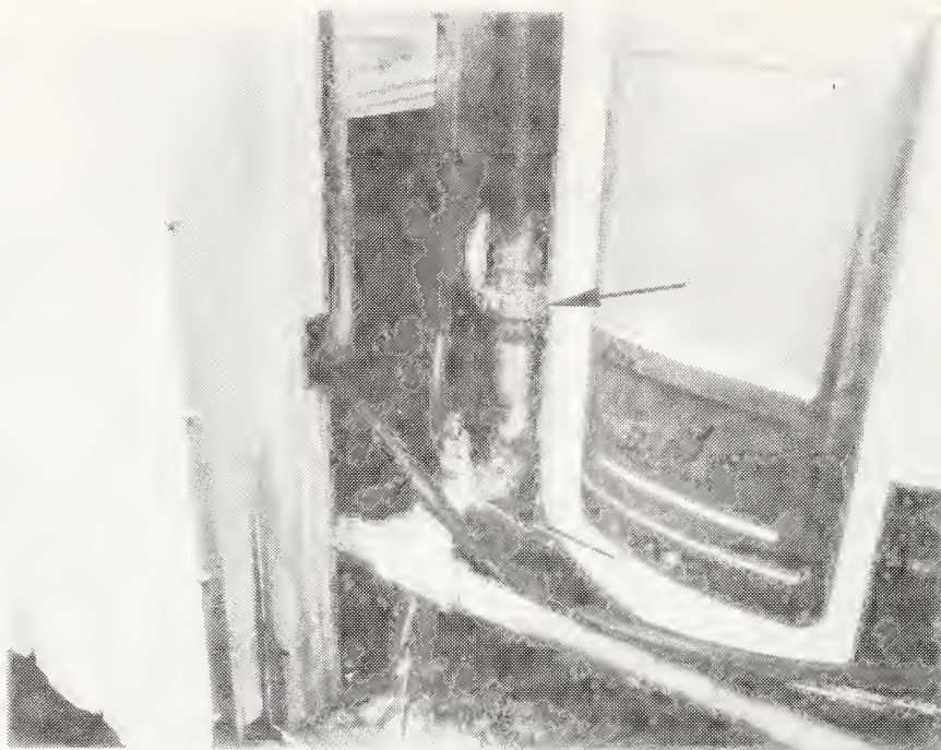
Figure C-65 Excessive Corrosion of Galvanized Steel Water Pipe in Hot Water Heater Compartment. Also, Electrical Cable Not adequately Supported
