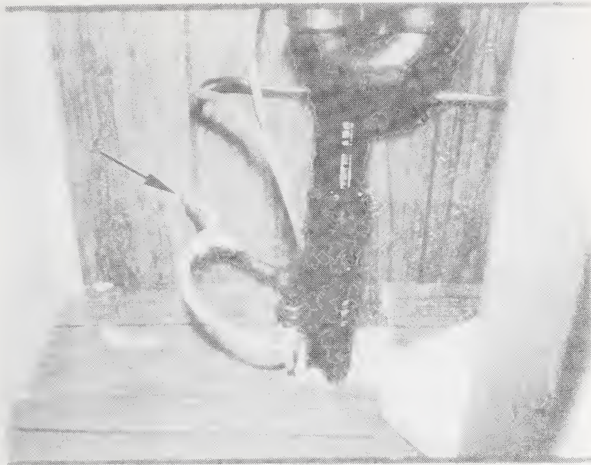
Figure C-67 Example of Poor Workmanship - Water Supply Piping and Electrical Wiring Passing Through the Same Undersize Wall Penetration
