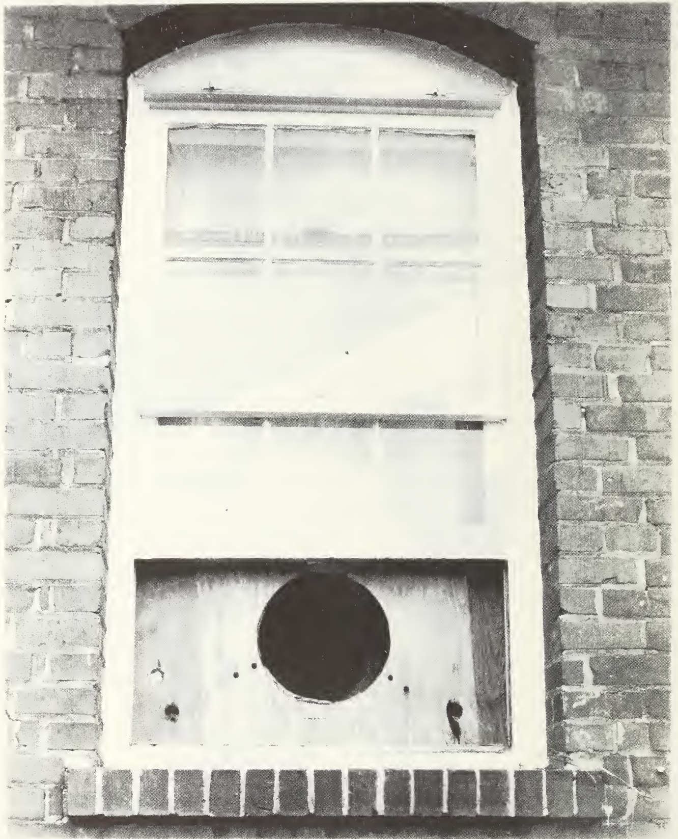
Figure 3B Flexible Duct Attic Ventilation Port
