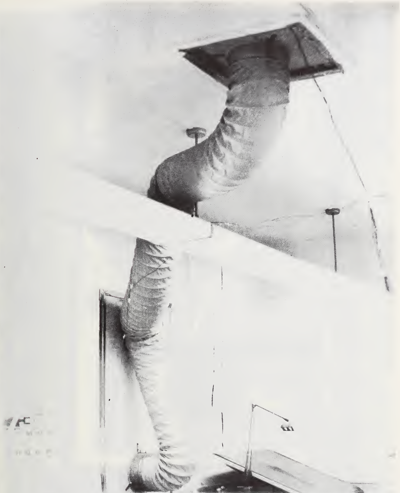
Figure 3A Flexible Duct Attic Ventilation System at the North End of Building 219
