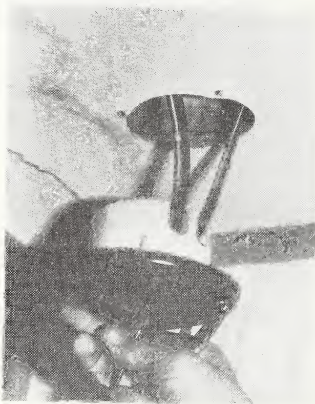
Figure 2 - Light Fixture in Area of Water Damage Pulled Loose from Ceiling
