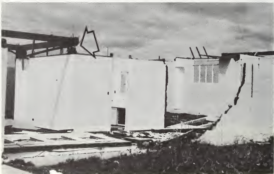
Figure 25 Wall and roof damage resulting from Typhoon Yoling, November 1970
