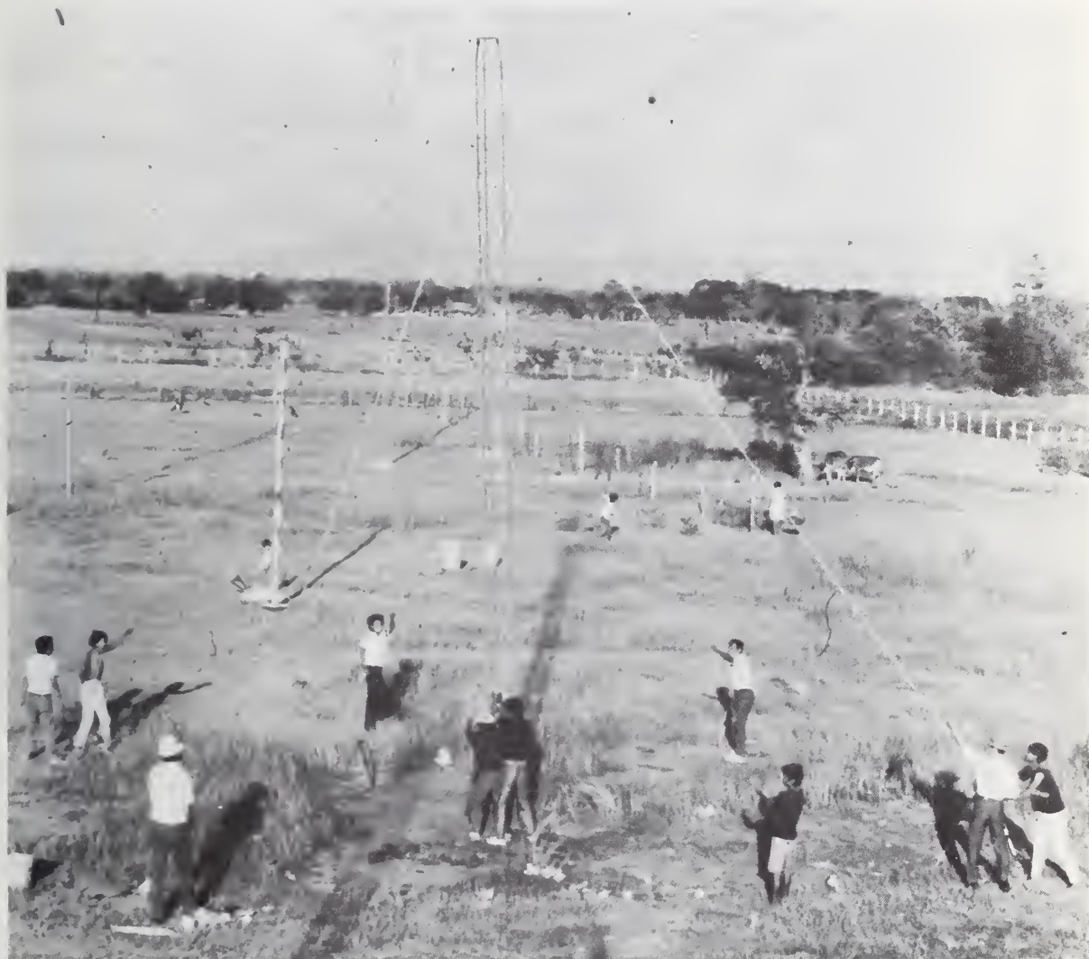
Figure 7 Erecting 10-meter meteorological tower which supports the anemometer and ambient pressure probe. Note guy wires running to ground anchors
