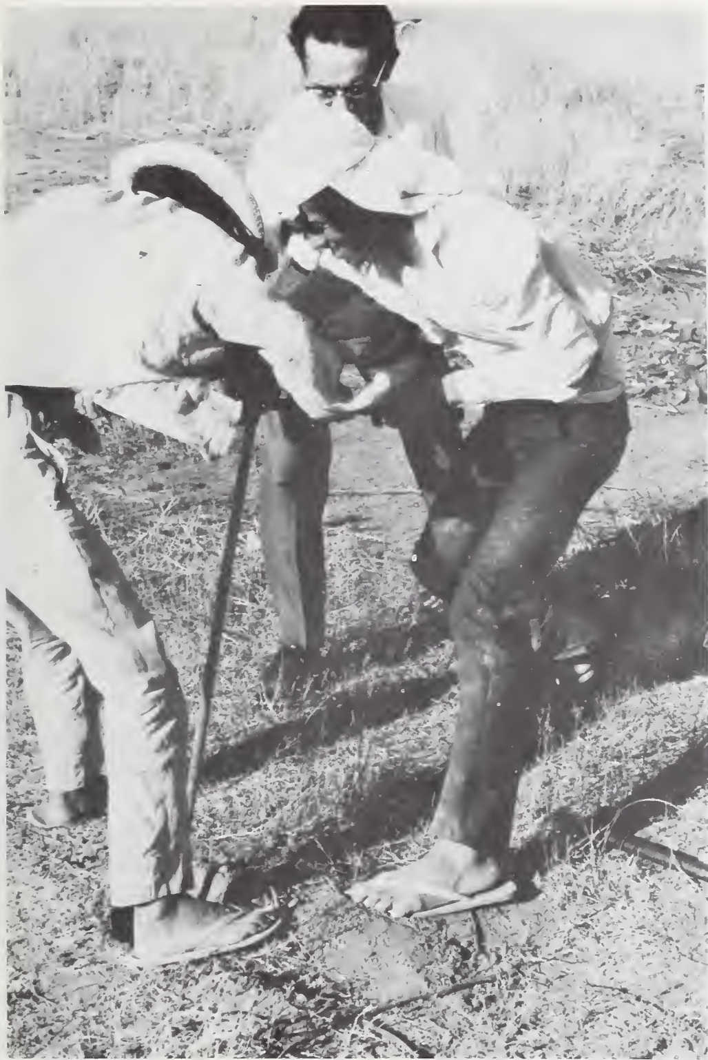
Figure 5 Typical installation of ground anchors by PAGASA technicians prior to erection of meteorological tower
