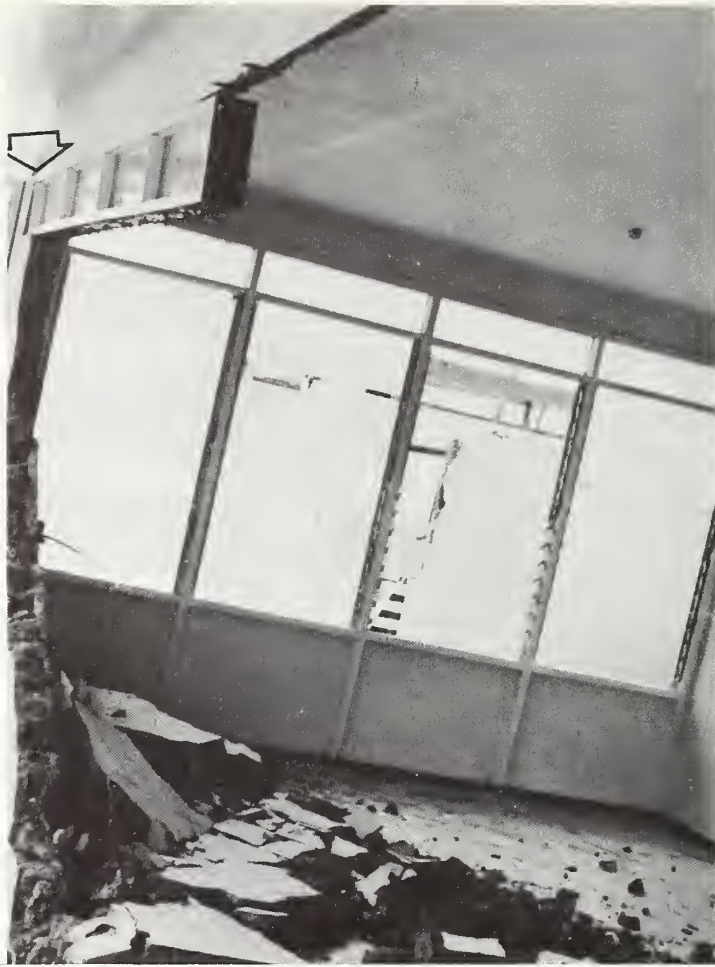
Figure 24 Wall damage resulting from Typhoon Yoling, November 1970
