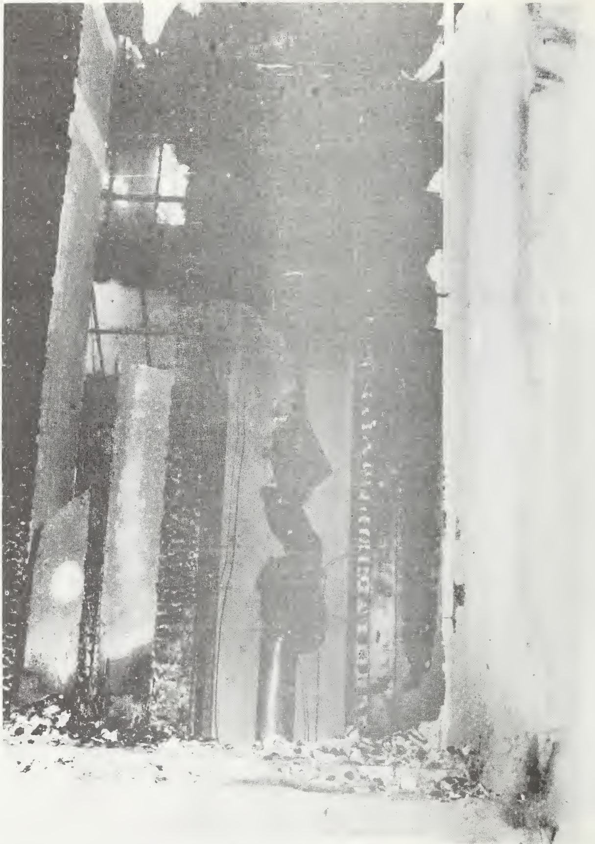
Fig. 38 Chamber 5 after Test 2.
