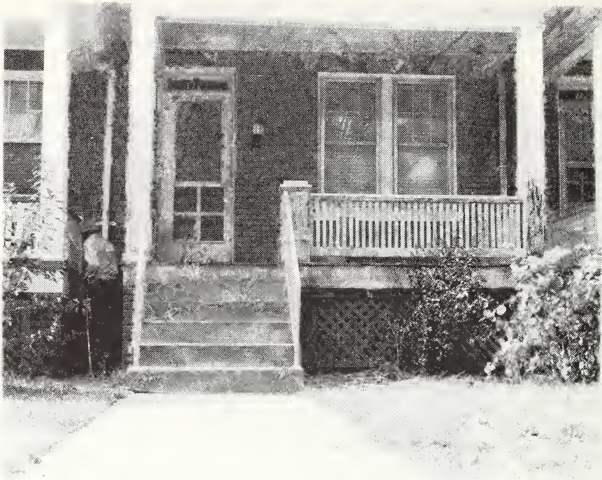
Figure 1. Front porch of pilot demonstration dwelling unit at the start of the paint removal process.
