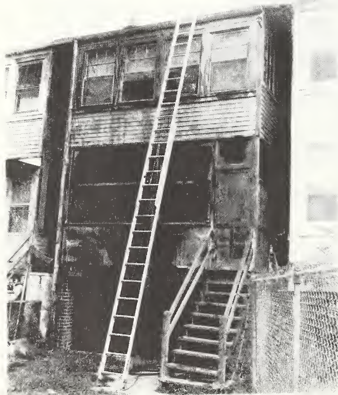
Figure 8. Appearance of paint on wood siding and trim on first floor and basement areas and on metal siding below second floor windows after 30 minutes dwell time of paint remover.
