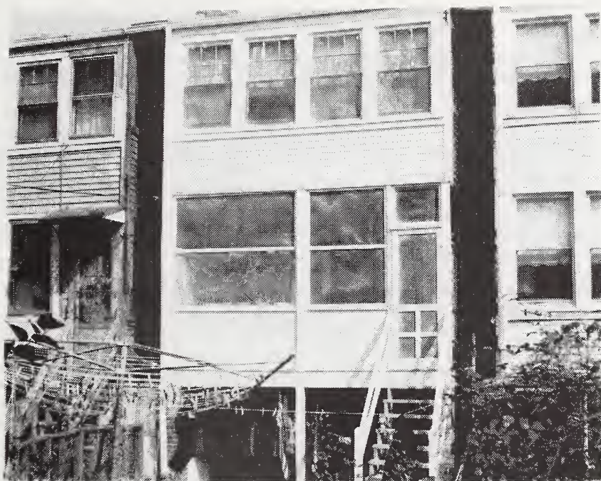
Figure 16. Back screened porch, enclosed second floor porch and basement area way of pilot demonstration after removal of old paint and repainting.
