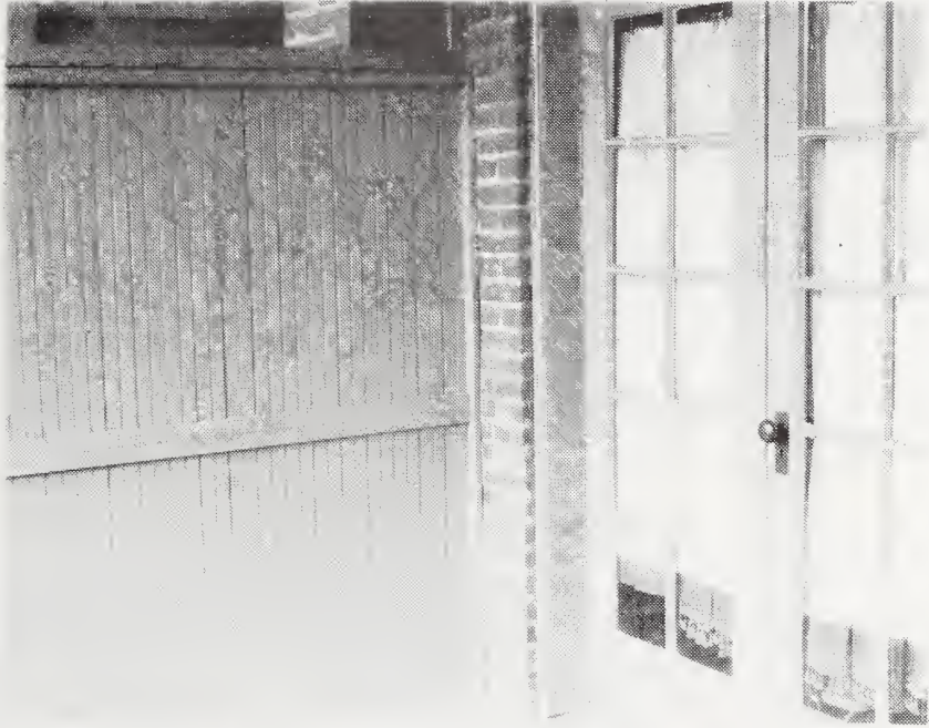
Figure 3. Interior wall and door of back screened porch before removal of paint.
