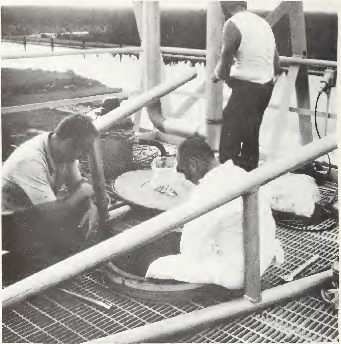
Figure 3. LOX tank outer manhole access.
