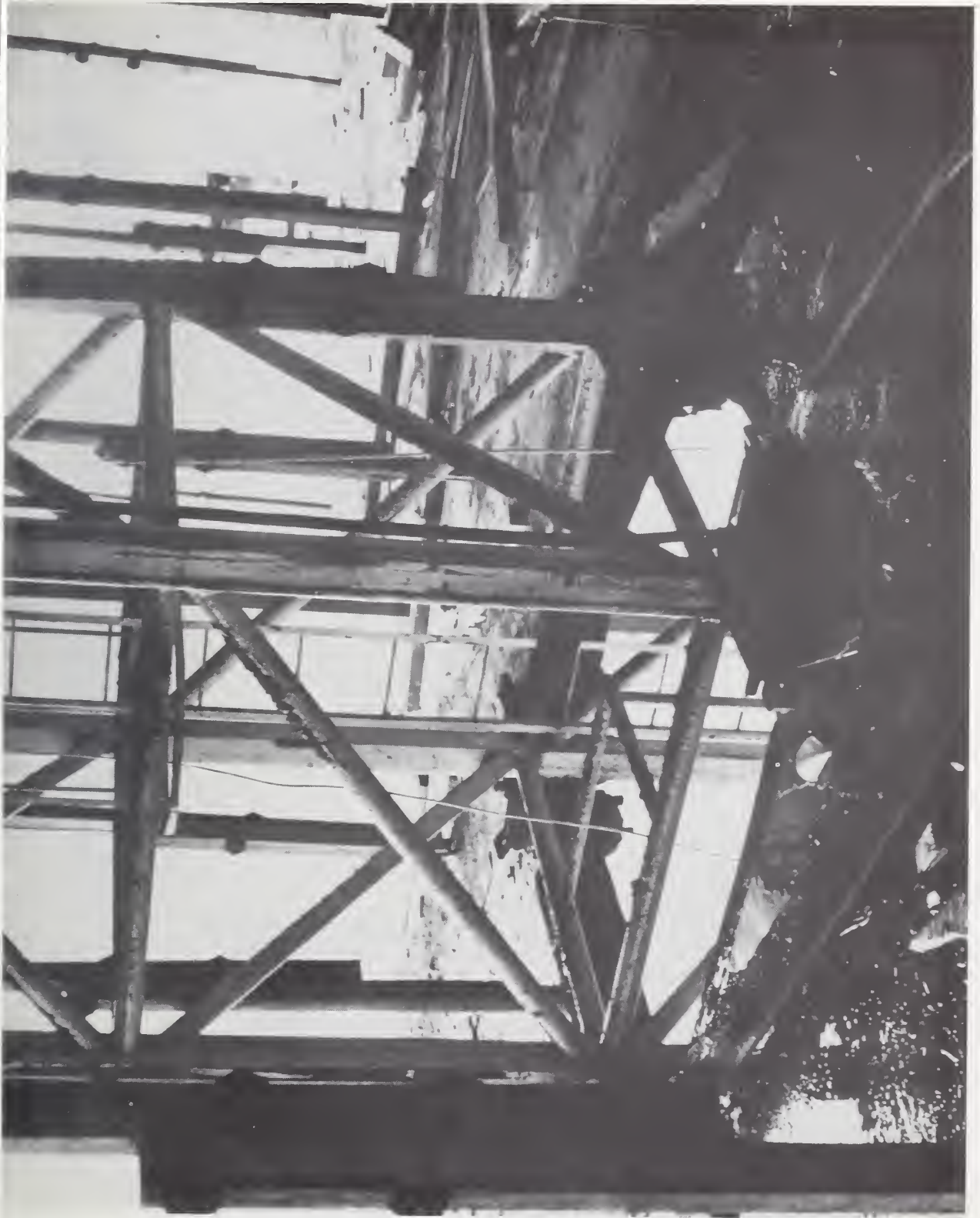
Figure 2.34 Upper support for crane no. 1.
