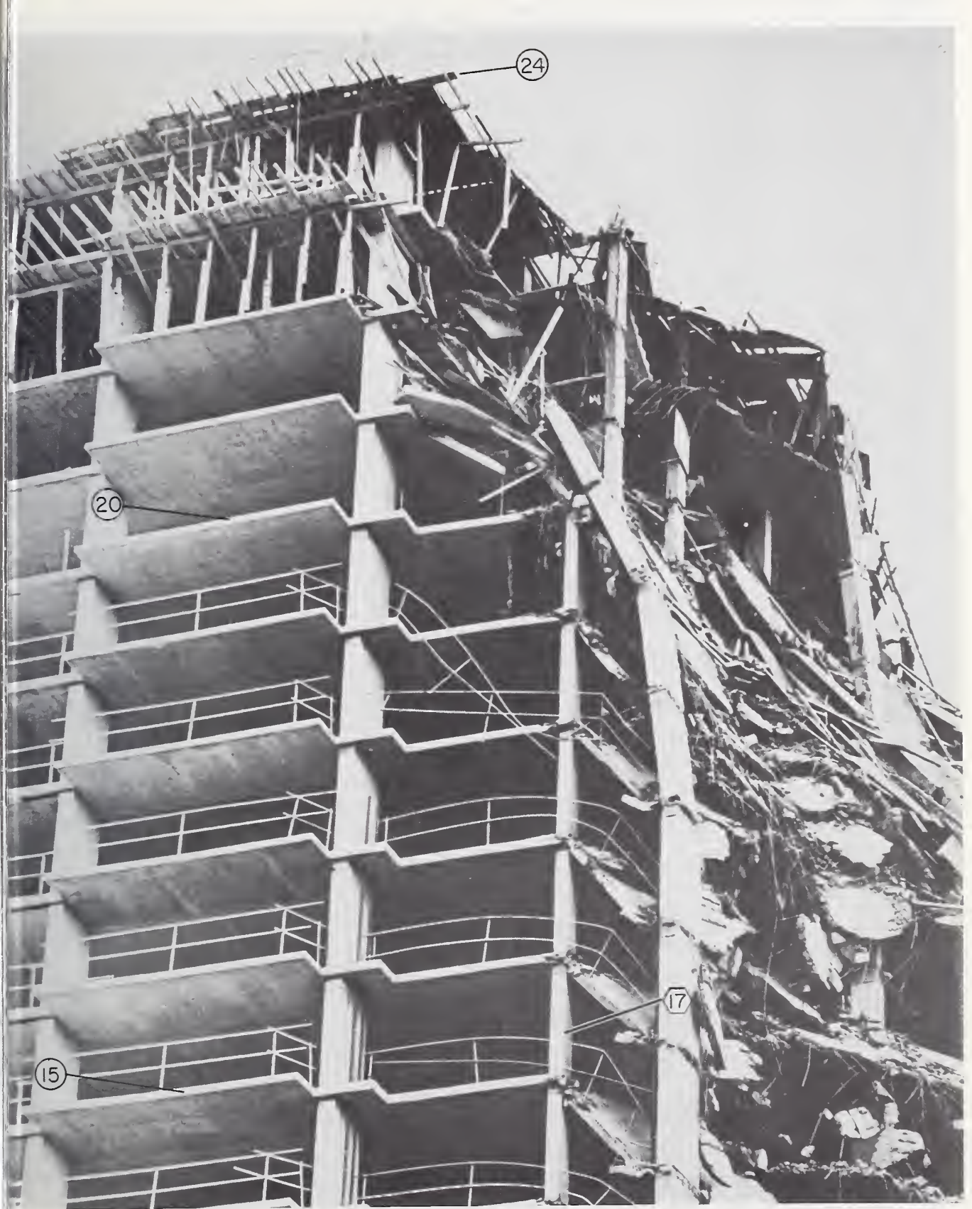
Figure 2.6 Closeup view of the top of the east end of the failure zone, looking south.
