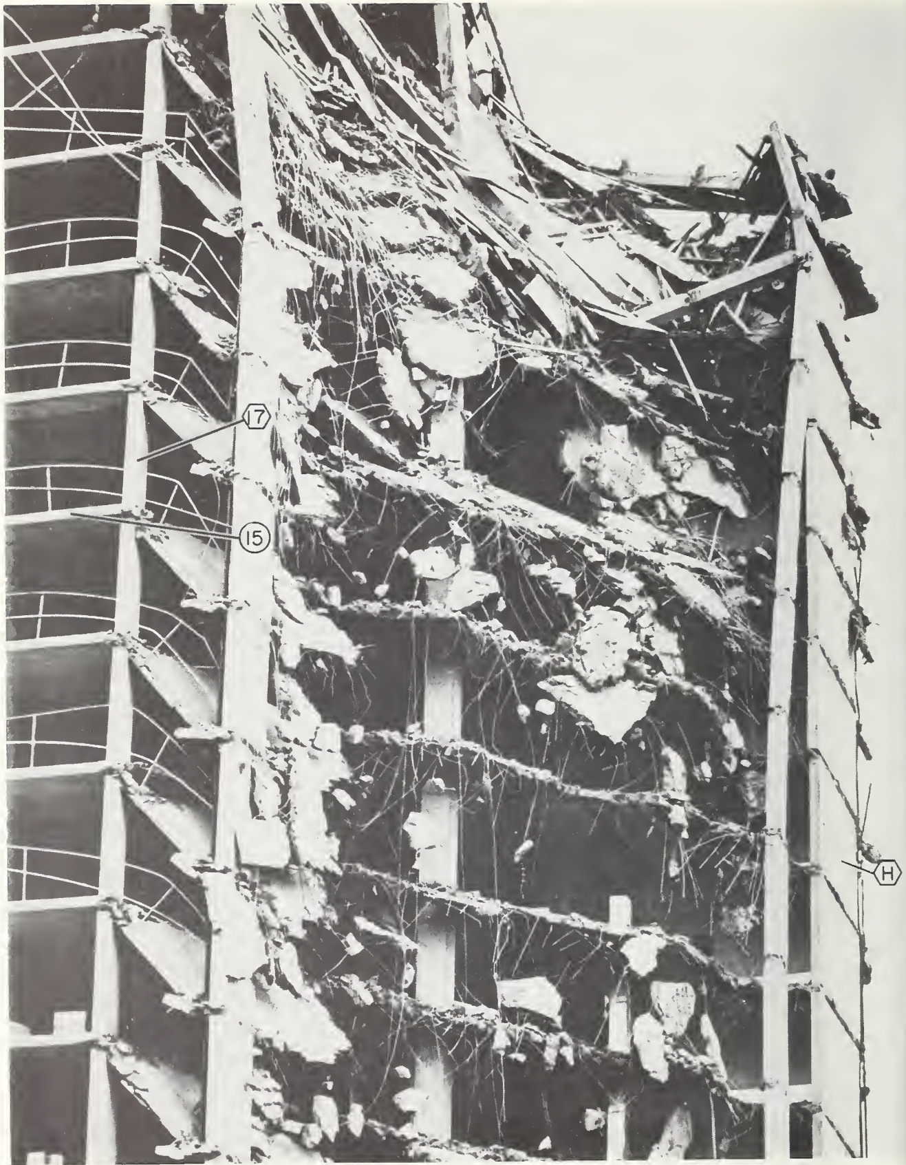
Figure 2.7 Closeup view near the top of the east end of the failure zone, looking south.
