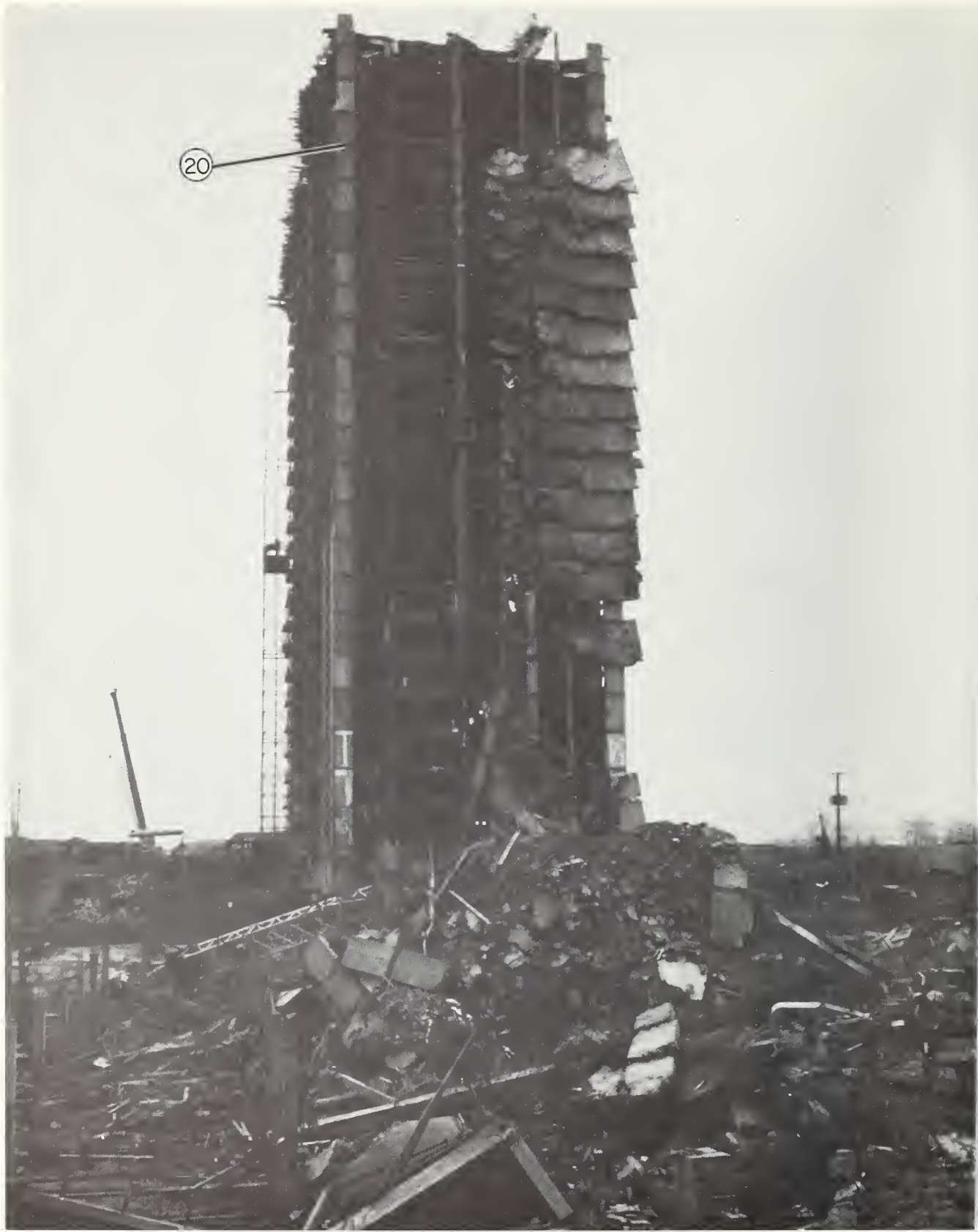
Figure 2.13 Appearance of A-4 after the removal of the east end of the building, viewed from the east.
