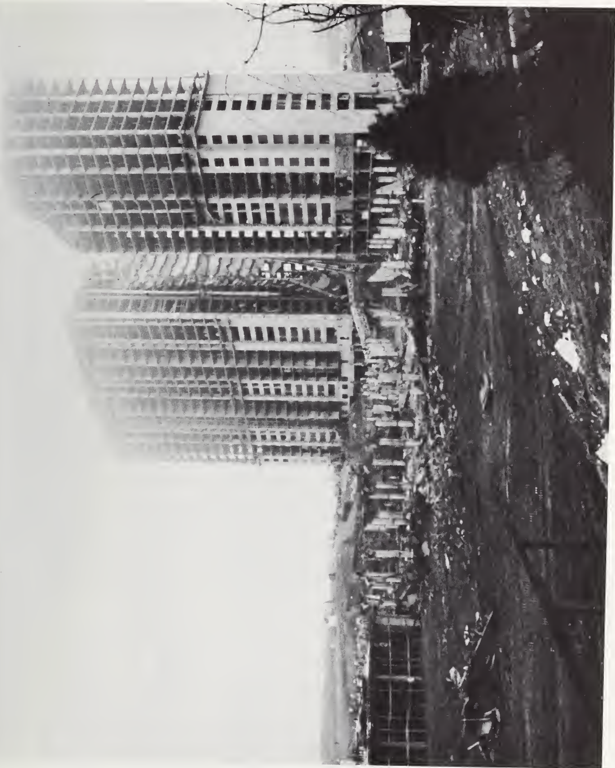
Figure 1.3 Appearance of the collapsed structures as viewed from the southeast.
