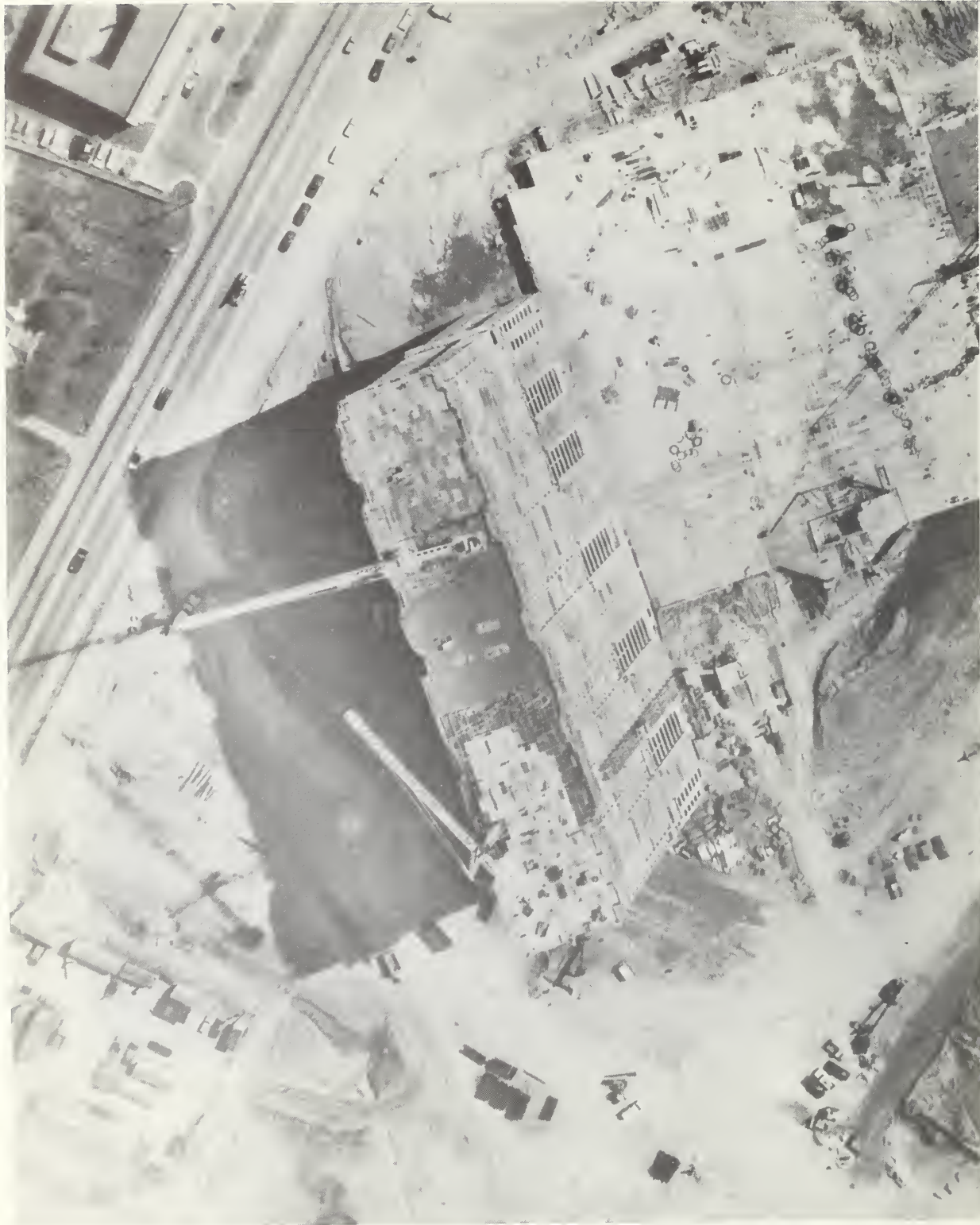
Figure 1.2 Aerial view of construction at 11:00 a.m., March 2, 1973 (north is to the top).
