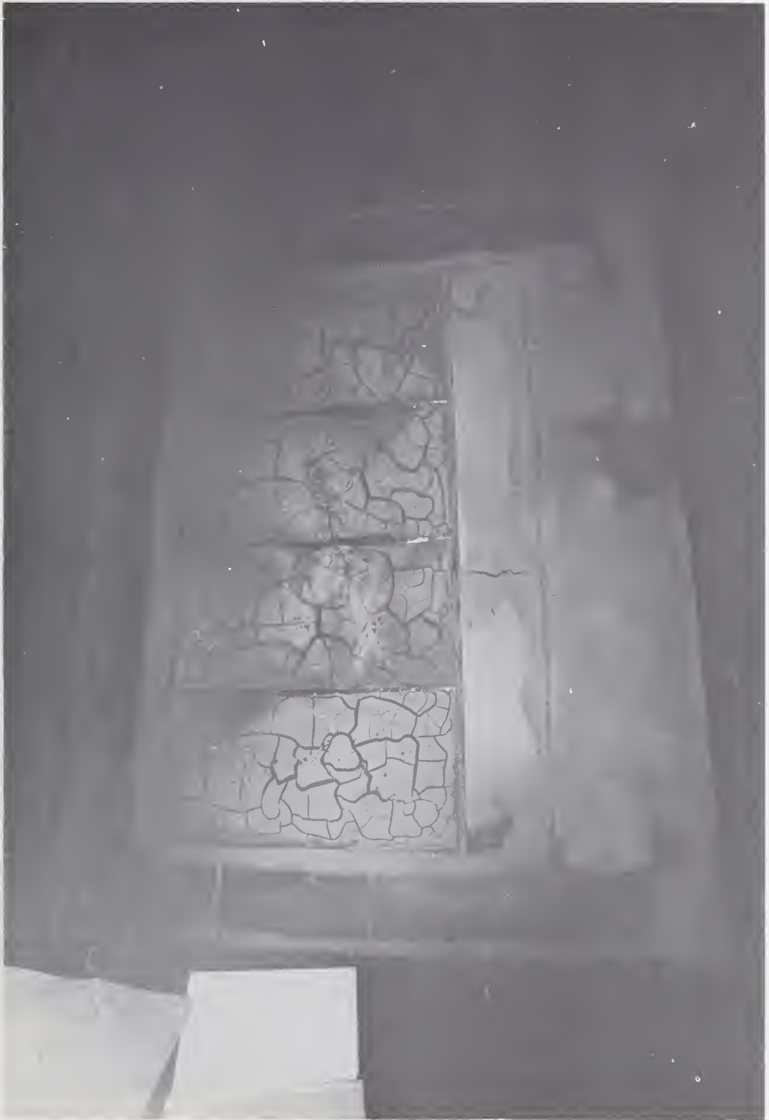
Figure 17. The fire side of the wall panel after it was removed from the surface just before extinguishment of the fire.
