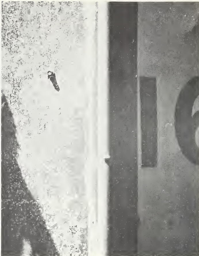
Fig. 26 - Corrosion of metal substrate where applied coating has been lost from panel (Puerto Rico). (C.2)
