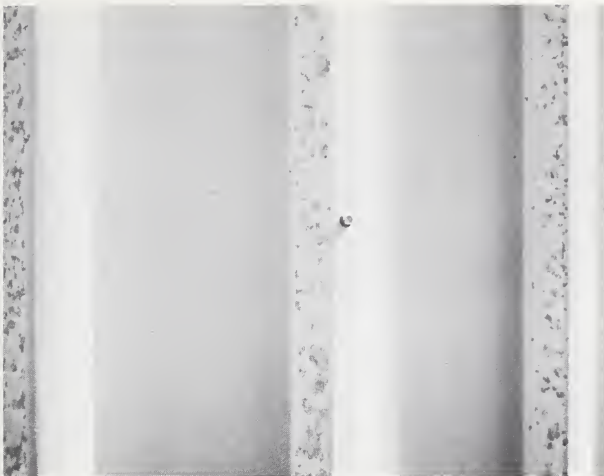
Fig. 34 - Close-up photograph of cladding damage pictured in figure 33, showing substrate exposed by hail impact. (C.2)
