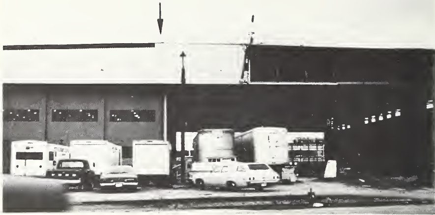
Fig. 30 - New cladding (to the right of the arrow), of same color as original cladding, being added to airplane hanger. (C.2)
