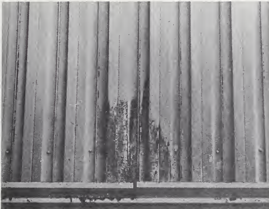
Fig. 28 - Cladding over a heat exchanger exhaust. (C.2)
