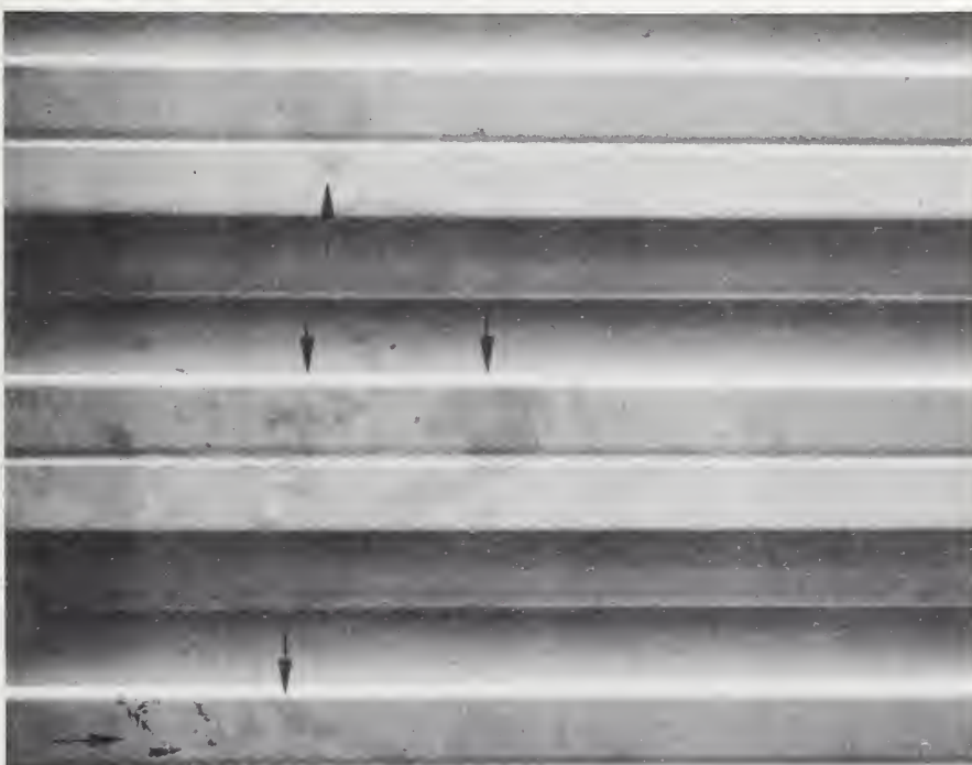
Fig. 29 - Cladding after 5 years near salt water, showing chalking (vertical arrows) and abrasion (horizontal arrow) of the applied coating. (C.2)
