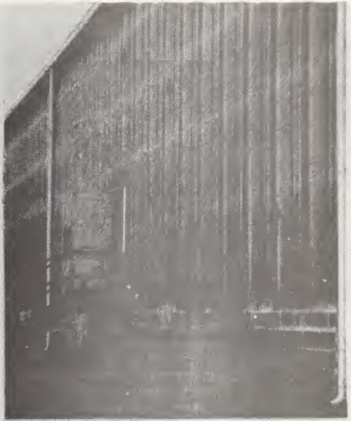
Fig. 32 - Building wall of industrial cladding with arrows indicating color fade of the applied coating. (C.2)
