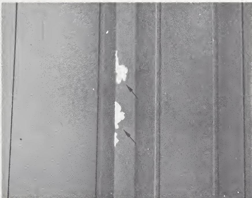
Fig. 35 - Spalling of applied coating (indicated by arrows) due to alleged improper preparation of substrate during factory coating. (E.2)
