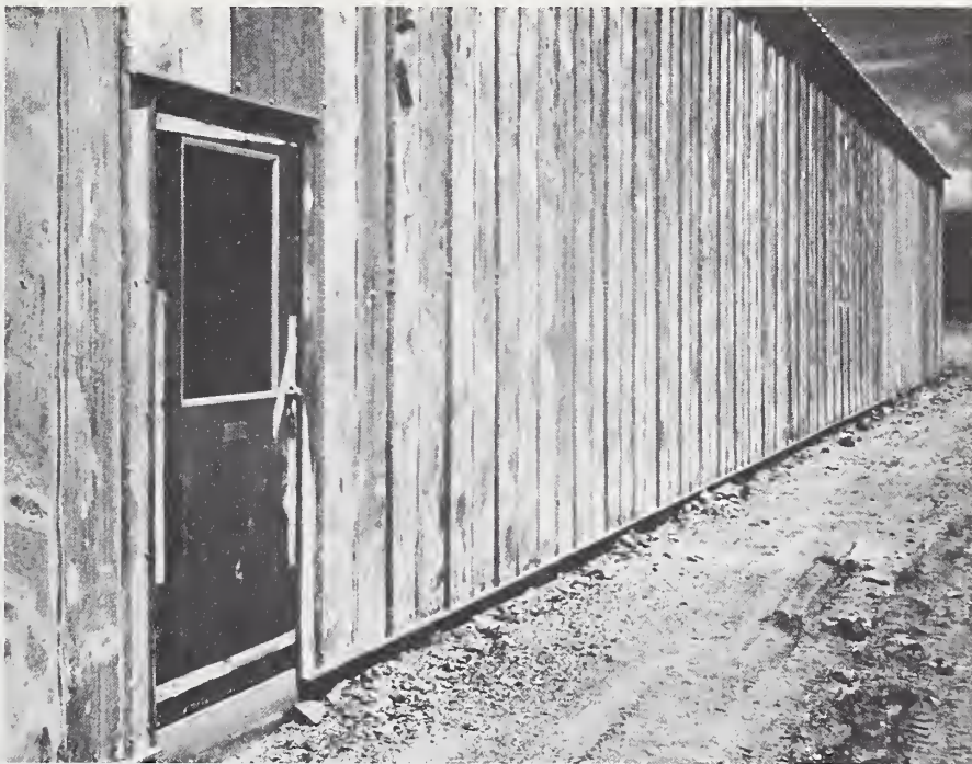
Fig. 25 - Building in Puerto Rico, constructed of non-coated metal cladding. (C.2)
