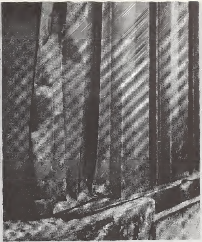
Fig. 38 - Damaged cladding next to loading dock. (E.2)
