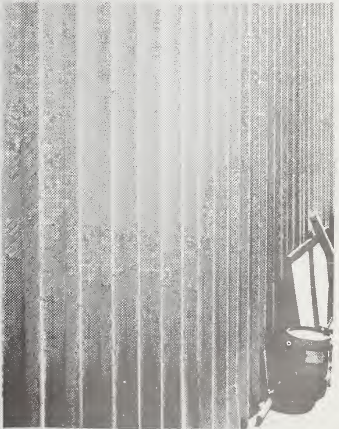
Fig. 33 - Industrial cladding damaged by hail. (C.2)
