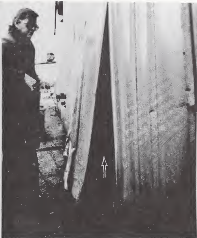
Fig. 40 - Wall panels pushed-out from inside building. Arrow indicates prongs of forklift truck. (E-2)
