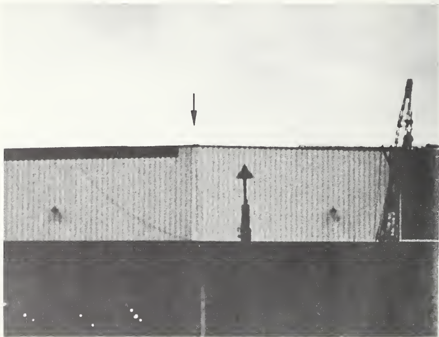
Fig. 31 - Enlargement of figure 30. Color of original cladding (left of arrow) is faded when compared to the identical color in the new cladding (right of arrow). (C.2)
