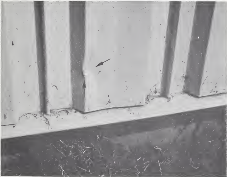
Fig. 37 - Deformation of wall panels (indicated by arrows) from grass cutting machinery. (E.2)
