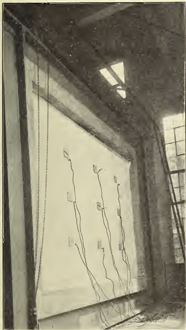
Partition in place for test forms one side of the furnace chamber
