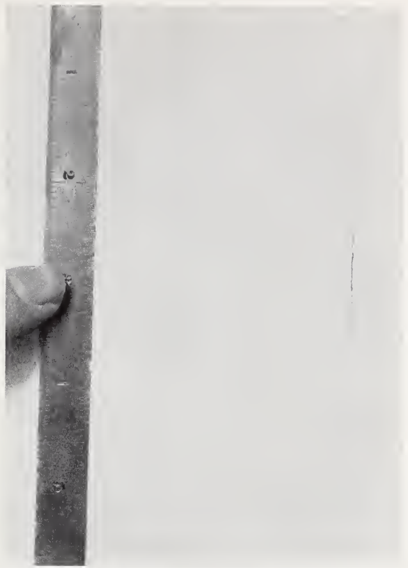
FIGURE 3.—Unightly cracks at joints between fiberboards nailed to studs.
