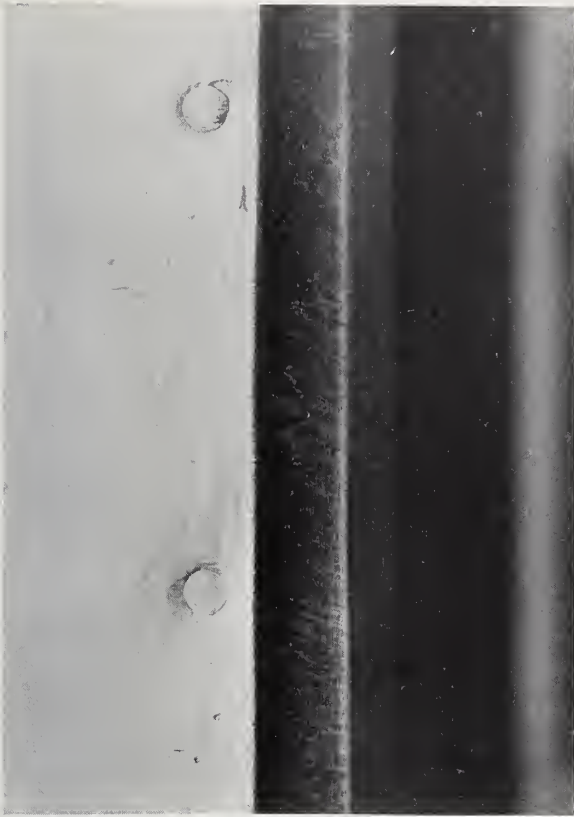
FIGURE 2.—Distortion at nail heads on fiberboards nailed to studs.
