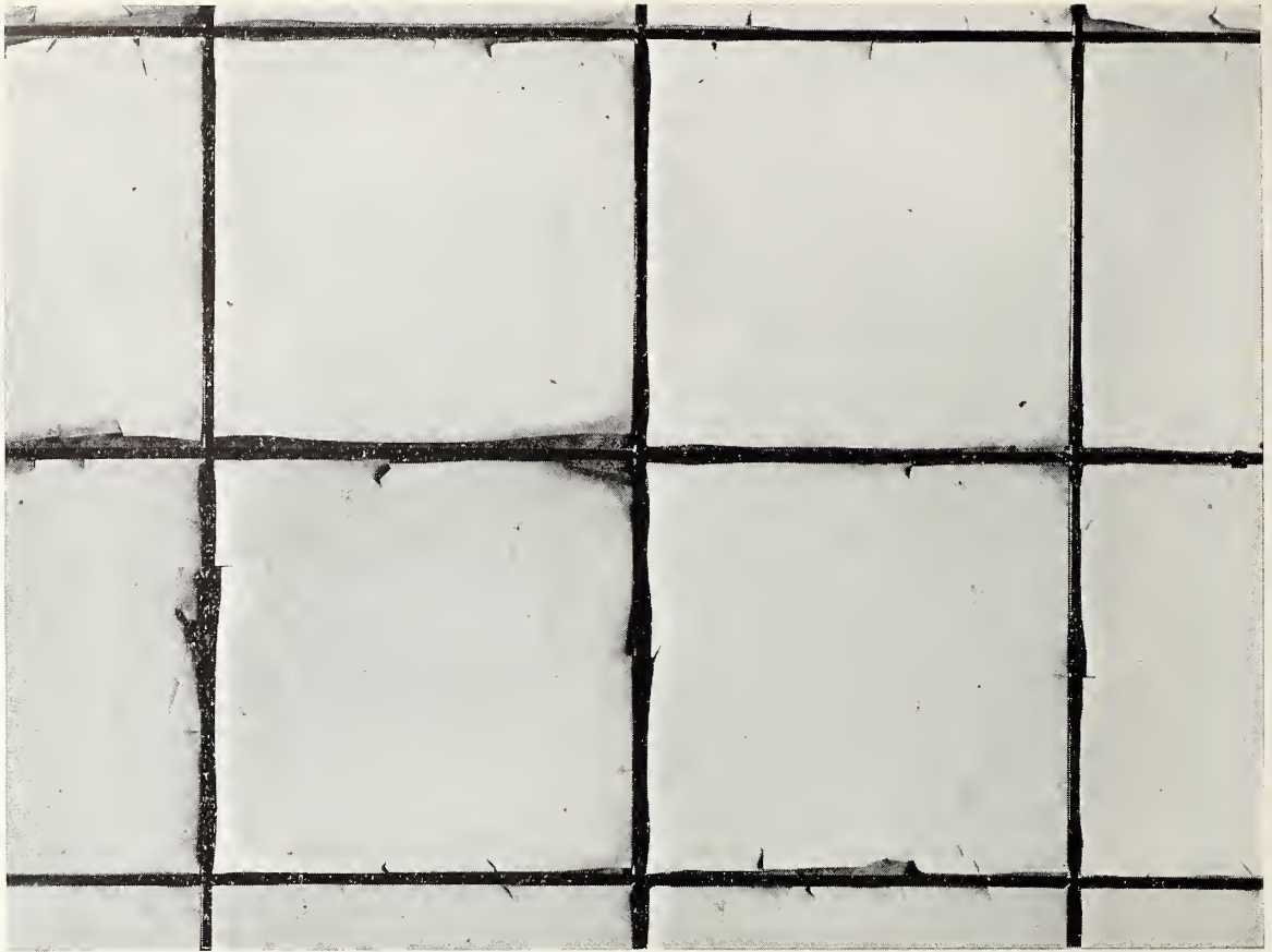
FIGURE 5.— Loosening of surface coat due to failure of bond between surface coat and base material when steamed.
