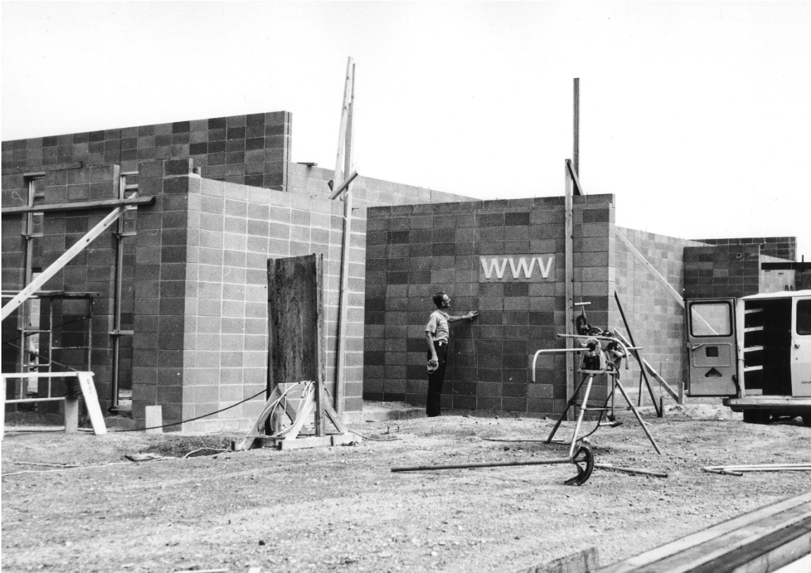
Fig. 18. WWV building under construction in Colorado, 1966. The call letters on the wall were the only parts transferred from the Greenbelt, Maryland, location.
